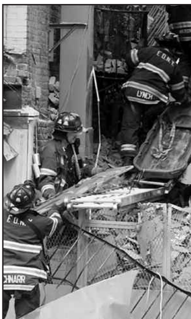
FF Christopher Lynch operates at Manhattan crane collapse in 2008.
