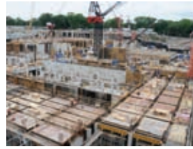
Croton Water Filtration Plant
