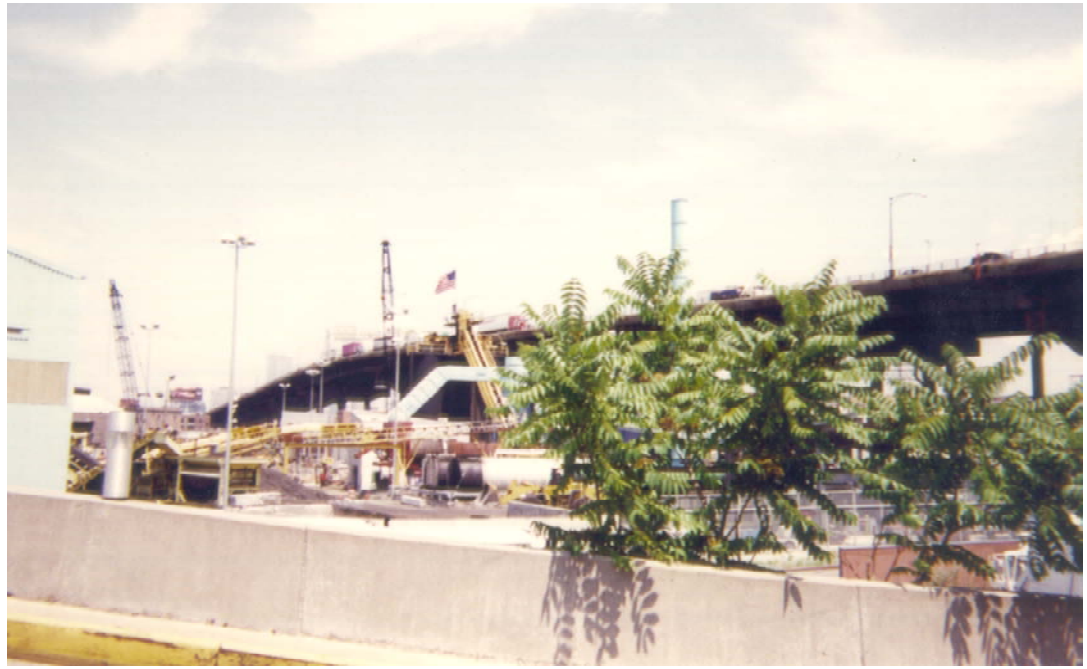
Figure 7.7-5 : View of DOT property, looking northward from interior of the site. (Photo 2000)
