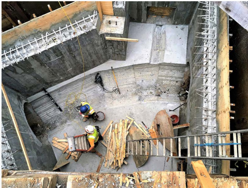
Wood forms being removed from a new concrete storm sewer chamber on Lucas Street between Nashville Boulevard and 122 nd Avenue (October 2017)
