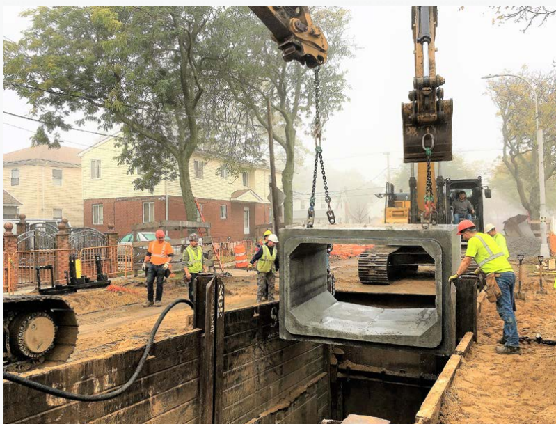
A section of large concrete sewer is lowered into place on Lucas Street between Nashville Boulevard and Williamson Avenue (November 2017)
