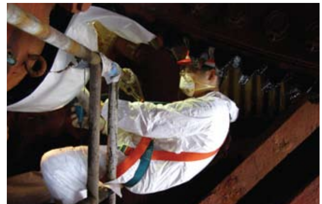
Installing strain gauges on a movable bridge — Pulaski Bridge over Newtown Creek
