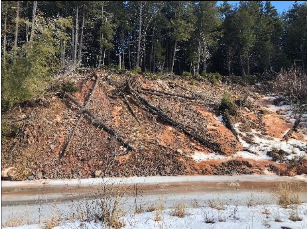
Figure 3. Example of freeze/thaw induced turbid discharge from the hillslope.
