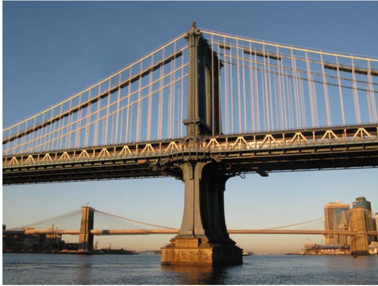
Work Platforms for Cable Rewrapping on Cable C of the Manhattan Bridge and Painting Containment and Shielding on the Brooklyn Bridge in August 2010. (Credit: Bojidar Yanev)
