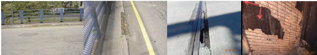
Spalled Section of Curb on the East 8 th Street Bridge in 2006. (Credit: NYSDOT) Spalling With Exposed Rebar on the Beginning Abutment Joint Header of the Westchester Avenue Bridge over the Bronx River in 2011. Underdeck Spalling With Exposed Rebar on the Concourse Village Avenue Bridge over Metro North in 2012.
