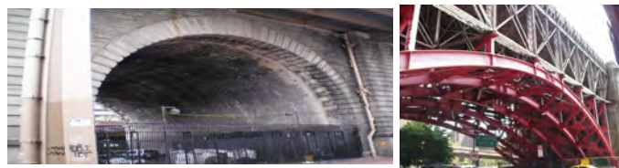
Manhattan Approach: Arch Blocks C, B, and A, Cliff Street Arch, and Franklin Square Structure.
