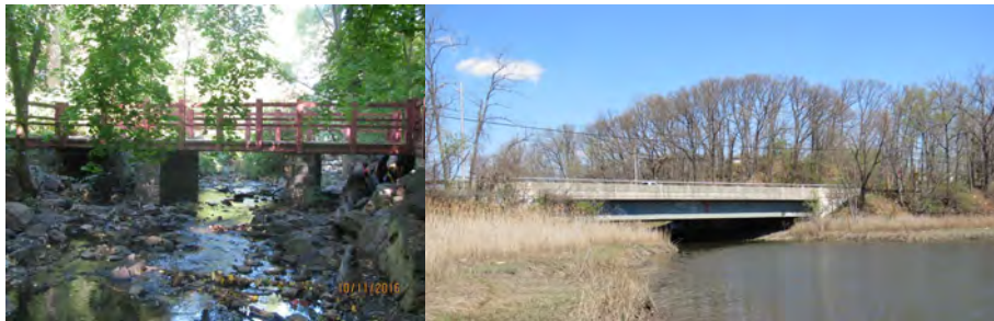
Footbridge South of Forest Avenue over Stream in Park. Hylan Boulevard Bridge over Lemon Creek.
