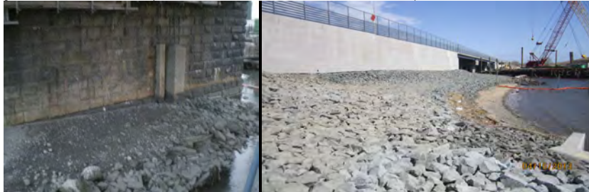
Eroded Riprap Pier Protection at Pier 11 of Old Willis Avenue Bridge in 2008. (Credit: NYSDOT) Riprap Installed in 2013 on South Side of Belt Parkway Bridge over Fresh Creek, Facing East.
