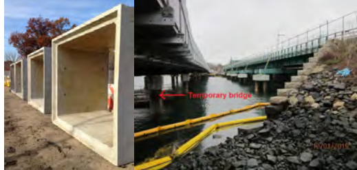
July 2015: Installing Decking for Span 15. November 2015: New Culvert Boxes to Replace the Aging Conduit that Connects the Bay with Turtle Cove, Located Beneath City Island Road. December 2015: Temporary Bridge at Left. (Temporary Bridge Credit: NYSDOT)
