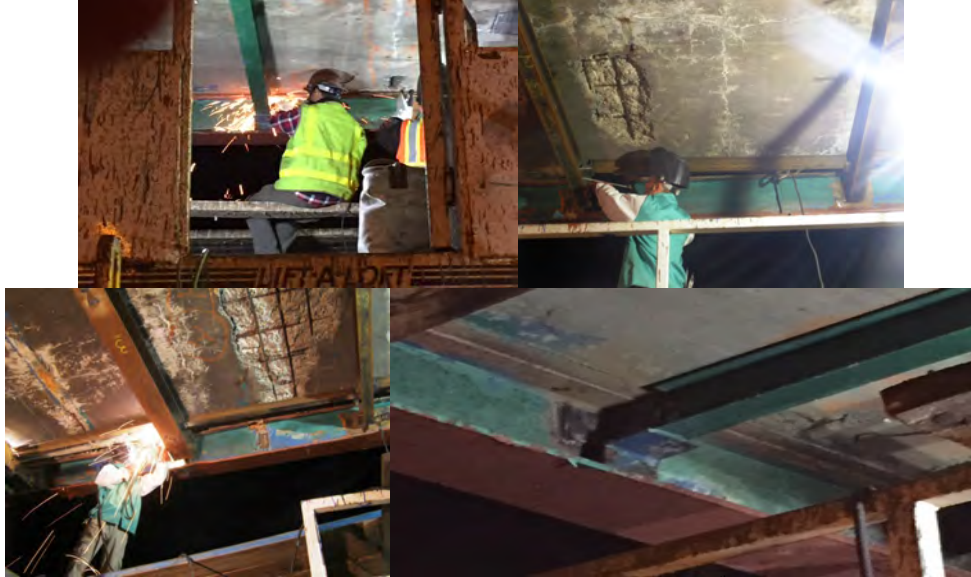
November 2016: Ironworkers Repairing a Diaphragm Connection on the East 128 th Street Pedestrian Bridge After a Recent Truck Strike.
