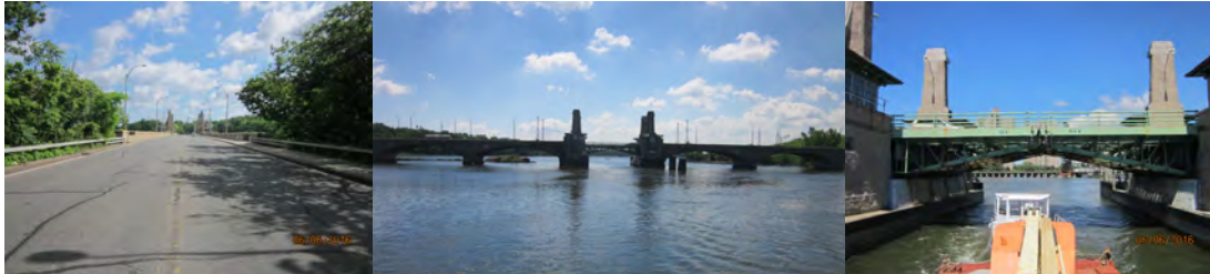
2016: Beginning Approach. Left Elevations Spans 4 – 7. Right Elevation Spans 1-5. Left Elevation Span#4. (Credit: NYSDOT)
