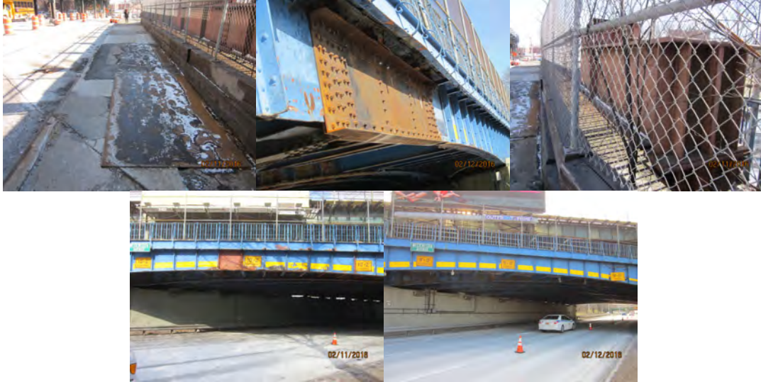
2016: Span 1 Right Sidewalk Near Beginning Abutment – Steel Plates. Girder Reinforced With New Steel Plate and Angles. Strongback Girder at Right Side of Span 1. Right and Left Fascia. (Credit: NYSDOT)
