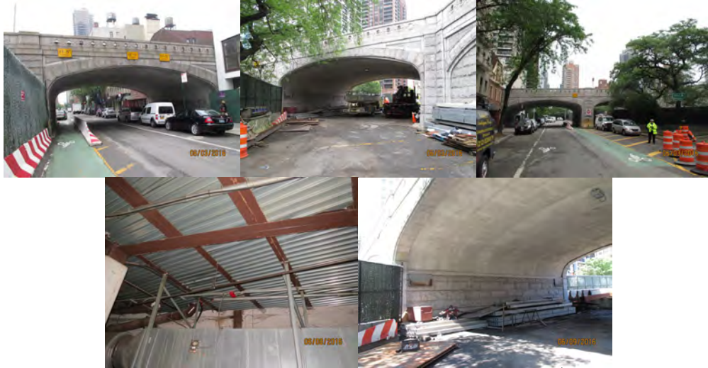
Ramp to the Ed Koch – Queensboro Bridge from East 58 th Street over East 59 th Street. June 2016: Westbound Span 11 Vertical Clearance Signs. Span 10 – Left Elevation. Spans 10 and 11 – Left and Right Elevations Span 8, Underside of Deck at Bay 2. Steel Stay-in-Place forms Installed as Shielding. Pier 11. (Credit: NYSDOT)
