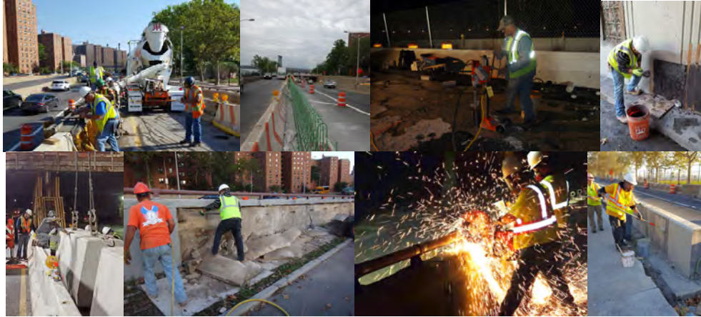
June 2016: Concrete Placement for West Barrier Wall at Entrance Ramp. Rebar for West Barrier Wall. Core Drilling Lift Holes for Stage 2 Deck Removal. October 2016.
