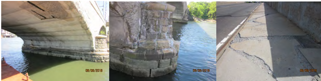
2016: Pier 1 Begin Face. Pier 2, Left End of Pier Nose - Typical Mortar Loss Between Stones. Span 6 Right Sidewalk Exhibits Full Width Shallow Spalls. (Credit: NYSDOT)
