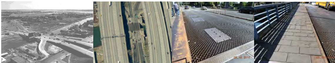
Unionport Bridge in 1953 and 2009. 2015: Span #9, Open Deck Grating at Westbound Roadway, Looking Ahead and Right. Loose and Bouncing Plates. Plastic Delineator Posts Mounted to the Concrete Median are Missing the Majority of Posts Due to Vehicular Impacts. Span #9 Right Sidewalk, Looking Back. Asphalt Tiles Over the Bascule Span are Severely Deteriorated and Exhibit Several Missing Tiles. (Credit: NYSDOT)
