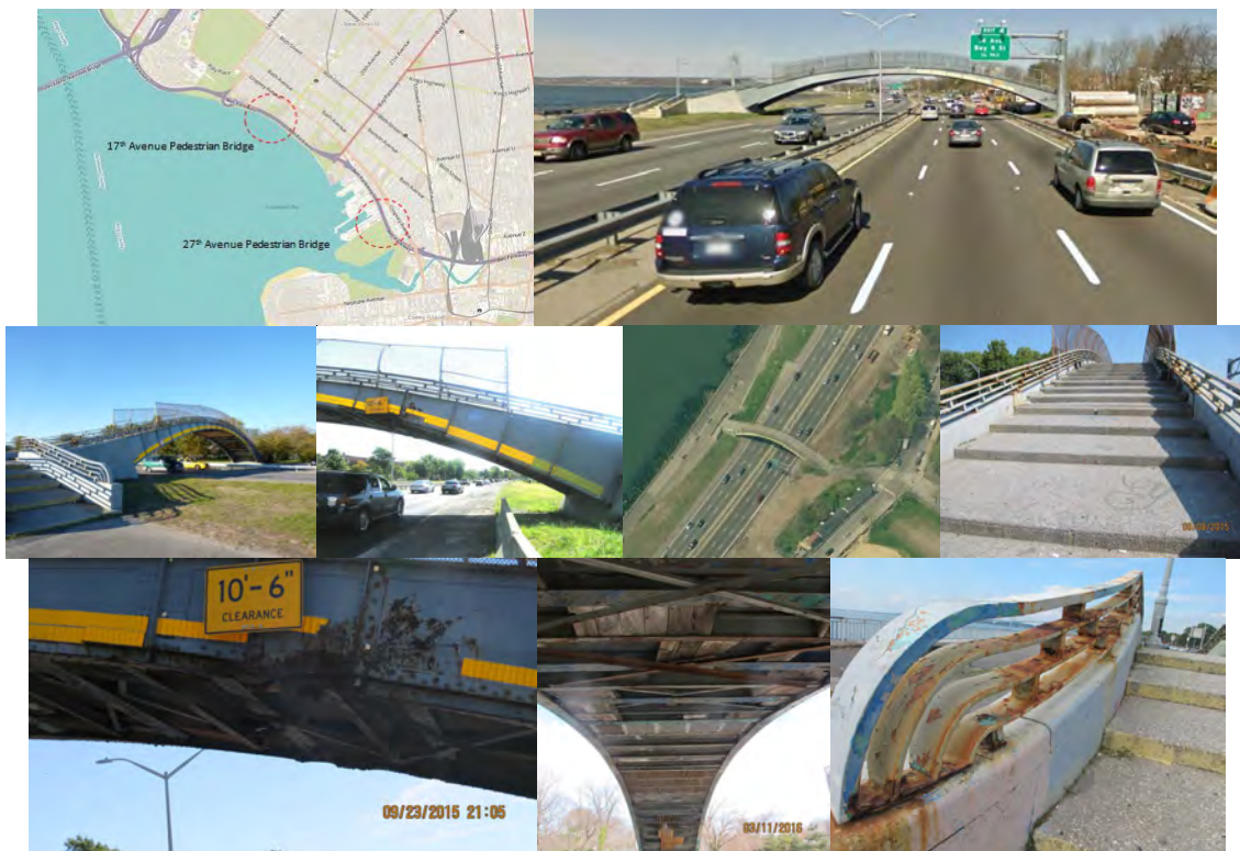
Location Map. 17 th Avenue Bridge – Existing Conditions. Deteriorated Left Girder. Top of Span 1, Looking North – Wearing Surface has Extensive Scaling with Exposed Aggregates. Span 1 Left Girder over Belt Pkwy Eastbound Left Lane was Struck in September 2015. March 2016: New Bracing Under Span 1. October 2016: Beginning Approach, Left Side – Extensive Corrosion on the Guide Railing.
