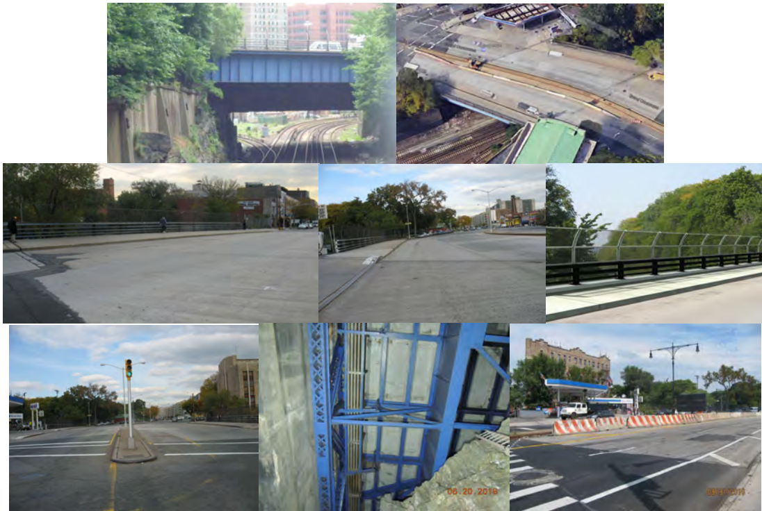
Grand Concourse Bridge over Metro North in 2010. (Credit: NYSDOT) Aerial View. East and West Sides of the Bridge. Proposed Fence and Bridge Railing. Top of Bridge. June 2016: Roadway Deck Underside of Span 1, Transverse Cracks With Efflorescence and Hollow Sections. (Credit: NYSDOT) August 2016: Jersey Barriers on Beginning Approach.
