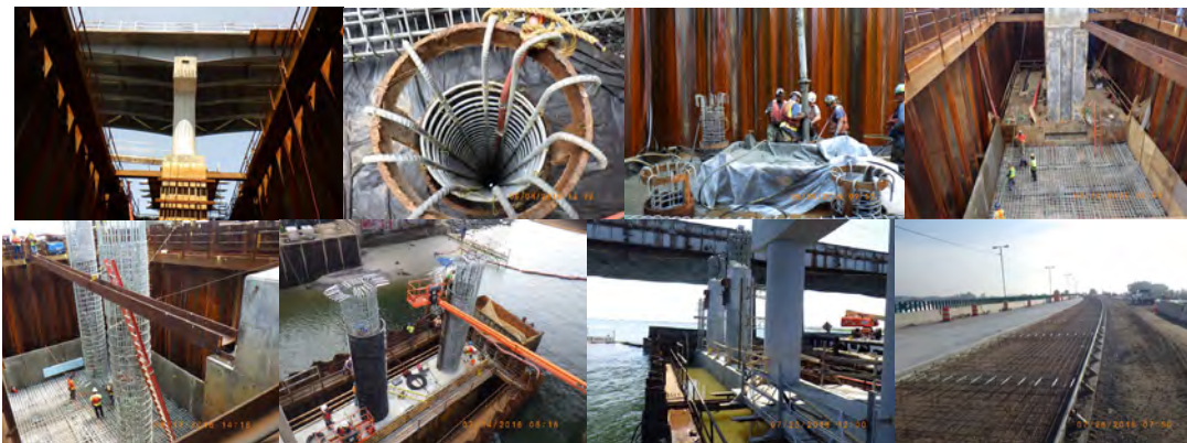
Gerritsen Inlet May 2016: Cofferdam at Pier at Pier #2. Column, Pier Cap and Structural Steel Placed in Stage 1. June 2016: Rebar Cage Placed Inside Steel Pipe Pile Prior to Concrete Operation. Filling Steel Pipe Piles With Pumped Concrete. Pier # 2 Setting Rebar for Footing to Extend Footing Placed During Stage 1. Lowering Column Rebar Cage
