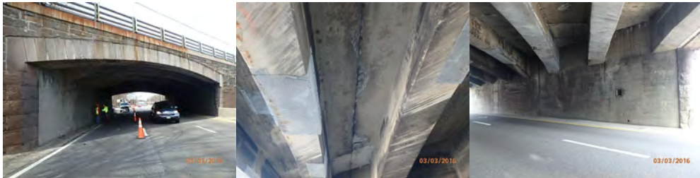
Douglaston Parkway Bridge Southbound Over Cross Island Parkway. March 2016: Right Elevation. Span 1 Concrete Beams Exhibit Spalls With Exposed Rebar Which Are Covered by Wire-Mesh Netting. (Credit: NYSDOT)
