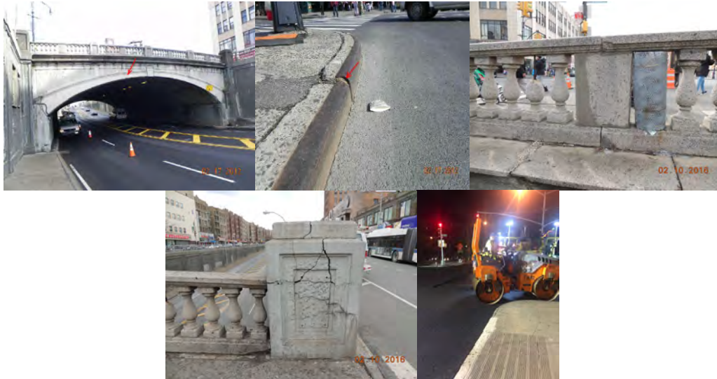
East Fordham Road Bridge over Grand Concourse. February 2016. Span 1, Left Railing Near End Abutment. Railing Balustrade Completely Spalled and Covered With Wire Mesh Netting. Span 1, Left Railing - End Pylon Exhibits Scattered Cracks Throughout. (Credit: NYSDOT) August 2016.
