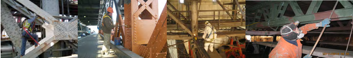
Williamsburg Bridge in June 2010: Application of Finish Coat at North Truss Diagonal. Salt Splash Painting on the Williamsburg Bridge. (Salt Splash Credit: Fouad Althaibani). Inspection of Blasting Surfaces Inside the Franklin Square Arch Containment in September 2010. Brooklyn Bridge Main Span Painting in December 2010.
