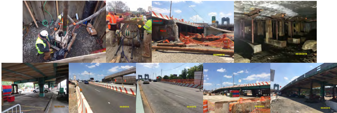
January 2016. February 2016: O-Cell. June 2016: Spans 1 and 2 - View of Removed Portion of Structure. Span 1 Temporary Timber Shoring Under Slab. Span 3 - Timber Planking at Deck Underside. Approach Begin and End. Left Elevation. Right Elevation Spans 3 - 7. (Credit: NYSDOT)
