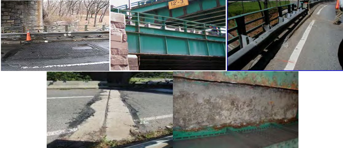
South and North Fascia - Along the Fascias are Built-Up Riveted Steel Girders. The Steel Railing Posts are Welded at the Base to the Top Flange of the Fascia Steel Girders. Deterioration of Joint at Abutment. Underside of Deck with Scaling and Efflorescence.
