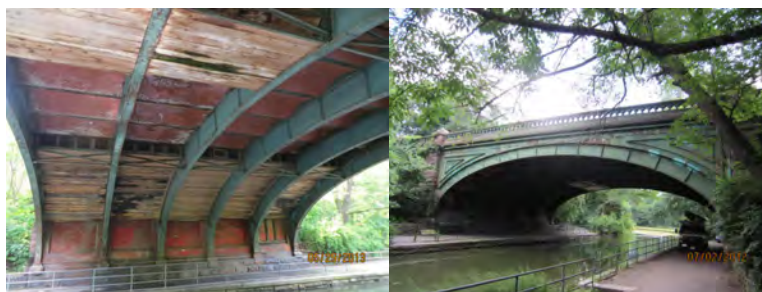
Hill Drive Bridge Span 2 Pier 1 End Face in 2013. View of Bridge in 2012. (Credit: NYSDOT)
