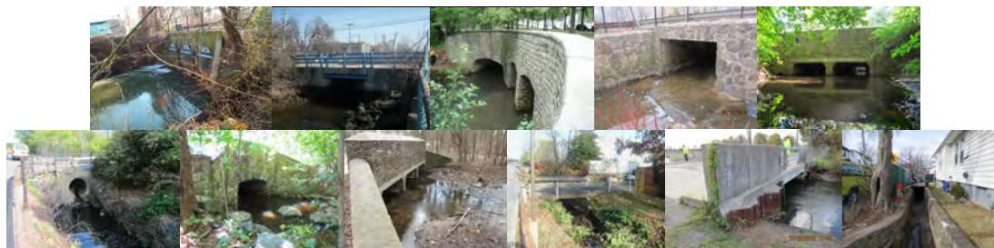
R00013 Naughton Avenue over Patterson Avenue. R00032 Seguine Avenue over Purdy Place. R00115 Victory Boulevard over Cloves Lake Park. R00114 Sweet Brook Road over Ridgewood Road. R00103 Aultman Avenue over St. George Road. R00139 De Pew Place over Maguire Avenue. R00105 Arthur Kill Road over Clarke Avenue. R00101 St. Andrews Road over Lighthouse Avenue. R00040 113 Maguire Avenue over Depew Place. R00059 Western Avenue over RR Bridge. R00005 Bidwell Avenue over Columbus Place.
