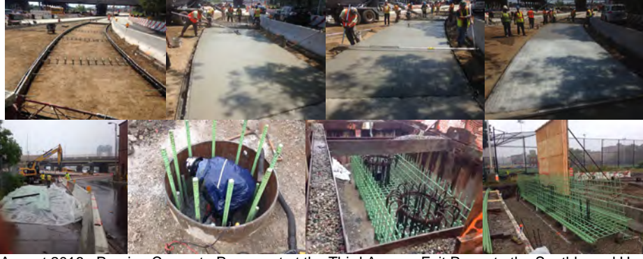
August 2016: Pouring Concrete Pavement at the Third Avenue Exit Ramp to the Southbound Harlem River Drive - The Rails are Used to Create the Proper Super-Elevation on a Curve. A Vibrating Truss Screed is Used to "Smooth" Out the Concrete and Remove any Voids in the Placement. Using a Float to Remove any High or Low Spots, the Pavement Sets Before Final Finishing. Texturing is Added using a Hand Tining Tool. The Finished Product. (Credit: Artemio Angeles) September 2016: North Abutment Pier 8 Foundation. Epoxy Reinforcement Bars to be Installed at South Abutment are Covered. Removing Concrete With a Chipping Gun. Reinforcement for Pile Cap. North Abutment - Reinforcement for the Stem and Forms. (Credit: Artemio Angeles)
