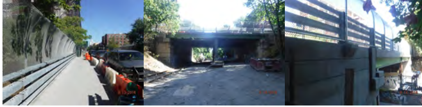
July 2014. September 2015. April 2016. September 2016: New Span 1 and 2 Left Steel Railing and Concrete Sidewalk. Left and Right Elevation. (September Credit: NYSDOT)
