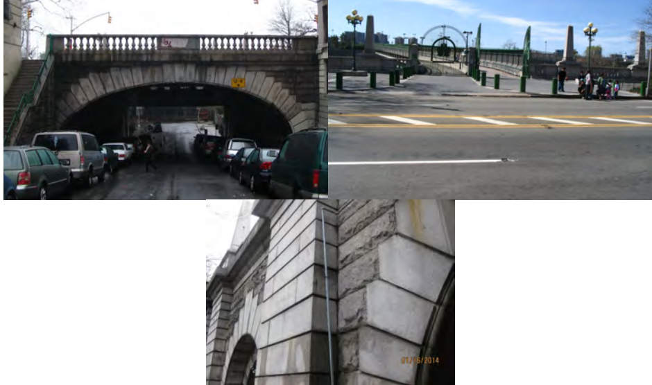
Riverside Drive Bridge over West 138 th Street. January 2014: End Abutment. (Credit: NYSDOT)
