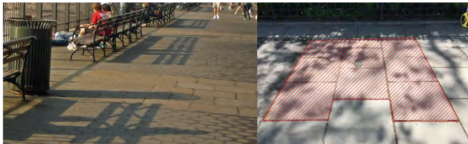
Brooklyn Heights Promenade Pavement - The deck slab of the Brooklyn Heights Promenade is paved with hexagonal pervious pavement interspersed with areas of large rectangular stone pavers. Pavers were removed for testing on the Promenade then replaced once completed. Hands-on inspection of the promenade revealed that the overall condition of the pavement is good, with the exception of a few areas of heaved or sunken pavement, missing pavement, and scaling paver stones. Heaved pavement was observed specifically at the bridge joints.
