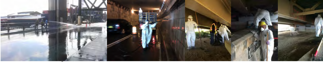
Water Spraying the 9 th Street Bridge over Gowanus Canal in July 2012. July 2013: Power Washing the Battery Park Underpass. (Credit: Earlene Powell) October and December 2015: Highway Repairer Abibi Ocampo Guevara Removing Debris Collected by Vagrants Under the Willis Avenue Bridge.
