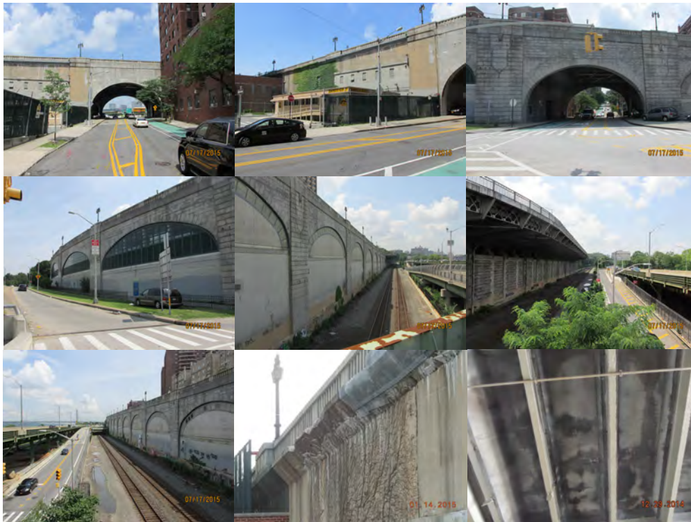
2015: Left Elevation Span 14, Spans 15 – 20. Right Elevation Span 14, Spans 13 – 1, 15 – 77, 41 – 77, and 43 – 13 (Section over NYCDOT Maintenance Garage Area). (Credit: NYSDOT) Spans 19-21, East Fascia Overhang, Looking Southwest - Large Edge Spalls with Numerous Cracks and Heavy Efflorescence Throughout Overhang. Span 52 Looking South - General View of Underside of Deck Showing Extensive Dampness and Cracks with Efflorescence.
