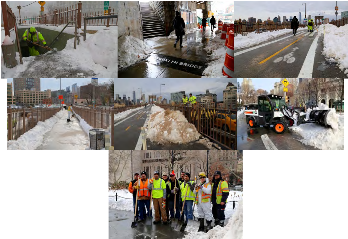
On January 23, 2016, a Record 26.6 Inches of Snow Fell in Central Park, Snow Removal on the Brooklyn Bridge After Storm Jonas in January 2016. Highway Repairer Giovanni Caballero, Bricklayer Stephen Daniel, Cement Mason Stephen Buckley, Cement Mason Mike Biancianiello, Bricklayer Louis Giarratano, Cement Mason Stephen Buckley, Supervisor Bricklayer Edward Alfano, Cement Masons Lawrence Marks and Frank Finizio, Bricklayers Stephen Daniel and Vincent Sciuila, and Cement Mason Victor Porowski.
