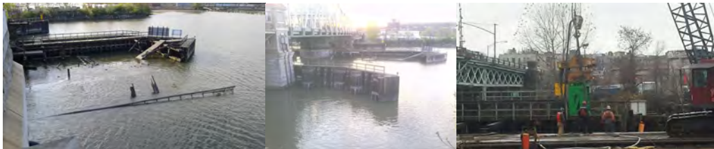
May 2015 – University Heights Collapsed Fender System. Collapsed Fender System in East Channel. December 2015: Loosening the Existing Wooden Pile to Facilitate its Easy Removal From the River (Mud) Bed. The Vibrating Hammer is Attached to the Crane Initially to Vibrate it and Ultimately Loosen the Existing Piles.
