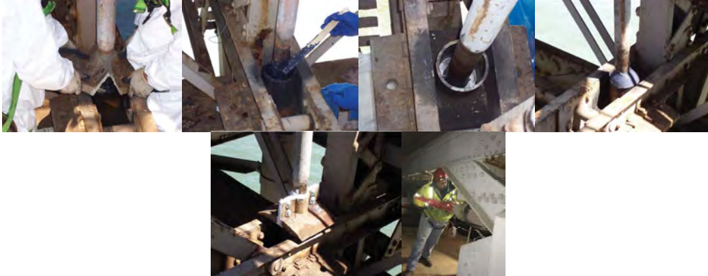
Cleaning and Lubricating the Solid Rods' Suspender Bearings on the Brooklyn Bridge. Oiler Rene Francis on the Madison Avenue Bridge During a Manual Opening of the End Lift Machinery. (Credit: Vera Ovetskaya)
