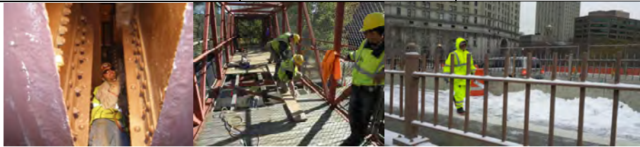
Bridge Repairer Riveter Damian Venezia Squeezing Between the Girders to Access a Floor Beam That Needed to be Reinforced on the Ed Koch Queensboro Bridge – August 2010. (Credit: Hany Soliman) Carpenters John Horgan and Ruben Urena, and Assistant Civil Engineer Fouad Althaibani Repairing the PS-5 Bridge in November 2011. (Credit: Thomas Whitehouse) Cement Mason Victor Porowski Spreading Sodium Acetate on the Walkway of the Brooklyn Bridge in 2013. (Credit: Paul Schwartz).
