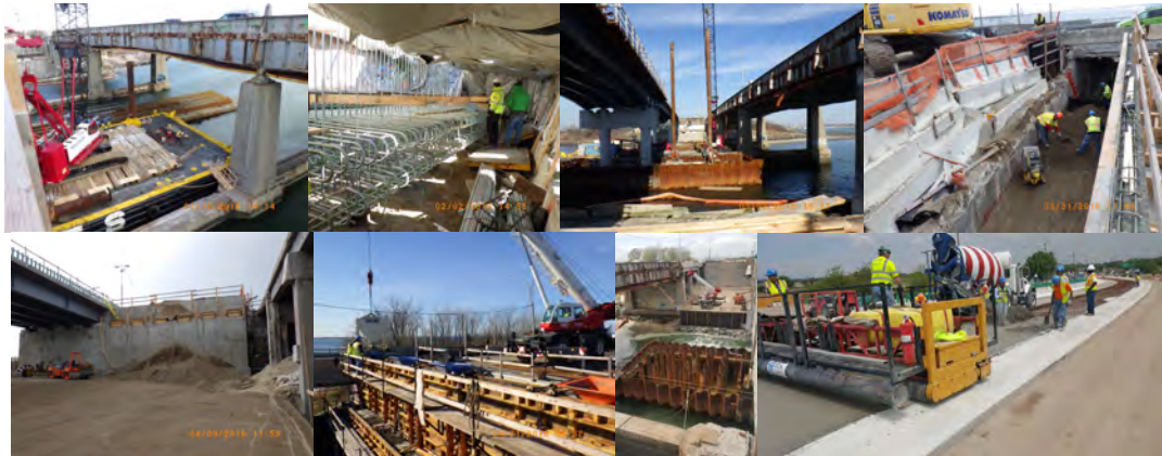
Gerritsen Inlet January 2016: Work Barges Setting up to Drive Steel Shell Piles at Pier #1. Existing Bridge at Right (Partially Demolished) Carrying Eastbound Traffic. February 2016: Galvanized Rebars in Place for East Abutment Footing. March 2016: Driving 24" Diameter Steel Shell Piles at Extension of Pier #1 Cofferdam. New Westbound Bridge at Left. Existing Eastbound Bridge at Right. Backfill Between Old East Abutment of Bridge at Left and New East Abutment Wall for Stage # 2 Bridge Construction. April 2016: Completed Portion of New East Abutment of the Bridge. New Bridge at Left. Placing Concrete at West Abutment Back Wall With a Crane and Bucket. May 2016: Stage 2 Pier #1 Cofferdam With Steel Pipe Piles. Bottom - Existing Footing to be Removed. Top - West Abutment and Existing Eastbound Roadway at Upper Left. Placing and Finishing On-Grade Pavement at Approach.
