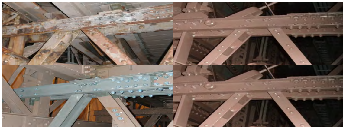
Steel Repair Process: Although Deteriorated Steel is Often Apparent Right Away, Many More Instances are Encountered Only After Removing the Paint. In Some Cases the Location of Deterioration is Painted Along With the Healthy Steel and its Location is Documented for Later Repair. Iron Workers Then Return to Those Locations and Replace the Deteriorated Sections With New Steel. The New Steel is Then Painted Over Again for the Final Protective Coating.
