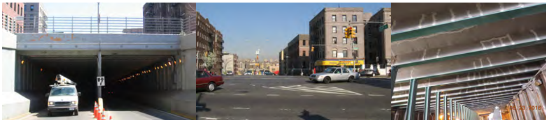
Grand Concourse Bridge over East 167 th Street. June 2016: Span 1, Repaired Underdeck and Girder Concrete Encasement. (Credit: NYSDOT)
