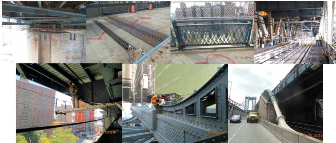
Manhattan Anchorage Maintenance Platform. Looking Northeast at a Trench Drain and Finger Joint on the Parking Deck. First South Rail at South Walkway. 2016: Inspecting the Bridge Using a Rolling Platform, Scaffold, and Sky Climber. (2016 Credit: NYSDOT) Bridge Saddle.
