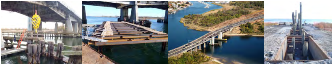
November 2015: Extracting Wood Piles From the Existing Bridge Fender System at New Pier #9 Site. Pier #9 Steel Framing for the Cofferdam on the West Side of the Existing Bridge. December 2015: Outfall #2. Pressure Treated Wood Piles – Facing East.
