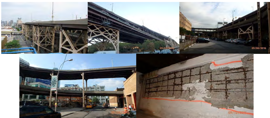
Ramp to 21 st Street From NY Over 22 nd Street. September 2016: Elevation Right Spans 1 to 12, 22 to 36, and 37 to 39. End Abutment Stem Wall – Spalled Concrete With Exposed Rebar. (Credit: NYSDOT)
