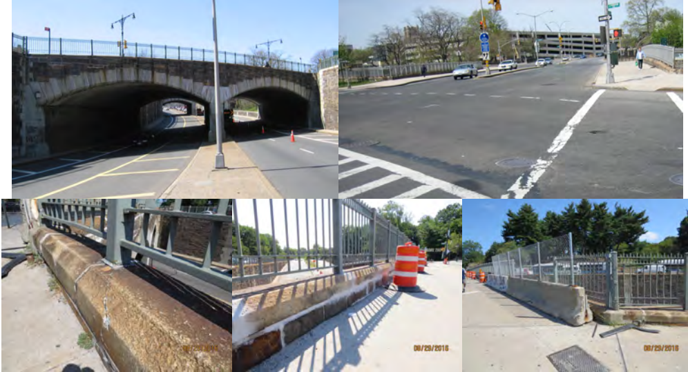
Southern Boulevard Bridge over East Fordham Road. August 2016: Cracked Cap Stone at Right Wingwall. Repaired Joints on Right Parapet. Jersey Barriers and Fence Above the Deck on Span 1.
