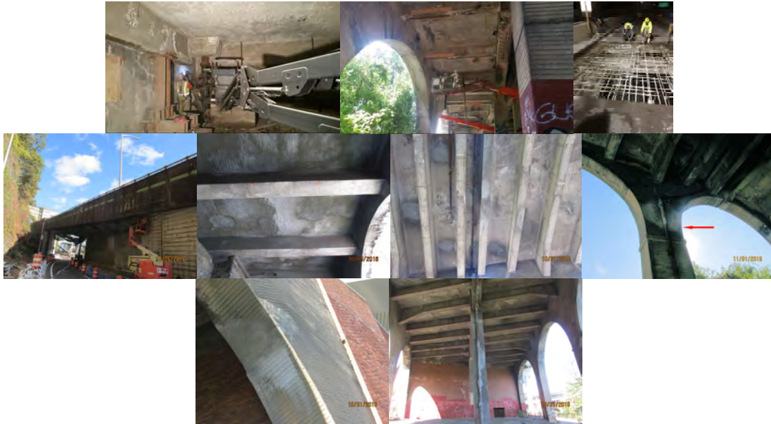
2016: Demolition of Spalled Concrete. Application of Shotcrete. Through Hole Deck Repairs. October 2016: Spans 11-18 Nylon Shielding. Span 27 Deck Repairs. Span 47 Floor Beam Repairs. Pier 43 Right Column Repairs. Span 51, Underside of Right Arch - Concrete Repairs. Pier 49, at Center Column - Concrete Repairs. (Shielding and Repair Credit: NYSDOT)
