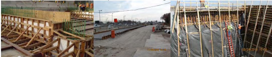
West 252 nd Street Bridge Formwork at the Pier and West Abutment in 2007. Formwork for the Westbound Roadway of the Rockaway Parkway Bridge in 2010. (Rockaway Bridge Credit: Eric Callender) Gerittsen Inlet Bridge in March 2014: Putting up Insulated Forms in Preparation for the Placement of Concrete at the West Abutment Wingwall. The Insulation Helps Protect the Concrete From the Elements and Fluctuating Temperatures During the Curing Period.
