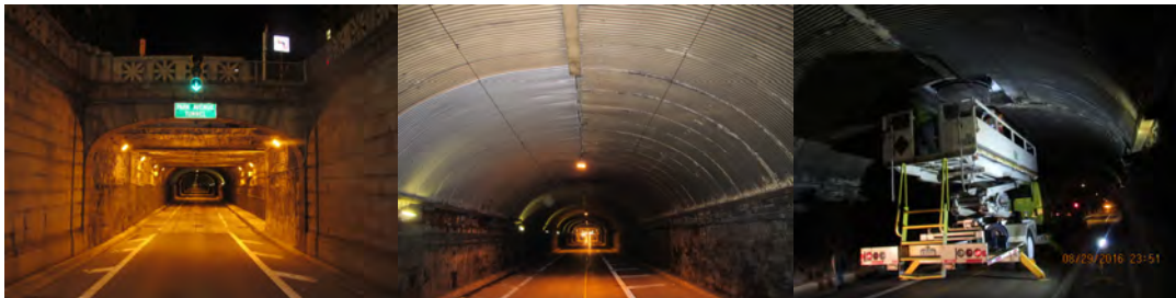
March 2016: 34 th Street Entrance, Looking Northeast. March 2016: Missing Joint Plates at Tunnel Crown. August 2016: Performing Overnight Preventive Maintenance.
