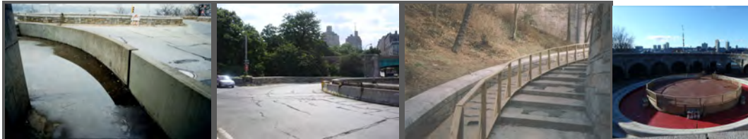
Traffic Circle Level: South Sidewalk Area - Extensive Water Ponding. Pavement - Widespread Cracking. Pedestrian Plaza Level: North Stairway - Timber Delivery Ramp. Closed Fountain.
