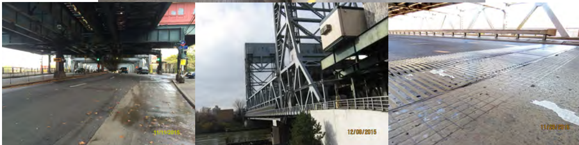
2015: Span 2 Right Sidewalk, Beginning and End Approaches, Framing Span 2. 2016: Pier 1, Finger Joint at Southbound Roadway - Misaligned Fingers. (Credit: NYSDOT)
