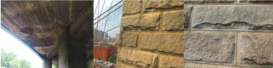
Hollow Sounding And Delaminated Concrete Areas With Exposed Rebars on the Sunrise Highway Bridge Westbound over Laurelton Parkway in 2014. Brooklyn Bridge Tower Stone Delamination in 2016.
