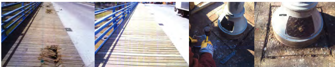
May 2015 Safety Flag: Borden Avenue Bridge Over Dutch Kills - Wooden Planks of Sidewalk Damaged After Vehicle Accident. East 14 th Street Bridge Over LIRR Bay Ridge –Ironworkers Fabricated and Installed the Bottom Cover of the Ventilation Post on the Right Sidewalk.
