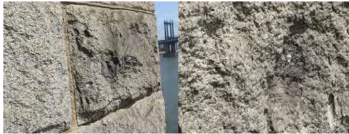
Brooklyn Bridge Tower Stone Scaling in 2016.
