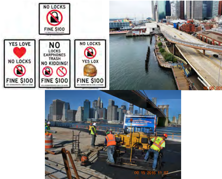
On September 8, 2016, a Guy-Wire Connected to a Street Lamp Over the Brooklyn-bound Traffic Snapped Under the Weight of the “Love Locks” Clipped to it, Shutting Down a Lane for Two Hours While Repairs were Performed. In October 2016, the Division Posted 16 Signs on the Lampposts and Along the Walkway Warning Lovers That Attaching “Love Locks” Onto the Bridge Could Leave Them Facing a $100 Fine. The Locks Pose a Danger to the Infrastructure and the Cars on the Brooklyn Bridge – More Than 34,200 Locks Were Removed Since the Division Began Keeping Count in 2013. 2,923 Love Locks Were Removed From the Bridge From January through April 2016, and Another 3,072 Between September and November 2016. October 2016: View of Ramp C Piers from Brooklyn Bridge. November 2016: Asphalt Placement at Fender System.
