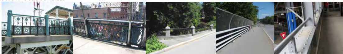
University Heights Bridge Railing. (Credit: NYSDOT) Manhattan Bridge Railing. (Credit: Russell Holcomb) Greywacke Arch Railing. Northern Boulevard over Cross Island Parkway – Left Sidewalk Railing in 2016. Staten Island Pedestrian Bridge over Parking Lot Exit Roadway – Right Side Railing of Span #2.
