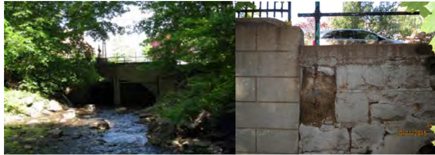
Forest Avenue Bridge Over Clove Lakes Park Stream. End Abutment Stone Masonry Wingwall. (Wingwall Credit: NYSDOT)
