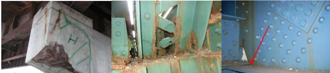
February 2008: Yellow Structural Flag Due to the Deteriorated Cap Beam. October 2008: Corrosion of Steel Secondary Member. November 2008: Crack in Steel Girder.
