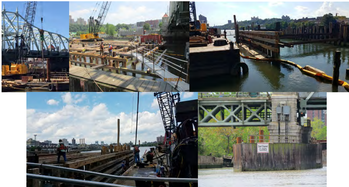
University Heights Bridge. April 2016: Pile Driving Operation. July 2016: Pier 3, Left Side, Repaired Wooden Catwalk. (July Credit: NYSDOT) September 2016: Installing and Securing the Whaler Timbers at the South and East Faces of the Fender. East Channel Closed Sign.
