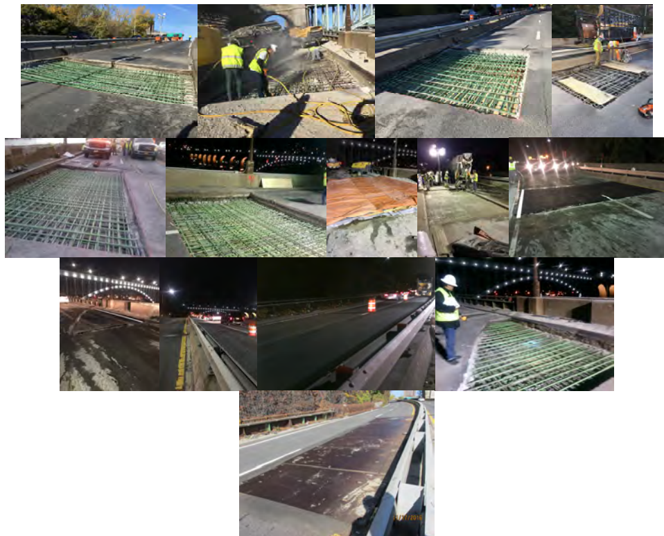
November 2016: Lathers Placing Rebar. Burlap, Plastic and Winter Blankets are Used to Cover the Concrete and Supply a Curing Environment. Span 17 and 18 Southbound Left Lanes - Metal Plates. (Plate Credit: NYSDOT)
