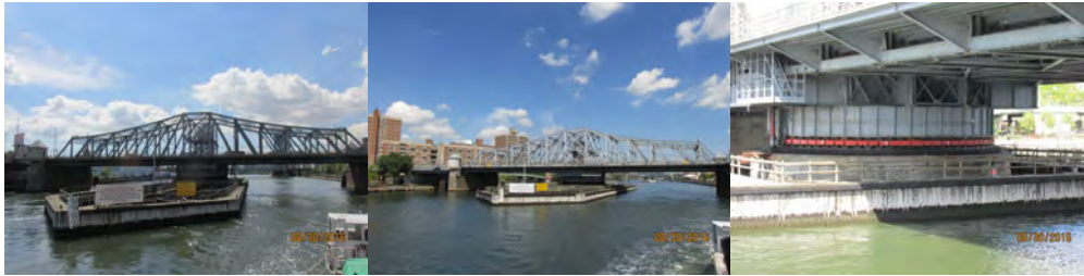
Madison Avenue Bridge in 2016: Left and Right Elevations Spans 12 to 15. Pier 13. (Credit: NYSDOT)
