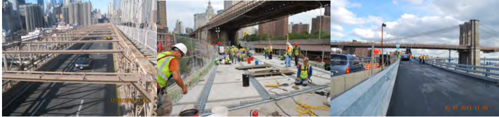
December 2011: Painted Top Struts of the Brooklyn-Bound Manhattan Side Span. Summer 2011: Manhattan Approach - Ramp C Deck Replacement. December 2011: Ramp C.
