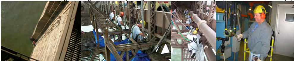
Repairing the Brooklyn Bridge Standpipe System, 130 Feet Below the Roadway. Maintenance Crew Conducting the Annual Cleaning and Lubrication of the Solid Rod Suspenders and Spherical Bearings on the Brooklyn Bridge. 2 nd Photo - Oilers Steven Marxhausen, Rene Francis, Richard Morreale, Thomas McAuliffe, and Andrew Sorrentino. (Credit: Anatoly Orlov) Oiler T. McAuliffe at the 9 th Street Bridge
