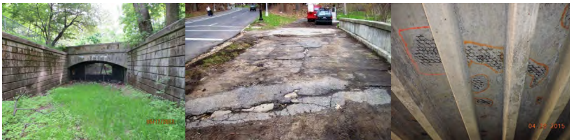
East Drive Bridge over Bridle Path. April 2015: Span 1 - Underside of Deck Exhibits Spalled Concrete With Exposed Wire Mesh. (Credit: NYSDOT)
