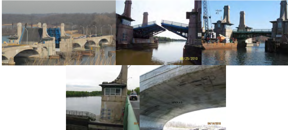
Bridge Closing in 2010. (Credit: NYSDOT) General View of Bridge Operator House #3 in 2011. Bridge Operator House #3 Exterior Wall in 2016, Looking Northwest. Underside of Arch Span # 5 - Spalled Concrete With Exposed Rebar is Secured With Netting.
