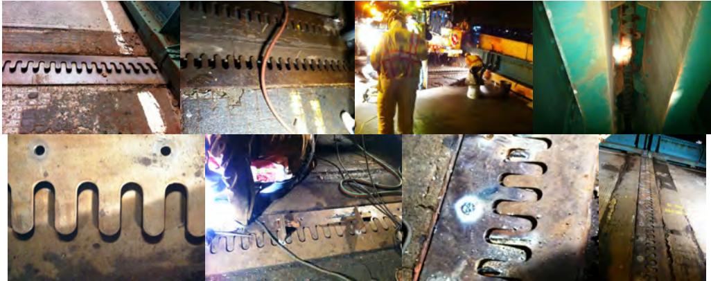
July 2013 PIA Safety Flag on the City Island Bridge. The repairs, conducted after a record-breaking heat wave, involved opening the joint plates and installing plug welds, which helped correct the plates' position and recreated the proper gap to allow the bridge to expand and contract safely. Finger Joint Before the Repair. Open Finger Joint. Division Crews Repairing the Joints. View Beneath the Finger Joint. The Joint Plates are Placed to Check for the Proper Gap. Leveling the Plate Before Welding. Close-Up of a Plug Weld. After 17 Plug Welds, the Finger Joints Sit Flush on the Roadway.
