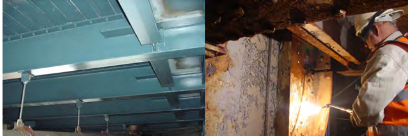
Stringers on the Manhattan Bridge. (Credit: NYSDOT) Bridge Repairer and Riveter Joseph Antony Repairing a Red-Flagged Stringer on the Bridge. (Credit: Hany Soliman)
