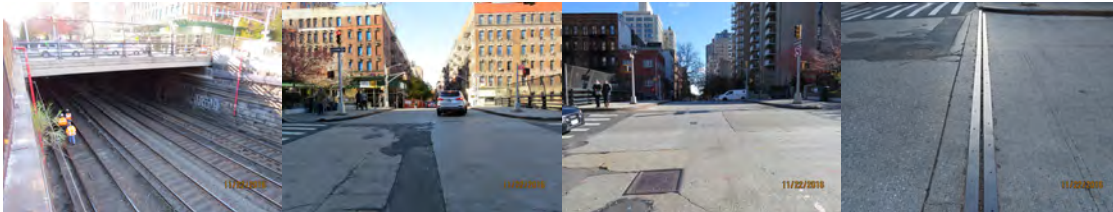
East 97 th Street Bridge over Metro North. 2016: Beginning and Ending Approaches. Beginning Abutment Joint - Deteriorated Sealer Material. (Credit: NYSDOT)
