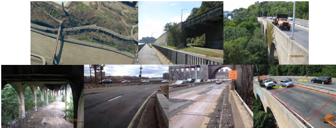
Aerial View. Trans-Manhattan Expressway Connector Ramp in 2014: Elevation Right Spans 1 – 25, 33 – 40. Span 42, Netting at Deck Underside, Looking Ahead. (Credit: NYSDOT) March 2015 Field Inspection. September 2015 - Span 42, Northbound Roadway, Looking Back. (Credit: NYSDOT)
