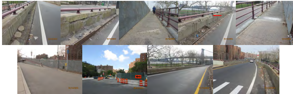
January 2016: South Approach Ramp - Span 2, Left Side Safety Walk and Curb. End Approach, Left Parapet. Span 4, Left Cantilever Sidewalk. North Approach Ramp – Span 2, Right Parapet and Safety Walk. Span 3, Right Cantilever Sidewalk. Elevation Right. 2016: Main Bridge – Spans 1 and 2 at Left Side. South and North Approach Ramps, Span 1 Top of Deck Wearing Surface.
