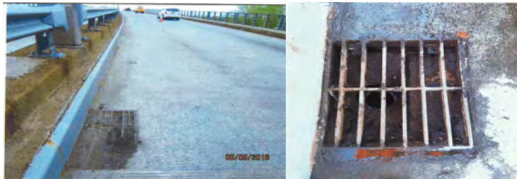
Debris and Sediment Fully Clogging a Scupper on the Northbound Roadway of the Boston Road Bridge over the Hutchinson River. Scupper After Cleaning.
