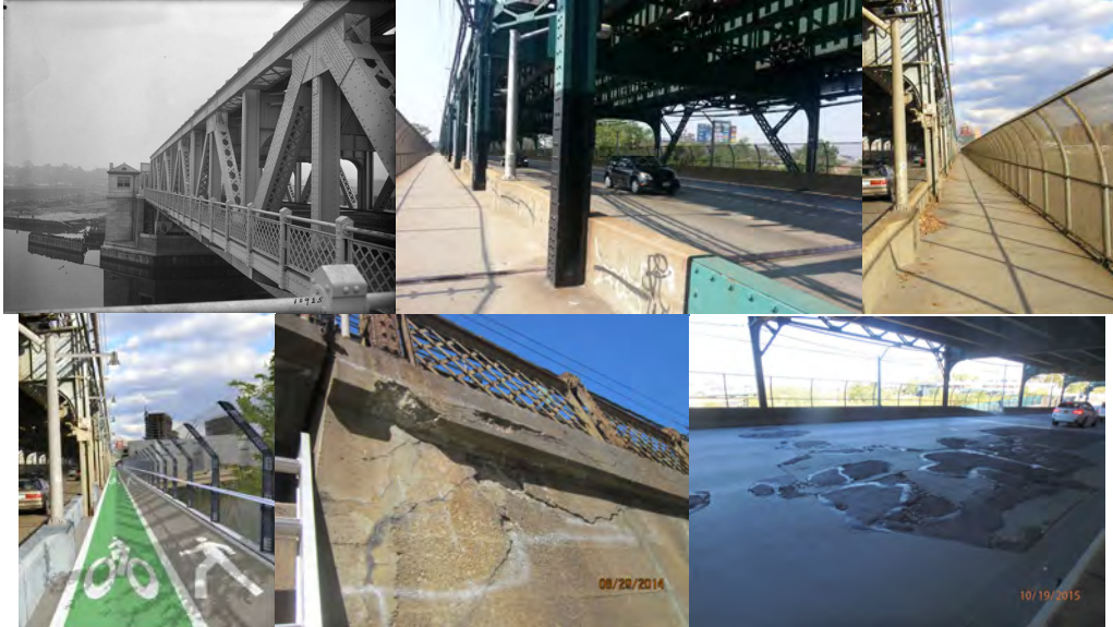
Roosevelt Avenue Bridge – In 1927. (Credit: NYC Records). Looking East. Existing and Proposed Bicycle/Pedestrian Path. 2014: Right Wingwall at the End Abutment. The Top Exhibits an area of Diagonal Cracks With Efflorescence and Spalls. The Deteriorated Concrete Areas are in Safe and Stable Condition. 2015: Spans 26 and 27 – Examples of Uneven Asphalt Patches and Broken Concrete Areas. (Credit: NYSDOT)
