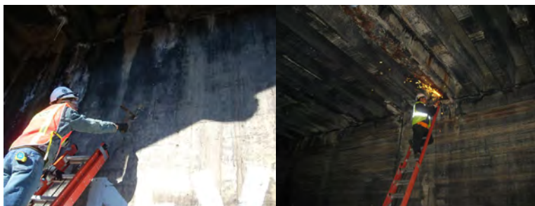
2010 Inspection - Hands-On Inspection of A Pier. Obtaining a Steel Coupon Sample From a Stringer.
