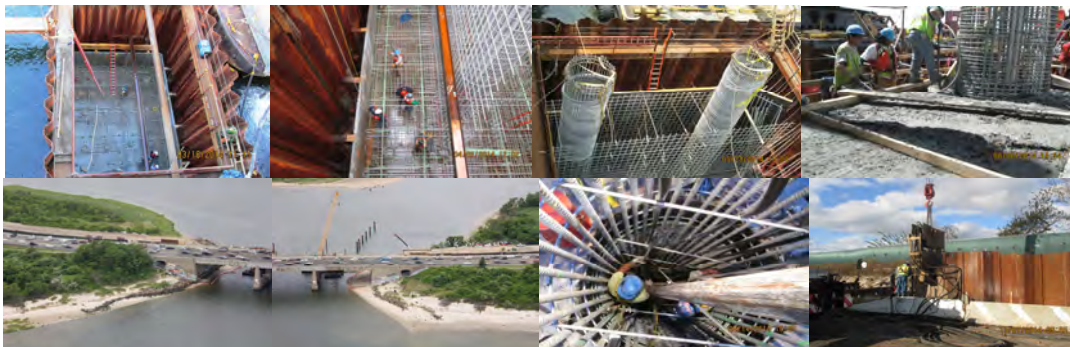
Gerritsen March 2014: Setting Footing Rebars Prior to Placing Pier Rebars and Concrete at Pier No. 2. April 2014: Setting Rebars for Footing and Pier Inside Cofferdam at Pier #1. May 2014: Plinth and Column Reinforcement Inside the Cofferdam for Pier 2. June 2014: Placing and Vibrating Concrete for Plinth at Pier #1. Rebars for Column in Place. West Abutment of Bridge. New Roadway Under Construction at top Next to Westbound Lanes. East Abutment of Bridge. Crane on Barge at Cofferdam for New Pier #2. August 2014: Workers Inside Rebar Cage During Operation of Pumping Concrete Into Pier #2 Column. November 2014: Steel Sheeting in Place for the East Approach Temporary Access Roadway.
