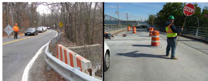
Flagperson at the Rockland Avenue at Manor Road Culvert, and at Hannah Street Over SIRT.
