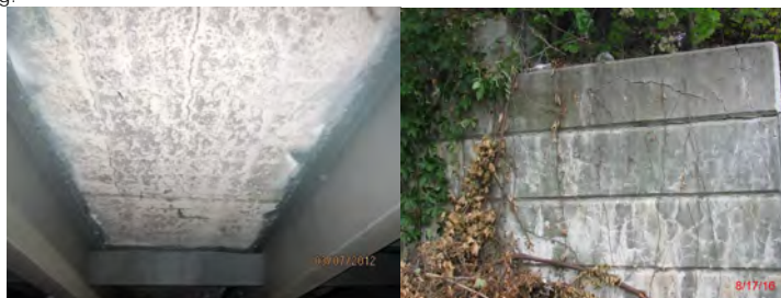
Union Street Bridge over Brooklyn-Queens Expressway in 2012 - Extensive Map Cracking With Efflorescence on the Underside of the Deck. (Credit: NYSDOT) Tompkins Avenue Bridge over B&O Railroad (Abandoned) in 2016 - Map Cracks With Efflorescence Near the End of the Wing Wall.
