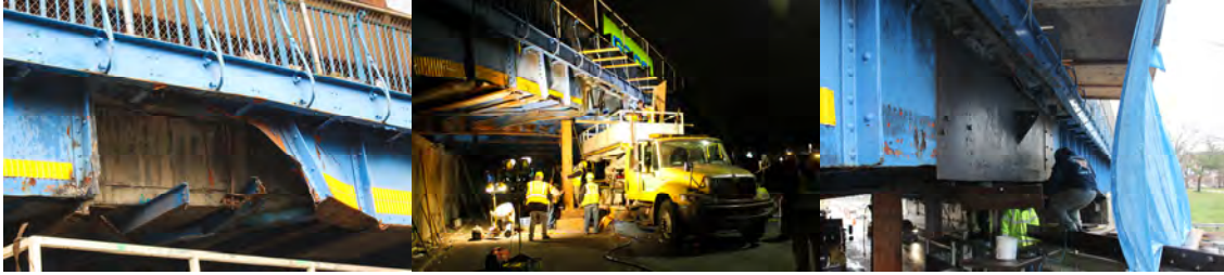
On January 9, 2016, a Truck Travelling South on the Parkway Struck the Bridge, Causing Damage to a Fascia Girder and its Preceding Girders, Stringers, and the Hanging Bars of a Strongback. Crews Responded, Cut a Portion of the Sheared Girder and Spliced it With a New Section and Installed Shoring.
