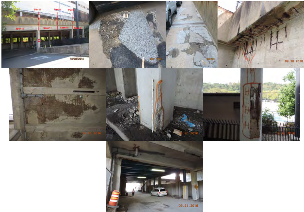
Matthewson Road Bridge over MacCracken Avenue. (Credit: NYSDOT) March 2016: Spalled and Exposed Rebar on Wearing Surface of Span 2. Left Sidewalk on Span 8. September 2016: Span 2, Underside of the Left Parapet and Left Face of Girder Exhibit Spalls with Exposed Rebar. Pier 7, Right and Left Columns Exhibit Exposed Rebar and Hollow Sounding Concrete. End Pier. (September Credit: NYSDOT)
