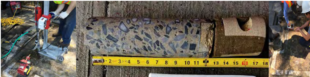
Utilizing a Coring Machine to Obtain a Concrete Core for Testing. June 2016: Core Sample from the Westbound BQE over Adams Street. Ground Penetrating Radar Utilized to Locate Rebars.
