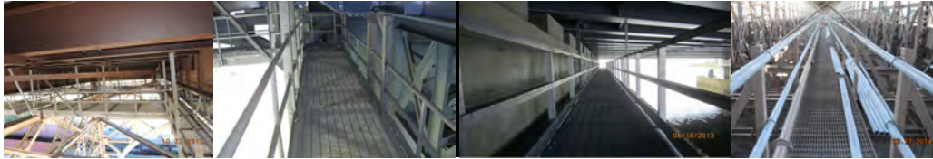
Ed Koch Queensboro Bridge Lower Level Flooring System Catwalk under Span 37. Manhattan Bridge Brooklyn Tower Catwalk. (Credit: NYSDOT) Fresh Creek Catwalk Under Deck. Brooklyn Bridge Manhattan Side Catwalk. (Brooklyn Credit: NYSDOT)
