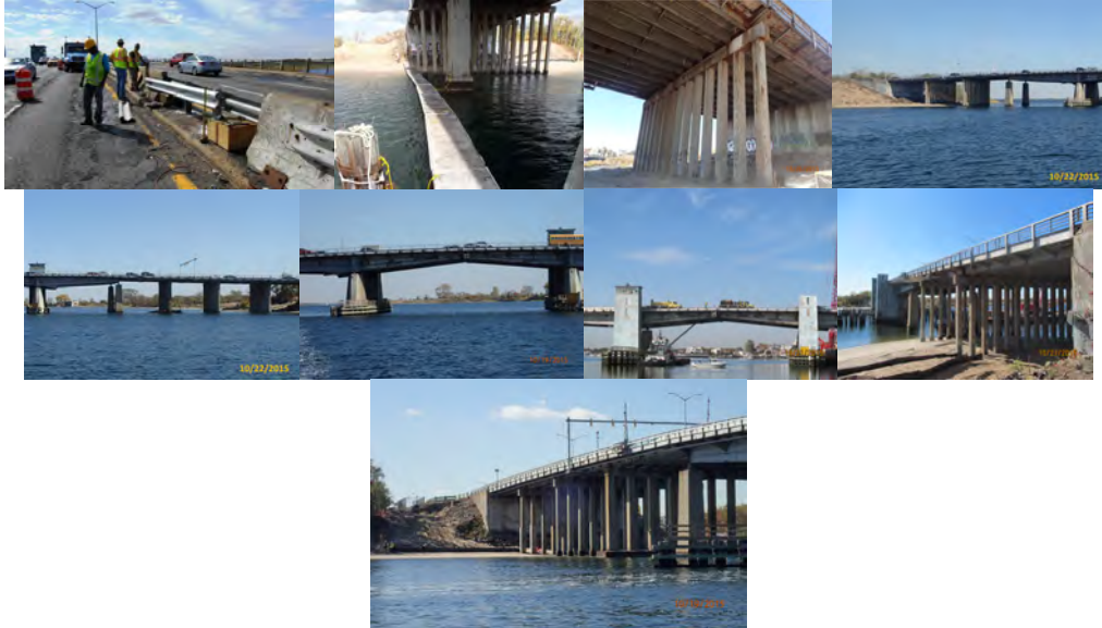
Mill Basin September 2015: Median Guide Rail Repair Operations on East Side of Bridge. October 2015: Temporary Walkway on North Side of Bridge for Access to Pier #9. Current Mill Basin Bridge in October 2015 - Span 11 Pier 11 - Columns with Cracks, Hollow and Spalls. Elevation Left Span 1-7, 7-14. Span 8. Elevation Right Span 8, 9-14, 1-7. (Inspection Credit: NYSDOT)
