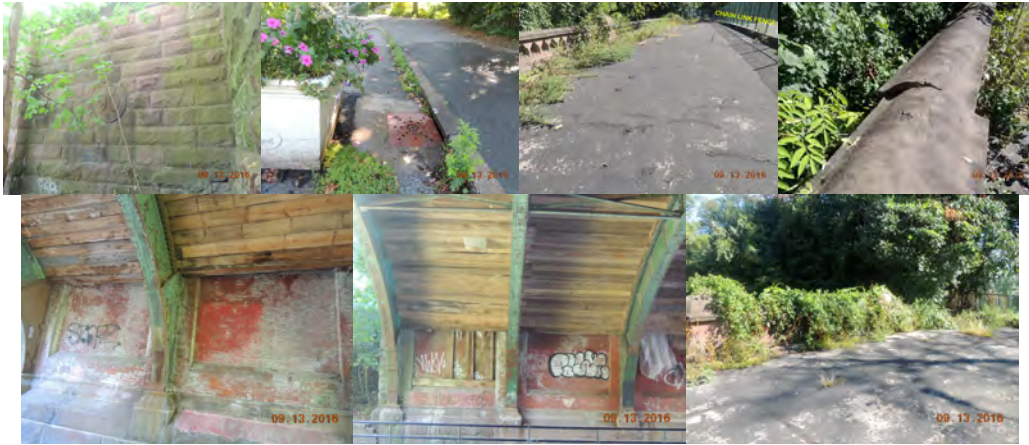
Hill Drive Bridge in 2016: Span 1, Left Exterior Enclosure Wall. End Approach at Right Curb Line. Spans 1 Through 3 Wearing Surface - Exhibits Partially Sealed Asphalt Cracks and Vegetation Growth on the Left Side. Span 1 Left Railing- Shifted but Stable Stone Railing Coping. Pier 1 Between Bays 4 and 5 - Exhibits Efflorescence and Water Stains Through the Brick. Span 2 Brick Arch - View of Installed Timber Shielding. Span 3 Left Parapet and Railing - Heavy Vegetation Growth. (Credit: NYSDOT)
