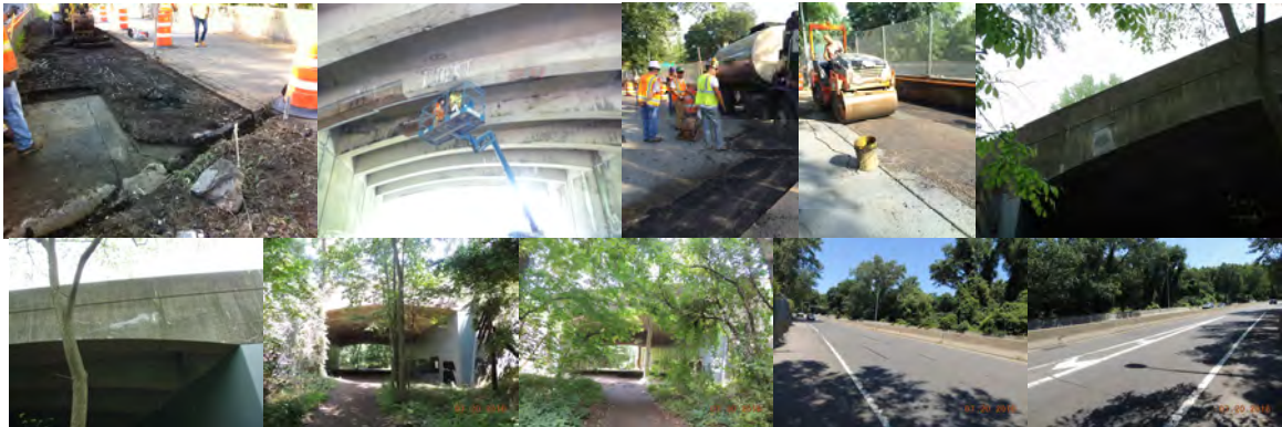
Mosholu Parkway Bridge over Conrail (Abandoned). Conditions in June 2015. Asphalt Work in July 2015. May 2016: Right Fascia Near Beginning Abutment – Repaired Spalled Concrete Area. Right Fascia Near End Abutment – Repaired Stringer. Elevation Left and Right, and Approach Begin and End in July 2016. (2016 Credit: NYSDOT)
