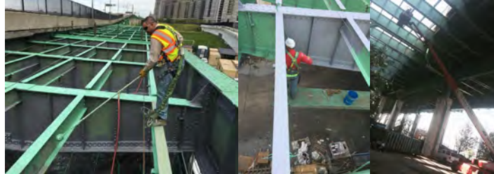
Bridge Painter Juscelino Andrade Painting the Miller Highway (Joe DiMaggio Highway) over Terrain. (Credit: Arlindo Lima)
