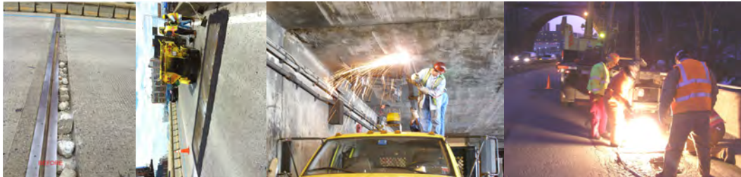
August 2014 PIA Safety Flag: Broken Joint Concrete Header And Steel Armor on the Long Island Expressway over Dutch Kills Creek. The Condition Was Made Safe By Installing Two Steel Plates. PIA Flag (Truck Wedged Under the FDR Drive at Span 41): Removing the Debris. (Credit: Victor Sandoval) PIA Flag Repair (Through Hole) on Harlem River Drive Ramp. (Credit: Bojidar Yanev)
