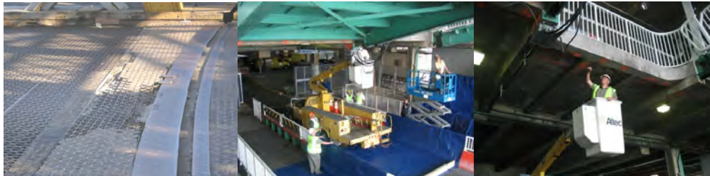
Example of PIA Safety Flag: Broken Grating. Associate Project Manager Thomas Whitehouse (White Hardhat) Ensuring the Proper Setup of Containment Procedures at the St. George Ferry Terminal Landing Slips Before the Masons Address A PIA Flag (Falling Concrete). Inspecting the Flagged Condition.
