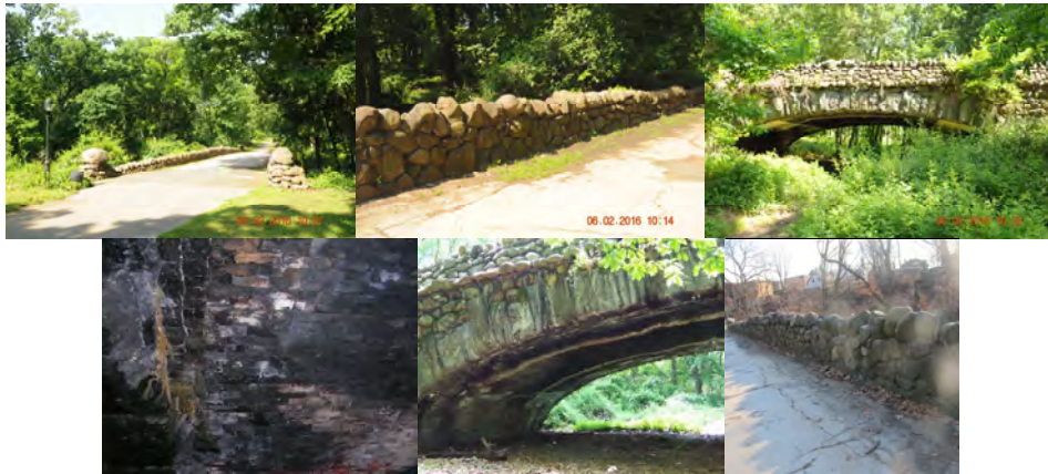
June 2016. Under-Deck Cracks and Missing Bricks - North-East Side. Under-Deck Arch Wall Showing Efflorescence Along the Cladding Stone and Brick Arch. Top of Bridge - Map Cracking, Spalled, and Patched Areas.
