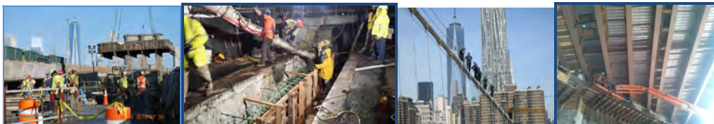
April 2014: York Street Structure Deck Replacement During Full Weekend Closure. May 2014: Main Street Structure – Abutment Concrete Placement. May 2014: Ascending the Cable. July 2014: Preparation for Closure Pour at Main Street Structure.
