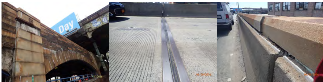
May 2016: Span 43, Right Side Fascia - the Stone Masonry Curtain Wall Exhibits Localized Moderate to Heavy Efflorescence Formation at Several Mortar Joints at the Outside Face and at the Underside of the Arch. Pier 19 Joint, Atlantic Avenue Westbound - Approximately 40% Length of Joint Compression Seal is Slightly Debonded. Spans 33 thru 35, Top of Deck, Right Fascia at Right Bridge Railing - Separation (up to 2") of the Fascia Stones From the Bridge Railing. (Credit: NYSDOT)
