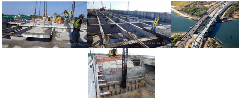
September 2015: Removing Saw-Cut Deck Panels. Deck Removed Prior to Steel Removal. October 2015: Stage 2 Traffic Pattern. Westbound Traffic at Right on New Bridge. Eastbound Traffic at Left on Existing Bridge. December 2015: Driving 14-Inch Diameter Steel Shell Piles at East Abutment - Facing East.
