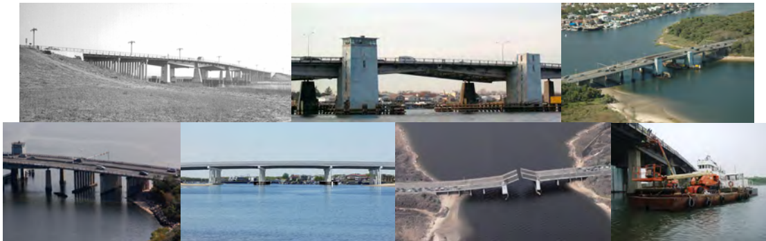
Mill Basin Bridge in 1946. Aerial Views. Proposed Bridge. Open Bridge. May 2013 – Inspecting the Bridge From a Barge.
