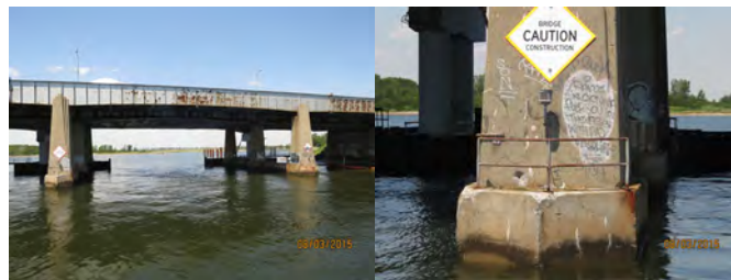
Current Gerritsen Inlet Bridge in August 2015 - Span 6, Right Fascia, Looking Left. Span 6, Pier 5, Column 3 – Construction Sign and Non-Functioning Light. (Credit: NYSDOT)
