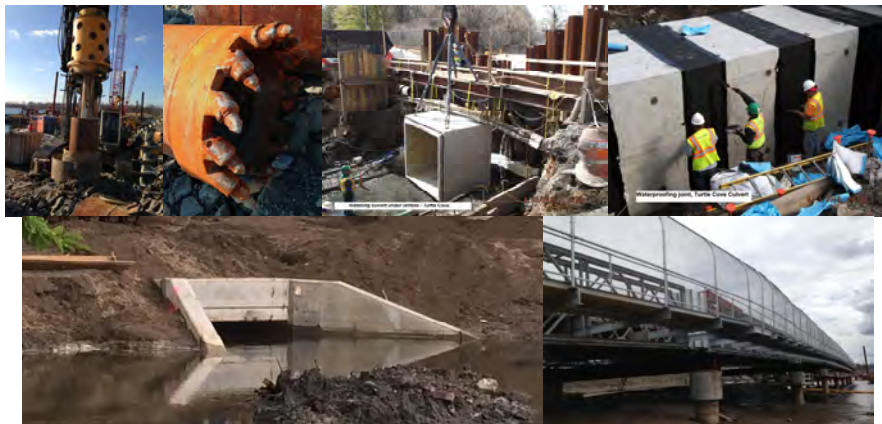
January 2015: Drilling Rig Construction Vehicle Used to Install Land-Based Drilled Shaft Casing for the Temporary Bridge. The Bucket Drills Carve Out the Casings With Teeth Capable of Tearing Through Rock. April 2015: Turtle Cove Culvert Replacement. Installing Culvert Under Utilities. May 2015: Waterproofing the
