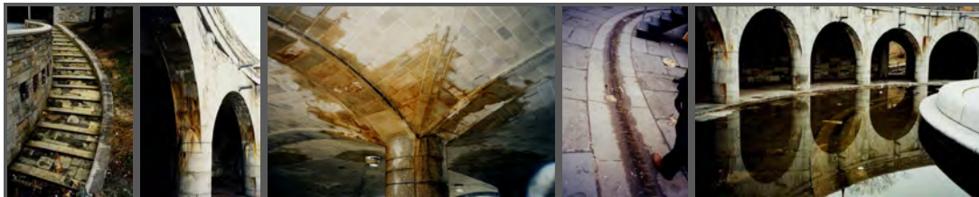
Pedestrian Plaza Level: South Stairway - Deterioration and Missing Stone Steps. Stone Clad Columns - Extensive Efflorescence and Staining. Guastavino Arch - Ponding Water and Efflorescence. Fountain Trench Drain - Deteriorated Grating and Clogged Drain. Extensive Water Ponding.
