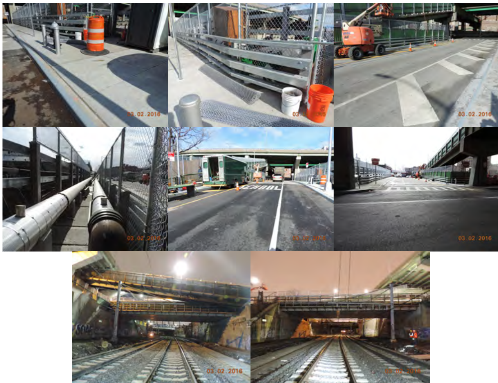
March 2016: Begin Approach, Right Sidewalk – New Concrete Sidewalk and Curb With Steel Facing. New Guide Rail. Span 1, New Concrete Overlay Wearing Surface. New Water-Mains on Top of Deck. Approach Begin and End. Left and Right Elevations. (Credit: NYSDOT)
