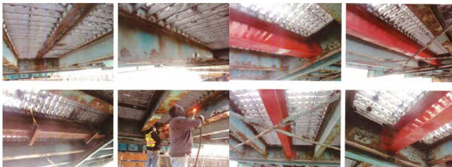
December 2016: Removing and Replacing a Severely Corroded Stringer Under Span 1 on the Grand Street Bridge over the Newtown Creek.
