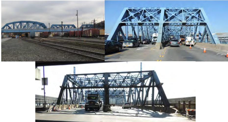
Leggett Avenue Bridge over Amtrak. October 2016: Begin and End Approaches. (Credit: NYSDOT)
