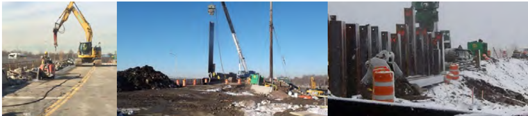
January 2016: Demolition - Removal of the Fencing and Temporary 16" Water Main From the South Side of the Bridge. Installing Metal Sheeting Plates on the East Approach. February 2016: Sheeting Operations - These Metal Sheets Will Act as a Support Brace When the Contractor Begins Ground Excavation.
