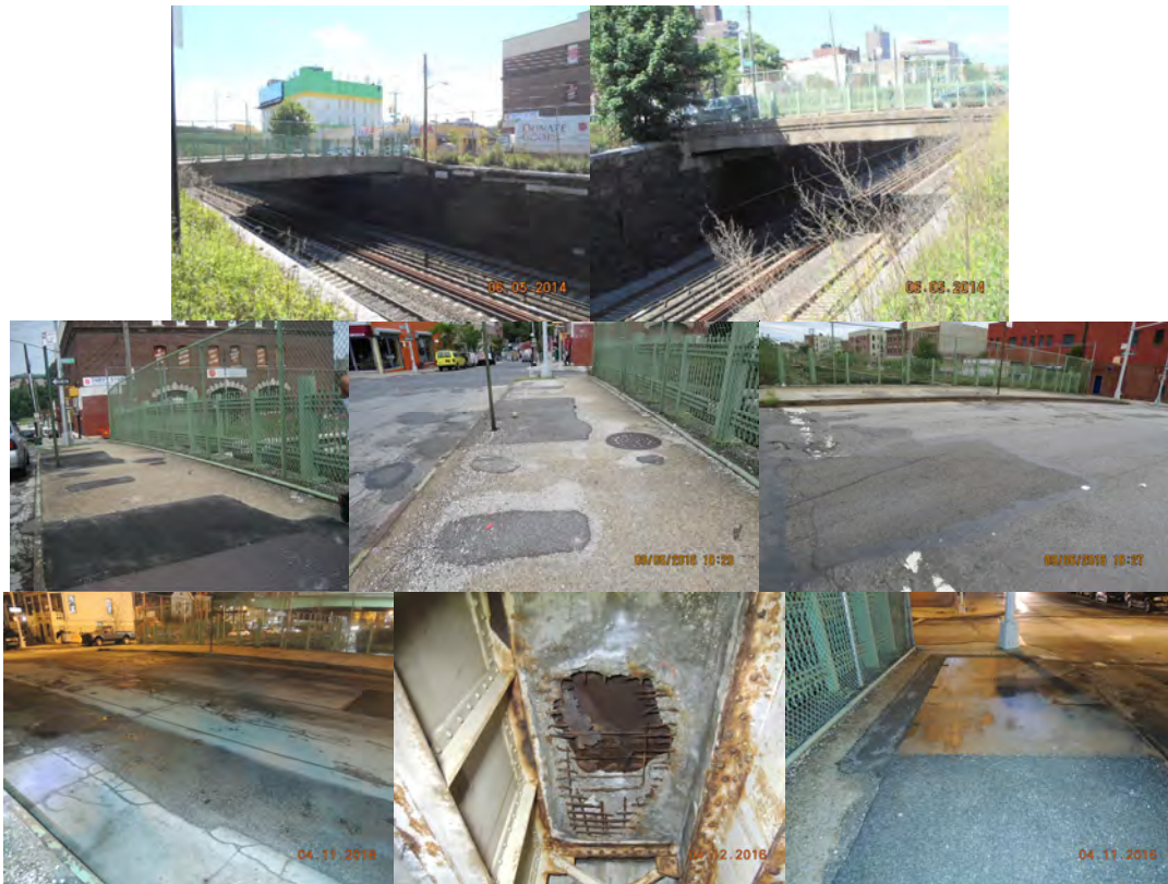
2014: East 175 th Street Bridge Left and Right Elevations. (Credit: NYSDOT) Sidewalk and Road Conditions in 2016. April 2016: Span 1, Wearing Surface at Mid-Span – Uneven Asphalt Patches on Approximately 40% of the Surface Area. Underdeck of Span 1- Through Hole and a Deep Spall With Exposed Rebar Near the End Abutment. There is a Steel Cover Plate Above. (April Credit: NYSDOT)
