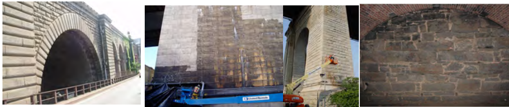
Brooklyn Bridge Cliff Street Arch Masonry. Cleaning the Masonry of the North Face of the Manhattan Bridge's Brooklyn Anchorage and of the North and East Faces of the Roosevelt Island Pier of the Ed Koch Queensboro Bridge. Masonry of the East Drive Bridge Over Eastwood Arch.
