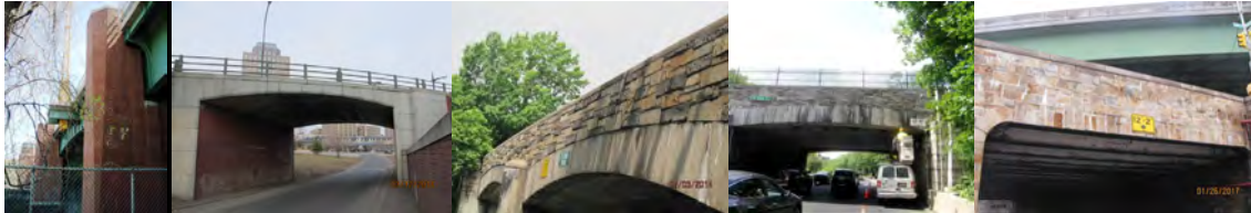
Hutchinson River Parkway Bridge. Brooklyn-Queens Expressway Over Ramp to Brooklyn-Queens Expressway (Eastbound). Right Side Fascia on the Bronx Pelham Parkway Bridge. Inspecting the Cladding Stones of the Fascia of Span 1 on West 252 nd Street Bridge Over Henry Hudson Parkway. Eliot Avenue Bridge Over Queens Boulevard.
