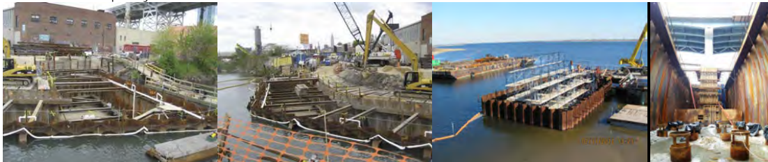
April 2010: Cofferdam With Filter Fabric and Gravel Placed Prior to Pile Driving During the Emergency Repair Project on the Borden Avenue Bridge over Dutch Kills. February 2011: Fresh Creek Bridge Cofferdam Pad. May 2016: View Inside the Gerritsen Inlet Pier 2 Cofferdam.
