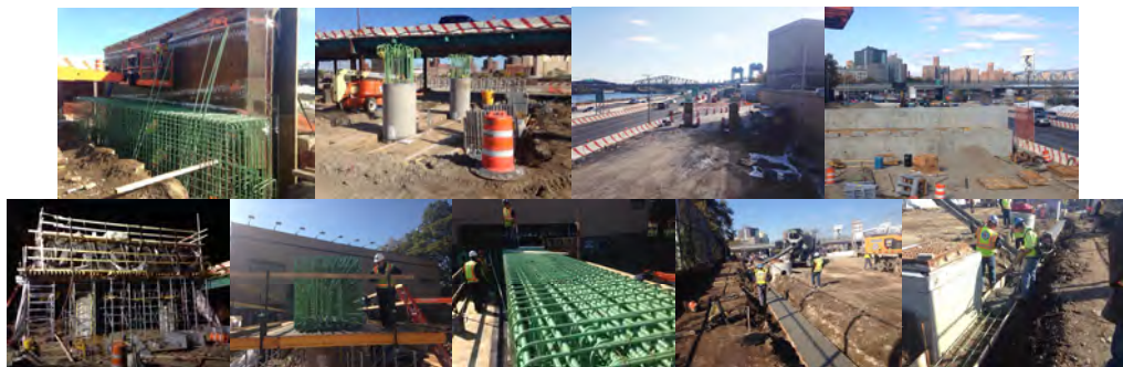
November 2016: South Abutment Stem Wall. Pier 1 - Scaffolding to Begin Setting up Steel Reinforcement and Formwork. General View of Construction Site From Pier 8 - Looking South. The North Abutment. Concrete Placement. (Credit: Artemio Angeles). Reinforcing for Pier 8 Cap Beam Being Inspected by Resident Engineer Jose Jardim. (Credit: Richard Solomon)
