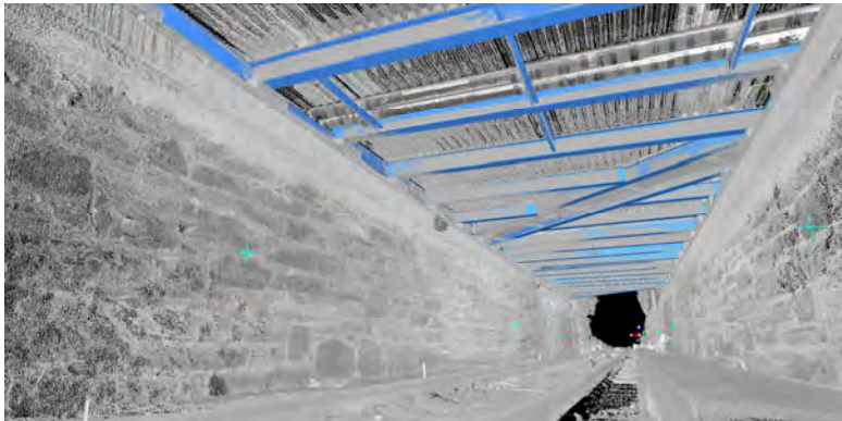
LIDAR Scan Image of the Jackson Avenue Bridge over LIRR Montauk Division In-depth Inspection). (Credit: Sarah Jurado)
