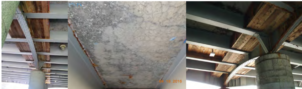
Span 1 Deck – Hollow Sounding Concrete Areas are Covered by Timber Planks That are in Good Condition. April 2016: Span 2, Underside of Deck, Bay 3 - Exhibits Scaling, Mapcracking with Localized Efflorescence, and Dampness Over Approximately 50%-60% of its Surface. (Credit: NYSDOT) July 2016: Span 2 Timber Shielding.
