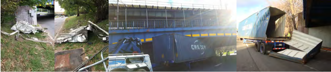
October 2016: Truck Debris Remaining at the South Side of the Bridge Along the Southbound Hutchinson River Parkway After a Bridge Strike. December 2016: Truck Tightly Wedged Under the Bridge.
