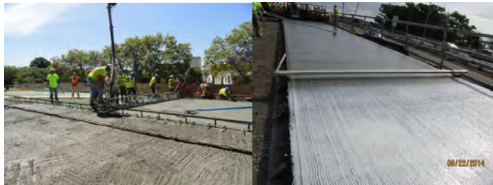
Screed at East 8 th Street Ramp in 2011, and at West Approach of Gerritsen Inlet Bridge in 2014.
