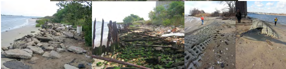
Tidal Wetland Mitigation Site. Before Mitigation – Large and Heavy Surface Debris and Deteriorated Bulkhead. Inspecting the Hurricane Sandy Damage at the Site in January 2013.
