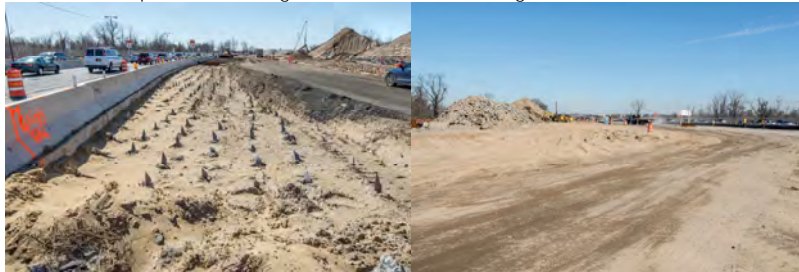
Northwest Quadrant Wick Drains for the New Mill Basin Bridge. Drains Backfilled.
