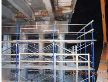
Mill Basin Bridge Scaffold Used During Pier Cap and Pier Column Repairs.
