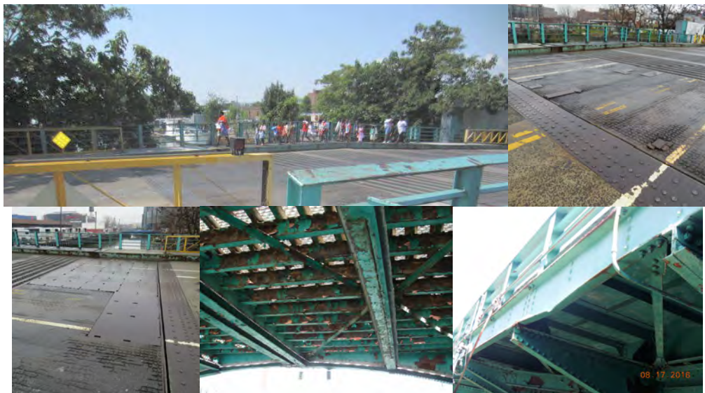
Union Street Bridge - Schoolchildren Crossing in 2012. (Credit: NYSDOT) Steel Plates Covering the Steel Grid Deck. 2016: Severe Corrosion and Peeling Off Paint Under Deck of Span #3. Span 3 - The Left Fascia Stringer Exhibits Impact Damage. (Impact Credit: NYSDOT)
