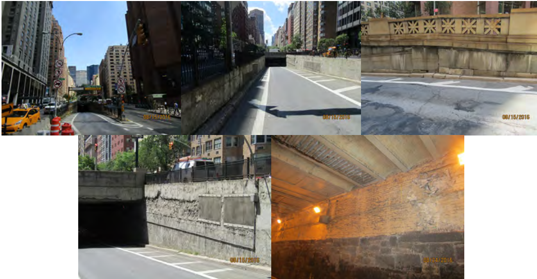
Park Avenue Tunnel – Left and Right Elevations in 2016. Begin Left Wingwall - Stones are Partially Dislodged, Cracked and With Missing Mortar. End Right Wingwall - Wall is Spalled and Exhibits Hollow Concrete Areas That are Shielded With Wire Mesh. End Abutment (Near South Portal) – Bricks Exhibit Deteriorated Mortar. (Credit: NYSDOT)
