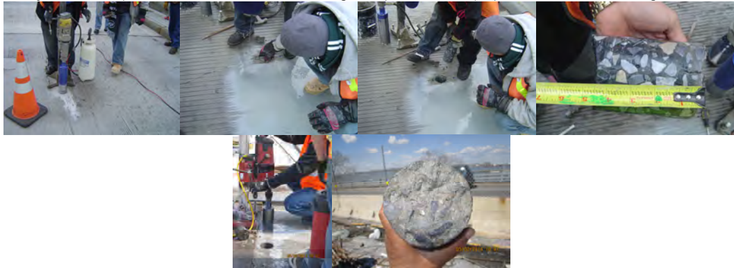
Removing a Core From 252 nd Street Bridge over Henry Hudson Parkway in January 2009. (Credit: Masroor Mahmood) Core Sampling on the Bay Ridge Avenue Bridge in 2014.
