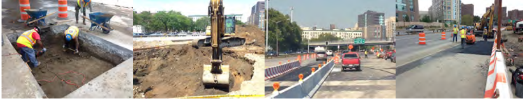
June 2015: Locating and Removing Utilities. Excavating and Removing Big Rocks. September 2015: Painted Concrete Barriers Near Ramp C and Temporary Roadway. October 2015: Adjusting the Grading on the New Temporary Roadway. (Credit: Artemio Angeles)
