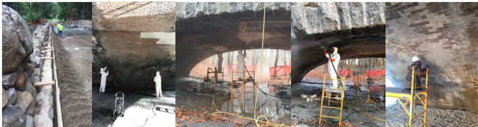
October 2016: Concrete Curb Layout. November 2016: Cleaning the Bricks Under the Bridge Arch. December 2016: Cleaning the Historic Stone Masonry and Removing Graffiti. Tuck Pointing the Bricks Under the Bridge Arch.
