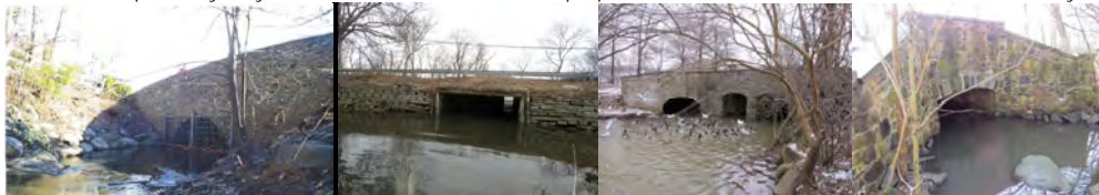
Sweet Brook Road Culvert. Richmond Terrace over Snug Harbor Culvert. Victory Boulevard Culvert. Arthur Kill Road Over Clarke Avenue Culvert.
