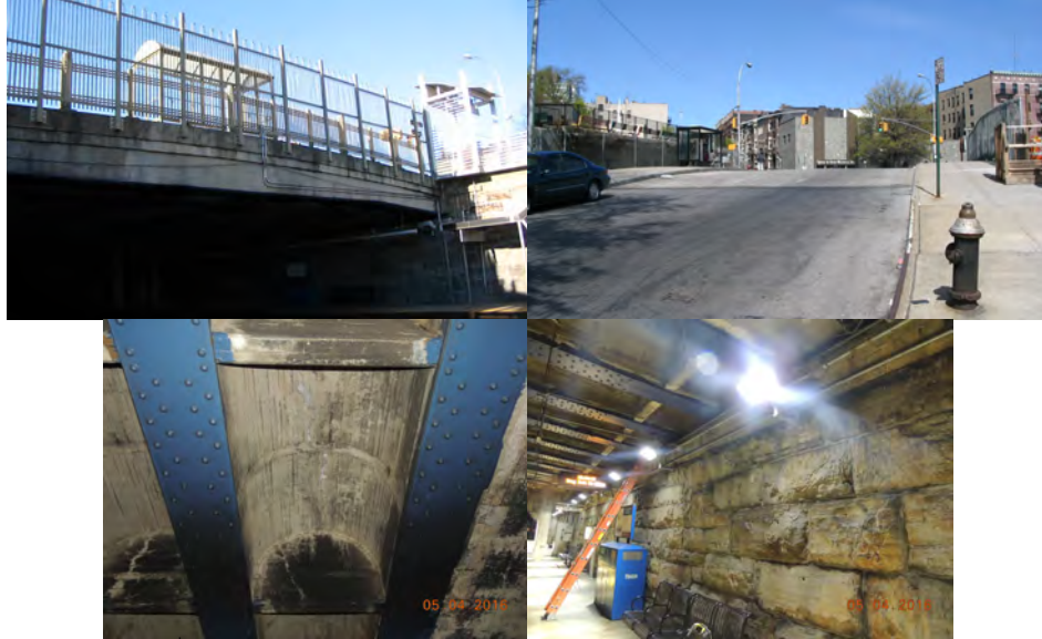
East 162 nd Street Bridge over MNRR. May 2016: Span 1, Underside of Deck Exhibits Longitudinal Cracks With Efflorescence. End Abutment Stem. (Credit: NYSDOT)
