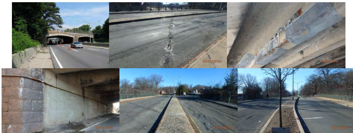
Douglaston Parkway Bridge Northbound Over Cross Island Parkway. March 2016: Top of Bridge, Asphalt Wearing Surface Above Beginning Abutment - Spalls and Uneven Wearing Surface. Span 1 - Deteriorated Concrete Covered With Wire Mesh. Abutment End. Approach Begin and End. (Credit: NYSDOT)
