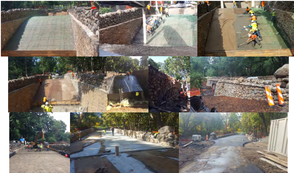
September 2016: Bridge Arch With Wire Mesh Reinforcement in Place Prior to Concrete Placement. Belt System Transporting the Concrete Into Position. Wet Burlap Placed Over Previously Finished Zones. Drip Hoses Placed to Keep Burlap Wet for the Next 7 Days. Center of the Bridge - Waterproofing Membrane Applied to Arch and Inner Walls of the Bridge. North Side of the Bridge - Cleaning the Historic Stone Masonry and Concrete Surfaces. Rubble Stone Work – the Darker Stones Have the Graffiti Protection Applied. Center of the Bridge - Backfilling and Compaction. After Backfilling, the Concrete Base for the Roadway was Placed. Following the Curing of the Concrete Base, Asphalt was Placed.
