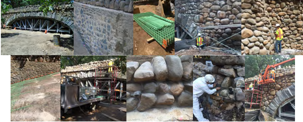
August 2016: Temporary Support Structure Under the Arch. Interior Walls After Power Washing. Epoxy-Coated Mesh Reinforcement. Chipping Out Existing Mortar. Top of Arch - Layout of Epoxy-Coated Mesh Reinforcement and Dowels. South Fascia – Cleaning the Existing Stone. South Fascia Parapet - Finished area – Cleaning, Chipping, and Repointing. North of Bridge - Cleaning and Repointing the Rubble Stone Masonry.
