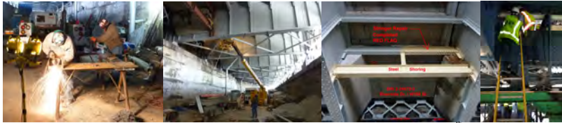
February 2011: Red Flag Stringer Repair at Riverside Drive Viaduct over West 158 th Street. July 2015: Highway Transportation Specialist Andrew Hoang and Assistant Civil Engineer Medina Inspecting a Red Flag on the Manhattan Bridge From the Motorized Bridge Inspection Traveler Platform Beneath the Bridge. (Credit: Tiffany Wong)
