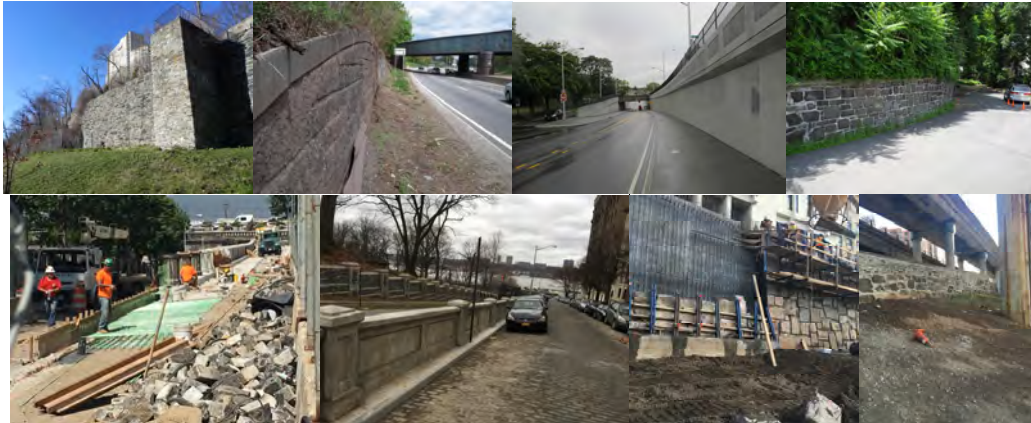
Retaining Walls: Irwin Avenue. Cross Island Parkway Southbound Before 100 th Avenue. Cooper Avenue. Douglas Road. 2016: West 155 th Street (Lower Level) Between Riverside Drive and Broadway During and After Rehabilitation by DDC. Riverside Drive (Northbound) to George Washington Bridge (West 168 th to 171 st Streets) During Rehabilitation. Riverside Drive Under George Washington Bridge Ramps (West 176 th to 177 th Streets). (2016 Credit: Jacob Ayman)
