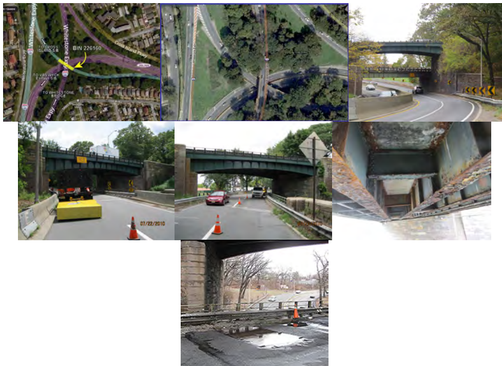
Location Map. (Credit: NYSDOT). Aerial View. Bridge (Lower Structure) in October 2016. Left and Right Elevations. (Elevation Credit: NYSDOT) Underside of Span #1 in October 2016 - Girders Have Rusted Bottom Flanges and Peeling Paint. March 2014: Steel Plates on Wearing Surface.
