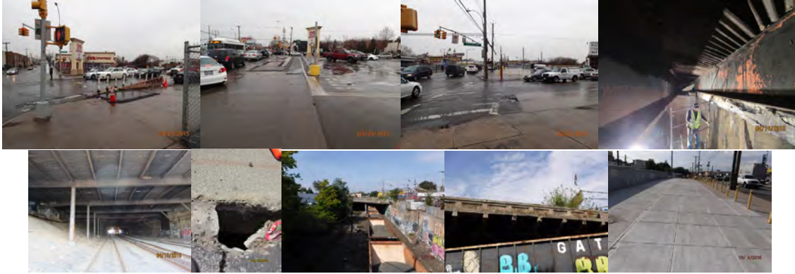
March 2015: Looking West, South, and East Across Bridge Deck. April 2015. October 2015: Elevation Right. Span 2 Right Parapet - The Outer Face Exhibits Spalls With Exposed Rebars. Spans 1 and 2 New Right Side Sidewalk. (Credit: NYSDOT)
