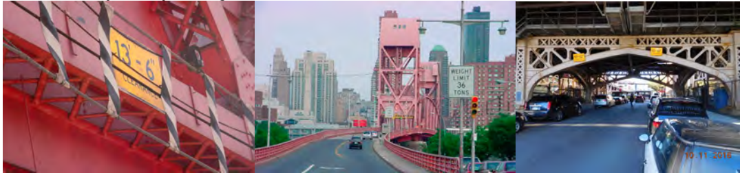
Roosevelt Island Bridge Vertical Clearance Restriction and Posted Weight Signs. Ed Koch – Queensboro Vertical Clearance Signs. (Credit: NYSDOT)
