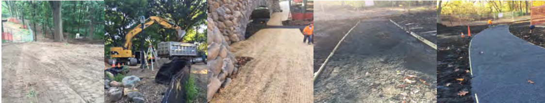
August 2016: North and South of Bridge – Clearing and Grubbing. November 2016: Placing Erosion Control Material Over the Slope Area on Both Sides of the Bridge. Placing Granular Fill Material (Crushed Stone) on the Bridge Pathway Under the Bridge Arch.
