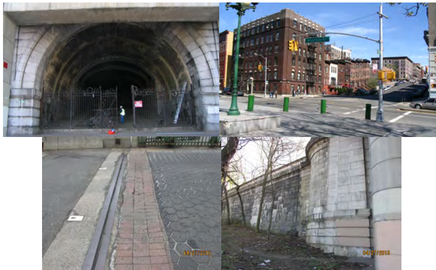
Riverside Drive Bridge over West 145 th Street. April 2015: Top of Deck, at Entrance to Riverbank State Park. East Abutment Wingwall. (Credit: NYSDOT)
