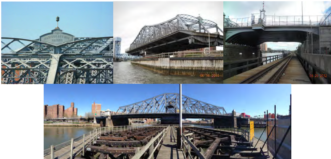
Madison Avenue Bridge Sign in 2007. (Credit: Duane Bailey-Castro) General View of Truss Swinging in 2010 and Right Elevation of Span 15 in 2012. (Credit: NYSDOT) North Elevation View.
