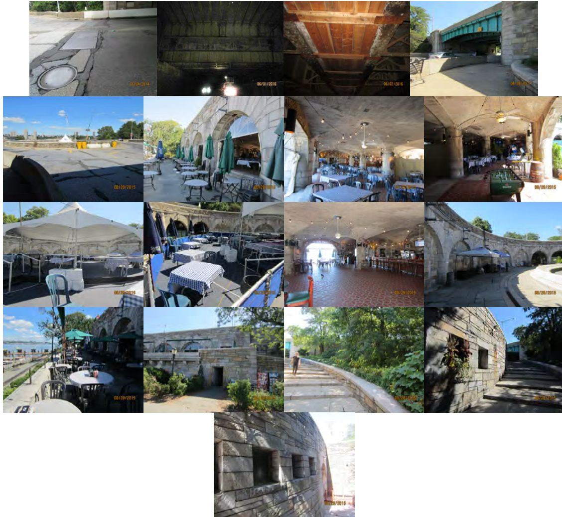
West 79 th Street Bridge Over Amtrak in 2014 – Beginning Abutment Joint – Top of Deck. June 2016: Left Elevation. Underside of Deck, Bay 7 – Timber Shielding. (Credit: NYSDOT) Traffic Circle Level. Plaza Level. Ramps and Façade.
