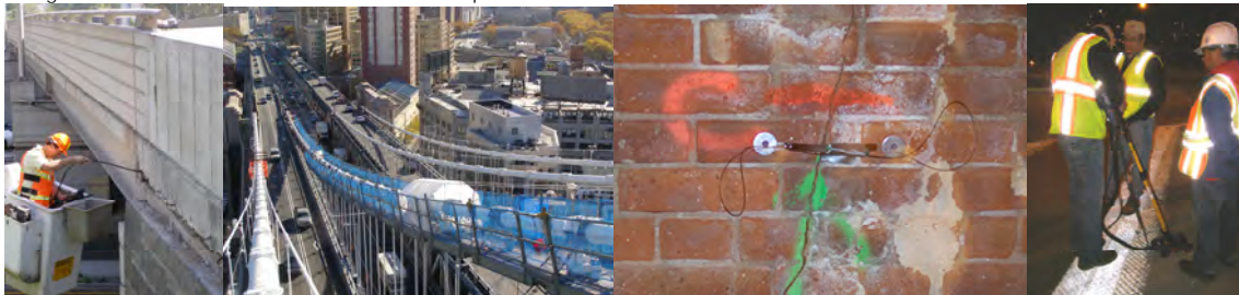
Director of Bridge Management Kevin McNulty Inspecting the Bridge Carrying the Belt Parkway over Ocean Parkway, Utilizing the Unit's Boreoscope. Experimental Corrosion Sensors Installed for a Test on Cable D of the Manhattan Bridge in 2011 (Left Corner). A Fiber Optic Sensor Monitoring a Crack in the Masonry of the Brooklyn Bridge's Manhattan Approach. A Ground Penetrating Radar Inspection of the Belt Parkway Bridge over Ocean Parkway. (Credit: Bojidar Yanev)
