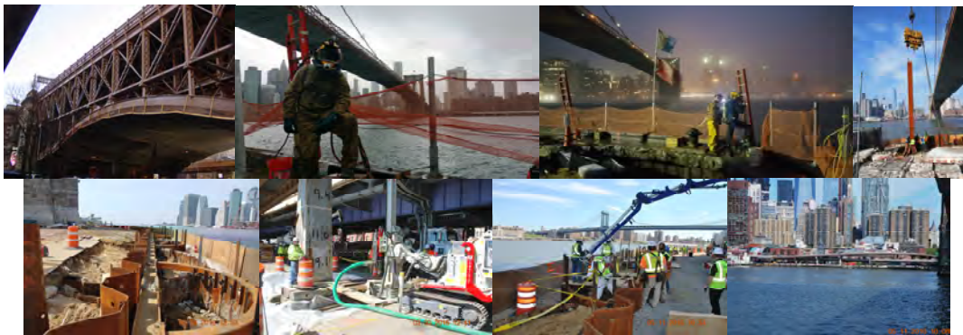
February 2016: Franklin Square Structure. (Franklin Credit: Maria Micolajczyk) Diver Geared up for Underwater Repairs to Steel Sheet Piling at Fender System. Divers About to Descend. March 2016: Driving Steel Sheet Piling at the Fender System. Steel Sheeting and Braces in Place for Cofferdam Reconstruction at Fender System. Installation of Bored-In Piles at Ramp C Pier Replacement. May 2016: Waterproof Concrete Placement at Fender System Cofferdams. View of Ramp C Piers from Brooklyn Shore.
