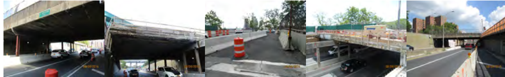
The Three Structures of the FDR Drive at Houston Street Overpass. 2016: Main Bridge – Span 2, Underside of Deck Slab. Partly Removed Deck Slab. Temporary Pedestrian Walkway. Left and Right Elevations in August.
