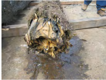
During the Demolition of the North End of the Existing University Heights Bridge Fender, Marine Borers were Discovered in the Southern Yellow Pine Piles. The End of a Pile Segment Removed From the Fender - Based on the Size of the Holes, Teredo Navalis is the Likely Species.
