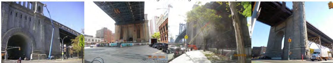
Inspecting the Exterior of the Manhattan Bridge Anchorage. Manhattan Bridge Brooklyn and Manhattan Anchorages. Ed Koch - Queensboro Bridge Queens Anchorage (Credit: NYSDOT)
