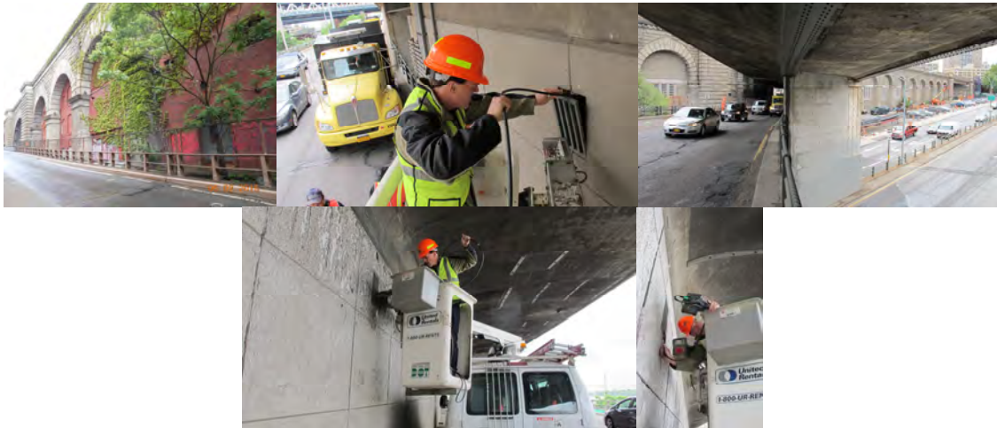
The Brooklyn Bridge Manhattan Approach, Arch Block B Elevation. June 2015: Director of Bridge Management Kevin McAnulty Utilizing a Borescope. June 2015: Director of Bridge Management Kevin McAnulty Inspecting the Brooklyn-Queens Expressway Between Cadman Plaza and Atlantic Avenue With a Borescope. (Credit: Bojidar Yanev)
