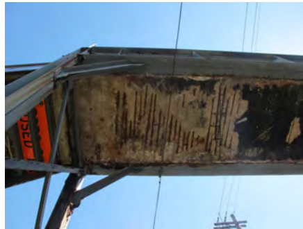
216 th Street Pedestrian Bridge in April 2016: Delaminated Concrete and Detached Exposed Rebar at Span 4 – Deck Underside.
