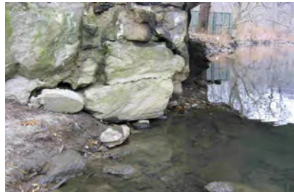
Scour on Pier 2 End Face of Mosholu Parkway Bridge Over Bronx River in 2008. (Credit: NYSDOT)
