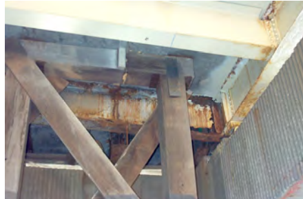
Timber Shoring Supporting a Falling Steel Beam – a Potential Winter Hazard. (Credit: Bojidar Yanev)
