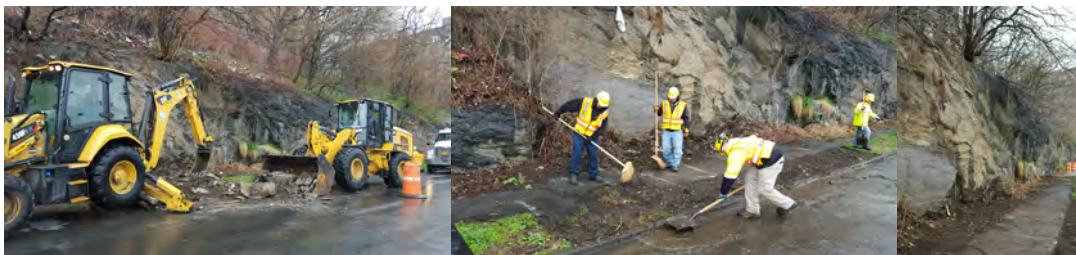
April 2016: The Department of Sanitation Requested Assistance Because Rocks had Slid Down From a Rock Outcropping on the East Side of Sedgwick Avenue Between University Avenue and 167 th Street. Tractor Operator Andrew Mond. Assistant City Highway Repairers James Kelleher, Anthony Angioletti, and James Cummings, and Highway Repairer Jonathan Adorno. Cleared Condition. (Credit: Paul Schwartz)
