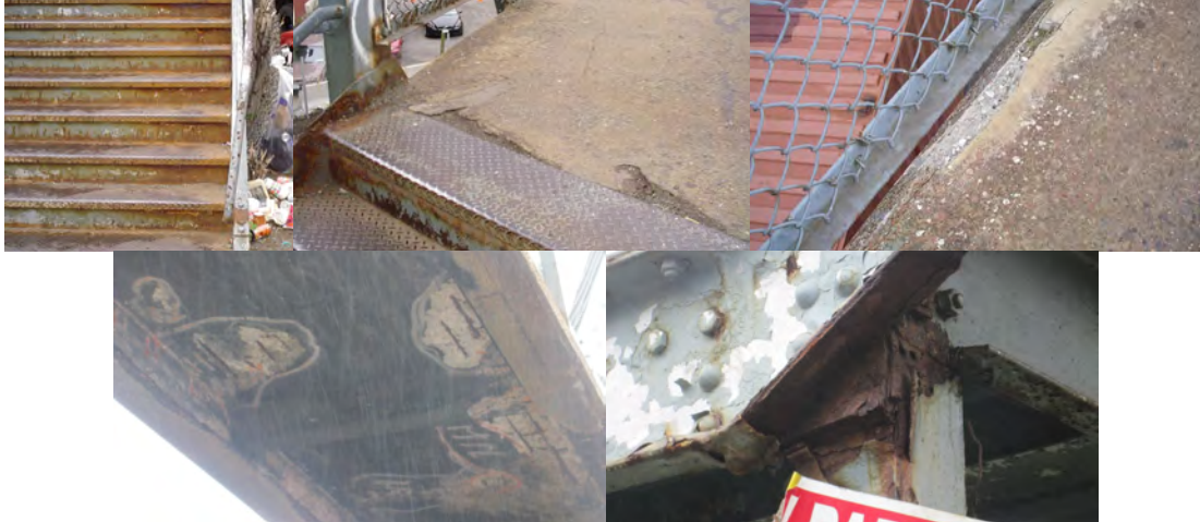
Existing Conditions: Rusted Steps and Damaged Railing. Deteriorated Deck. Spalled Concrete Deck on Main Span. Spalled Concrete – Underside of Deck. Deteriorated Steel.
