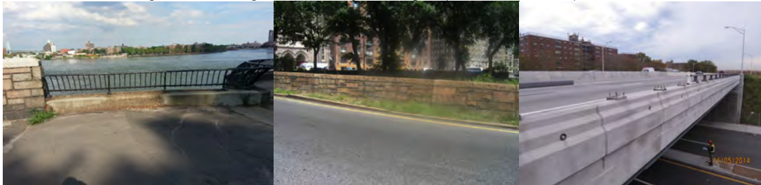
East 81 st to East 90 th Street Promenade over FDR Drive – Right Parapet at Span 45. West 65 th Street Entrance Eastbound over Bride Path West End – View From End of Left Side Parapet. Belt Parkway Bridge over Rockaway Parkway – Right Side Parapet. (Promenade and Rockaway Parkway Credit: NYSDOT)
