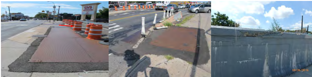
August 2016: Span 2 Left Sidewalk Looking South - Location of the Through Hole. Span 1 Right Sidewalk Looking North. Spalled and Cracked Areas on Top of Span 2 Parapet. (Parapet Credit: NYSDOT)
