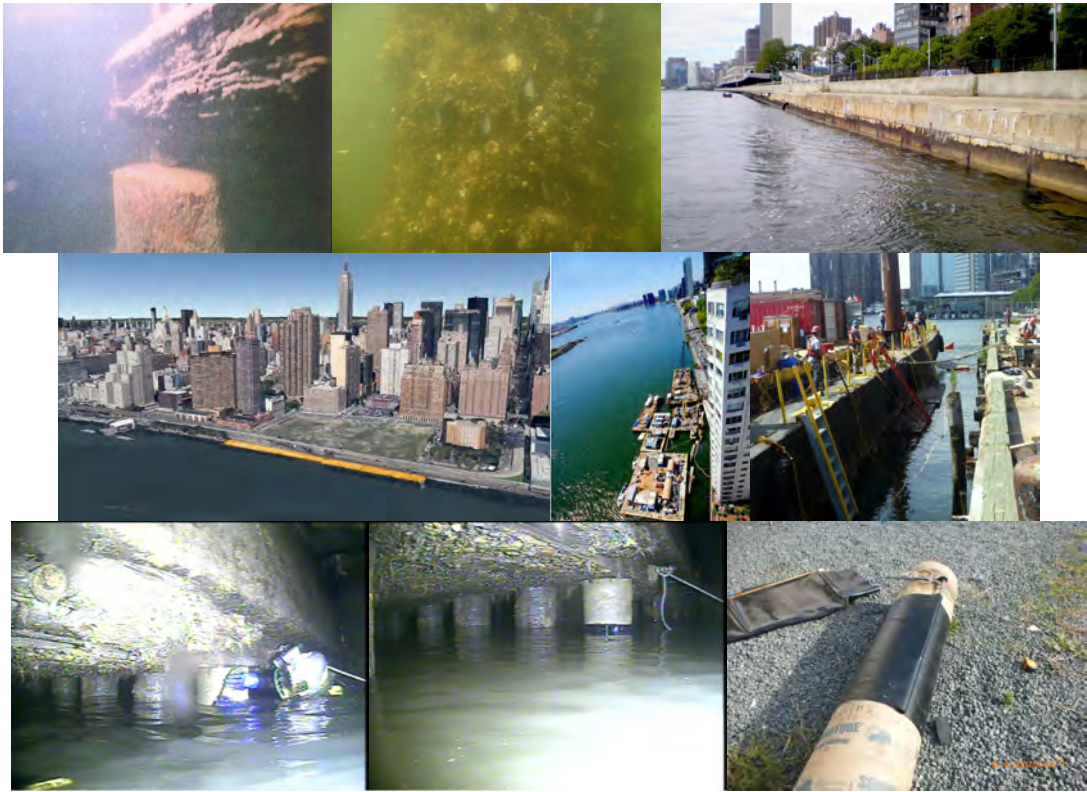
Severe Marine Borer Infestation in Timber Cribbing of Carroll Street Bridge and Moderate Marine Growth Below Waterline on the Ocean Avenue Pedestrian Bridge in 2009. (Credit: NYSDOT) FDR Drive. Location #4 on FDR Drive. Work Barges. Diver Applying Petrolatum Tape. Lower Wrap Section Applied.
