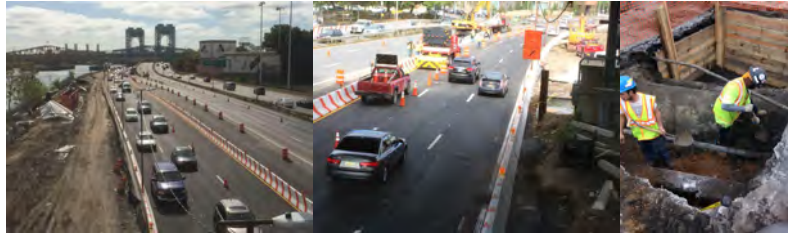
On October 5, 2015, the Temporary Roadway was Opened on the Northbound Harlem River Drive. This enabled the Start of Construction of the New 2 nd Avenue Exit Ramp. December 2015: Test Pit Pier 6.
