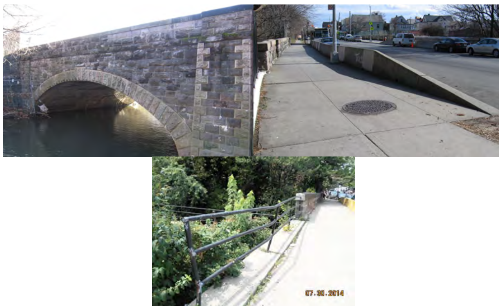
East 180 th Street Bridge over Bronx River. July 2014: Bent Railing at Side Approach. (Railing Credit: NYSDOT)
