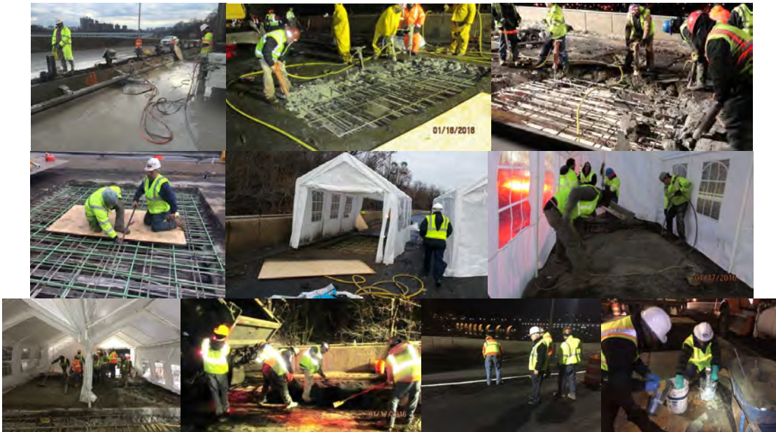
January 2016: Cold Weather Operations. Director of Manhattan and Brooklyn Roadway Bridges Mousa Nazif (White Helmet) Observing the Operations. Testing the Concrete.
