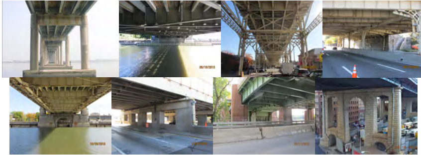
Pier 17 of Rikers Island Bridge. Pier 2 of Broadway Bridge. Piers 12, 33, 37, and 42 of Macombs Dam Bridge. (Credit: NYSDOT) Pier 1 (Looking East) of Hutchinson River Parkway Bridge over Hutchinson River. Pier 6 of Manhattan Bridge. (Credit: NYSDOT)
