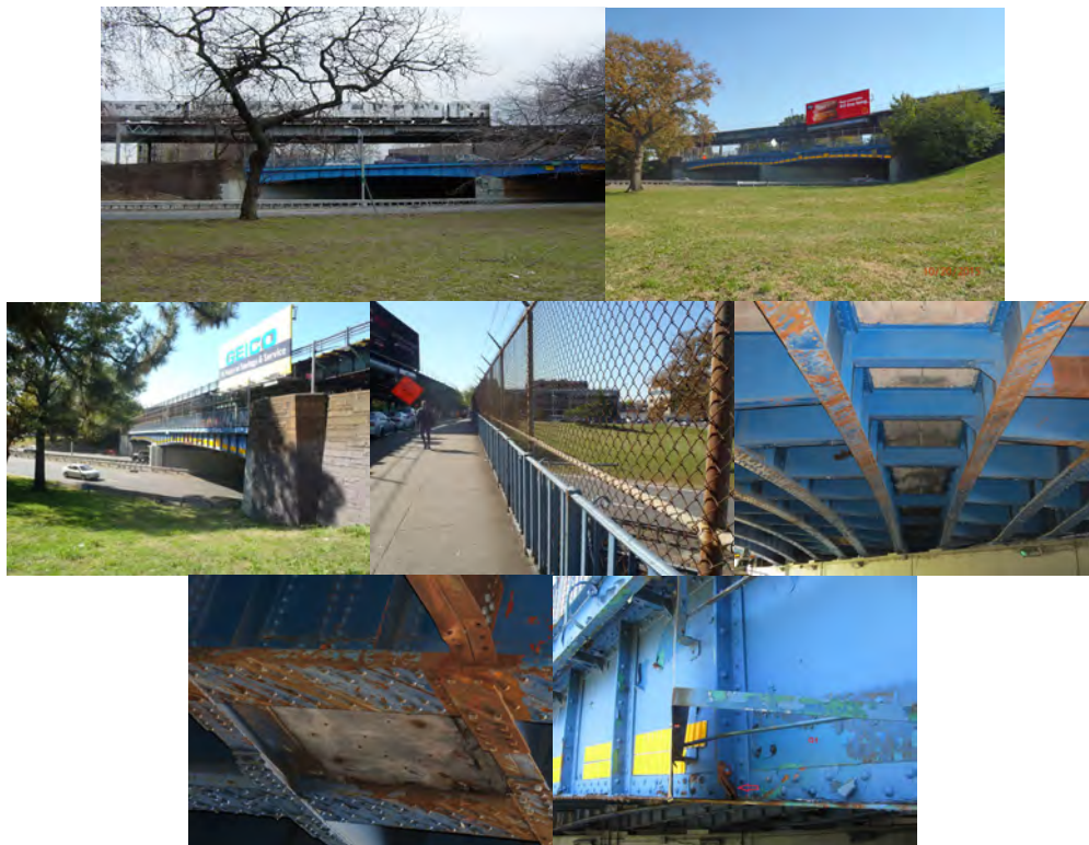
Westchester Avenue Bridge in 2015. June 2016: Underdeck of Span #1 - Deteriorated Deck is Shielded With Timber Planks and Wire Mesh. Bent Stiffener at Span #1.
