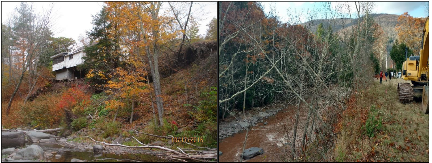
Figure 3.5 Views of a 4.8-acre property before and after demolition of the dwelling. This parcel is on the East Kill in the Town of Jewett and was acquired in 2017 under the NYCFFBO Program.
