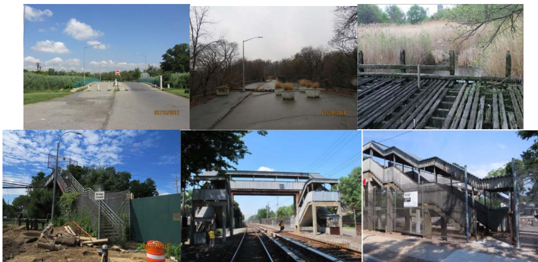
Boathouse Bridge over Aquacade Lake in 2017. (Credit: NYSDOT) Hill Drive Bridge in 2018. Flushing Meadow Park Pedestrian Bridge – (Date Unknown). 216 th Street Pedestrian Bridge in June 2018 - Bridge Closed Sign. Tracy Avenue and Bethel Avenue Pedestrian Bridges in July 2017.
