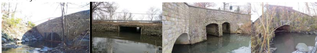
Sweet Brook Road Culvert. Richmond Terrace over Snug Harbor Culvert. Victory Boulevard Culvert. Arthur Kill Road over Clarke Avenue Culvert.
