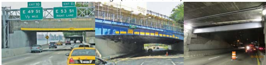
Retro-reflective Material Improves Visibility of These Low Vertical Clearance Bridges: East 60 th Street Bridge over FDR Drive and Westchester Avenue Bridge over Hutchinson River Parkway. Vertical Clearance Beam at Span 53, Southbound Roadway of the Promenade over the FDR Drive. (FDR Credit: NYSDOT)
