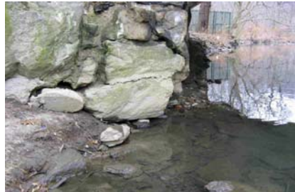
Scour on Pier 2 End Face of Mosholu Parkway Bridge Over Bronx River in 2008. (Credit: NYSDOT)
