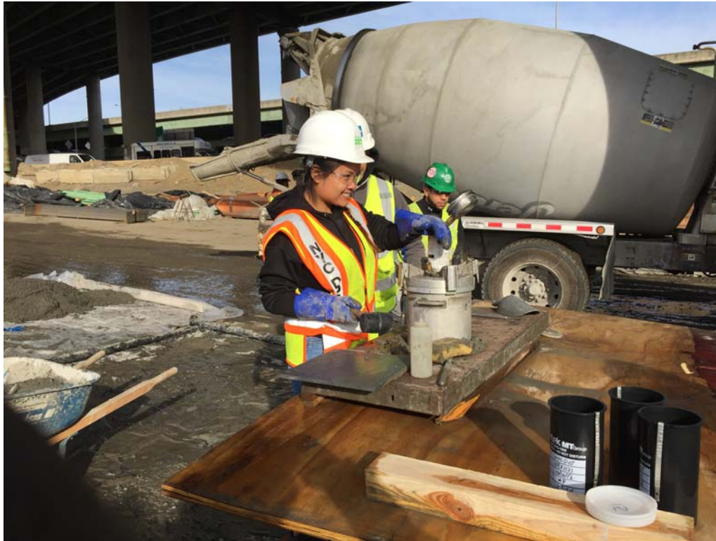
Civil Engineering Intern Phatsia "Patty" Suon Performing an Air Entrainment Test on Concrete Delivered to the Unionport Bridge Construction Project Site. Ms. Suon Joined the Agency in August 2018.
