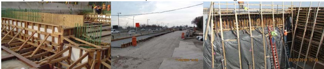
West 252 nd Street Bridge Formwork at the Pier and West Abutment in 2007. Formwork for the Westbound Roadway of the Rockaway Parkway Bridge in 2010. (Rockaway Bridge Credit: Eric Callender) Gerritsen Inlet Bridge in March 2014: Putting up Insulated Forms in Preparation for the Placement of Concrete at the West Abutment Wingwall. The Insulation Helps Protect the Concrete From the Elements and Fluctuating Temperatures During the Curing Period.
