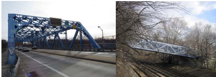
East 174 th Street Truss Bridge over Sheridan Expressway and 204 th Street Pedestrian Bridge over Metro North in 2017.
