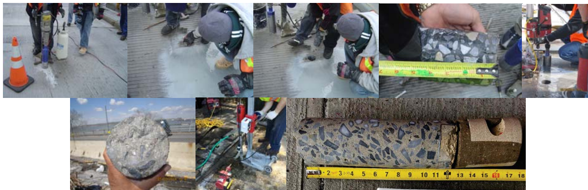
Removing a Core from 252 nd Street Bridge over Henry Hudson Parkway in January 2009. (Credit: Masroor Mahmood) Core Sampling on the Bay Ridge Avenue Bridge in 2014. Utilizing a Coring Machine to Obtain a Concrete Core for Testing in June 2016 from the Westbound BOE over Adams Street.
