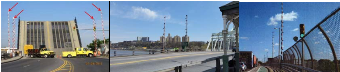
Metropolitan Avenue Bridge over English Kills Warning Gates. (Credit: NYSDOT) West 207 th Street/West Fordham Road Bridge Warning Gate. Greenpoint Avenue Bridge over Newtown Creek Southwest Warning Gate.
