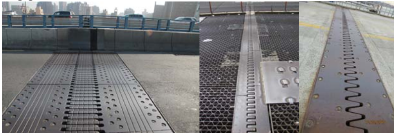
Manhattan Bridge Finger Dam. (Credit: Jagtar Khinda) Unionport Bridge Finger Dam at Span 9 in 2016. Riker's Island Finger Dam.
