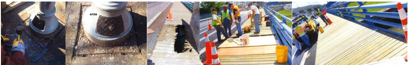
East 14 th Street Bridge Over LIRR Bay Ridge –Ironworkers Fabricated and Installed the Bottom Cover of the Ventilation Post on the Right Sidewalk. Safety Flag: Borden Avenue Bridge over Dutch Kills – Broken Wooden Planks of the Right Sidewalk at Span #1.
