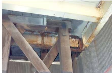
Timber Shoring Supporting a Failing Steel Beam – a Potential Winter Hazard. (Credit: Bojidar Yanev)
