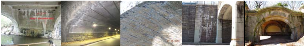
Heavy Efflorescence on End Abutment Stem Wall of Bridge over Dam at Clove Lake in 2014. Efflorescent Stains on the Shielding of Span #1 of the East Drive Bridge over Transverse Road #3 in 2015. Efflorescence, Stalactite Formations, and Scattered Areas of Dampness and Active Water Leakage on the Underside of the Span 3 Arch of the Mosholu Parkway Bridge over the Bronx River in 2016. (Mosholu Credit: NYSDOT) Heavy Efflorescence on Cladding Stones of Crotona Avenue Bridge over Bronx Pelham Parkway in 2016. Efflorescence and Discoloration on the Right Side Fascia of the Meadowport Arch in 2017.
