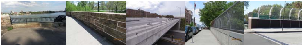
East 81 st to East 90 th Street Promenade over FDR Drive – Right Parapet at Span 45. West 65 th Street Entrance Eastbound over Bridle Path West End – Right Parapet, Looking Southeast. Belt Parkway Bridge over Rockaway Parkway – Right Side Parapet. Congress Street Bridge over Brooklyn-Queens Expressway - Span 1 & 2 Parapet Right side, Looking Northwest. Woodside Avenue Bridge over Brooklyn-Queens Expressway – Left Parapet above Beginning Abutment. (Promenade and Rockaway Parkway Credit: NYSDOT)
