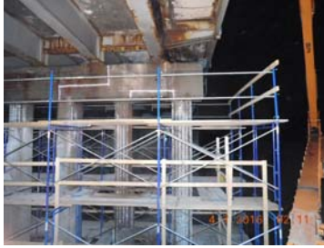
Old Mill Basin Bridge Scaffold Used During Pier Cap and Pier Column Repairs.
