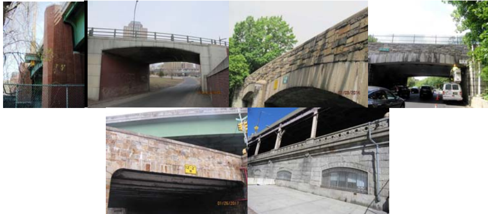
Hutchinson River Parkway Bridge. Brooklyn-Queens Expressway over Ramp to Brooklyn-Queens Expressway (Eastbound). Right Side Fascia on the Bronx Pelham Parkway Bridge. Inspecting the Cladding Stones of the Fascia of Span 1 on West 252 nd Street Bridge over Henry Hudson Parkway. Eliot Avenue Bridge over Queens Boulevard. To Queens from East 59 th Street over First Avenue – Cladding Stones of Span #11 to 13.
