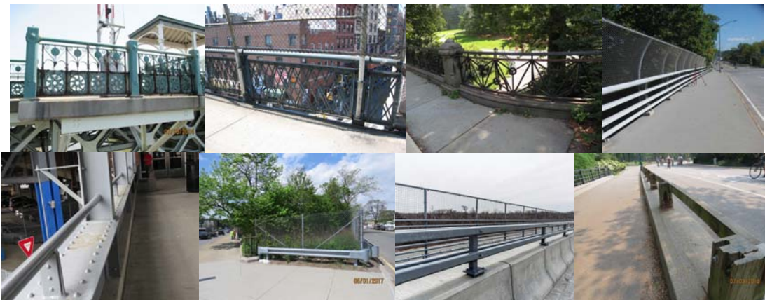
University Heights Bridge Railing. (Credit: NYSDOT) Manhattan Bridge Railing. (Credit: Russell Holcomb) Greywacke Arch Guide Railing in 2017. Northern Boulevard over Cross Island Parkway - Left Sidewalk Railing in 2016. Staten Island Pedestrian Bridge over Parking Lot Exit Roadway - Right Side Railing of Span #2. 14th Avenue Bridge over Cross Island Parkway -End Approach Guide Railing in 2017. New Belt Parkway Bridge over Mill Basin Guide Railing. Center Drive Bridge (Playmates Arch) - Timber Guide Railing Near the Beginning Abutment.
