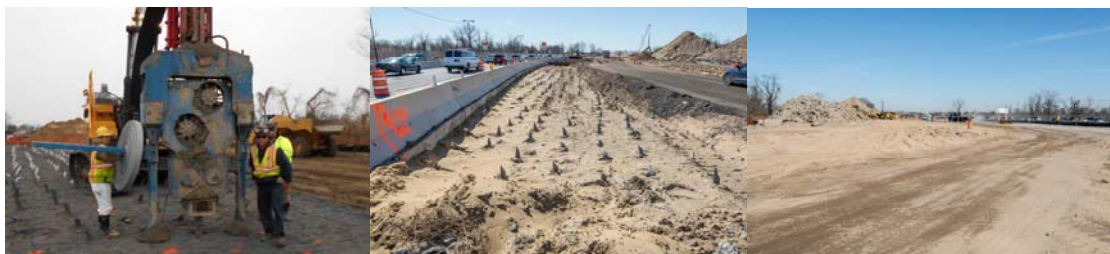
Northwest Quadrant Wick Drains for the New Mill Basin Bridge. Drains Backfilled.
