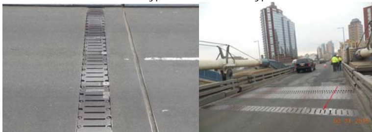
Manhattan Bridge Trench Drain.
