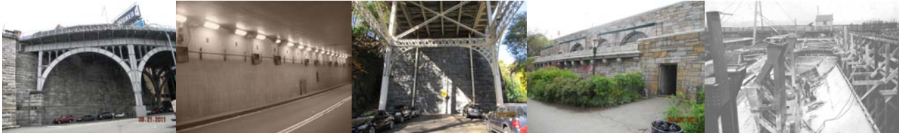
Riverside Drive Viaduct Abutment End. Battery Place Underpass Abutment. Macombs Dam Bridge Beginning Abutment. 79 th Street Traffic Circle Abutment End. (Credit: NYSDOT) Constructing the Abutment of the Eastchester Bridge in 1921.
