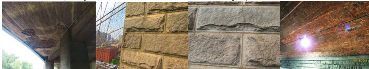
Hollow Sounding And Delaminated Concrete Areas With Exposed Rebars on the Sunrise Highway Bridge Westbound over Laurelton Parkway in 2014. Brooklyn Bridge Tower Stone Delamination in 2016. West Drive over Transverse Road #3 in 2018: Span 1 underside of arch near beginning abutment -Large area of scaled and delaminated brick facing area near begin abutment.
