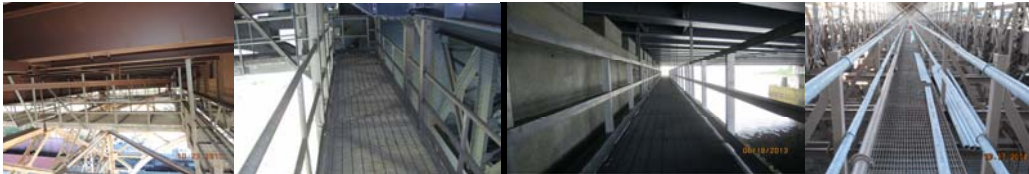
Ed Koch Queensboro Bridge Lower Level Flooring System Catwalk under Span 37. Manhattan Bridge Brooklyn Tower Catwalk. (Credit: NYSDOT) Fresh Creek Catwalk under Deck. Brooklyn Bridge Manhattan Side Catwalk. (Brooklyn Credit: NYSDOT)
