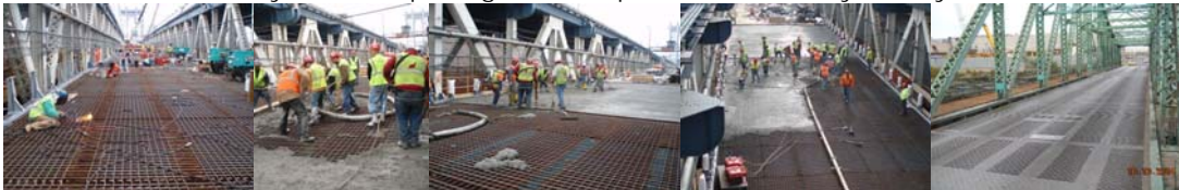
Installation of Full Width Grid Deck Panels on the Manhattan Bridge Lower Roadway in 2006. Pouring the Concrete. Grand Street Deck. (Grand Street Credit: NYSDOT)
