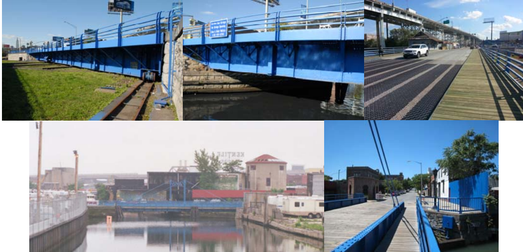
Borden Avenue Bridge. (1 st and 2 nd Credit: Peter Basich, 3 rd : Vadim Sokolovsky) Carroll Street Bridge. (1 st Credit: NYSDOT, 2 nd : Russell Holcomb)
