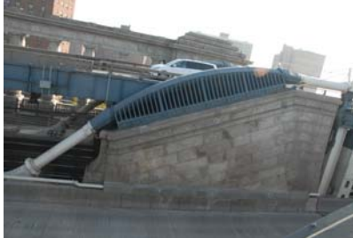
Manhattan Bridge Saddle. (Credit: Jagtar Khinda)
