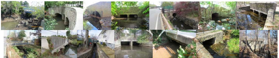
R00032 Seguire Avenue over Purdy Place. R00115 Victory Boulevard over Cloves Lake Park. R00114 Sweet Brook Road over Ridgewood Road. R00103 Aultman Avenue over St. George Road. R00139 De Pew Place over Maguire Avenue. R00105 Arthur Kill Road over Clarke Avenue. R00101 St. Andrews Road over Lighthouse Avenue. R00040 113 Maguire Avenue over Depew Place. R00059 Western Avenue over RR Bridge. R00005 Bidwell Avenue over Columbus Place. R00060 Signs Road over Victory Boulevard. R00062 Kissel Avenue over Snug Harbor Road. R00038 Maguire Avenue over Depew Place. R00036 Amboy Road over Arbutus Avenue.
