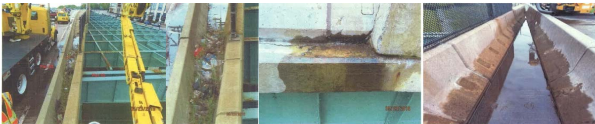
Safety Flag on the Miller Highway in 2018: Debris and Soil Accumulated Between the Jersey Barriers at Pier 55. This Caused Vegetation Growth and Water Ponding and Leaking Onto the Girders. This Leads to Pavement Deterioration and Girder Rust. The Debris and Soil Were Removed.
