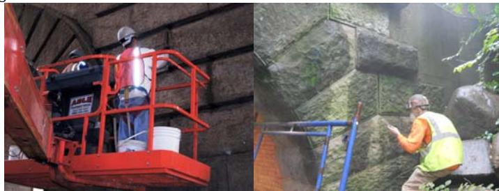
Pointing Joints on the East Face of the Brooklyn Anchorage of the Manhattan Bridge. Pointing the Masonry on the East Drive Bridge (East Wood Arch).
