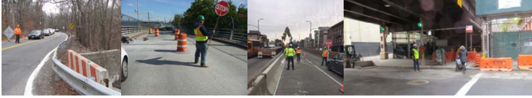
Flagperson at the Rockland Avenue at Manor Road Culvert, Hannah Street Over SIRT, Atlantic Avenue, and at the Queensboro Bridge Ramp to East 62 nd Street From Queens.
