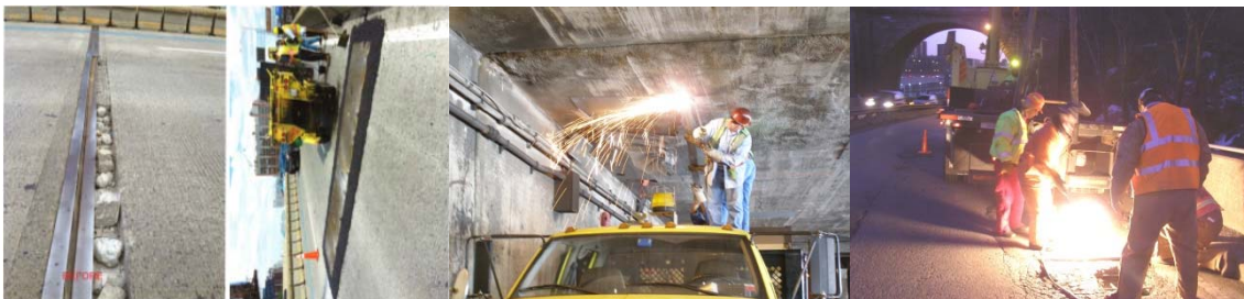
August 2014 PIA Safety Flag: Broken Joint Concrete Header and Steel Armor on the Long Island Expressway over Dutch Kills Creek. The Condition Was Made Safe By Installing Two Steel Plates. PIA Flag (Truck Wedged Under the FDR Drive at Span 41): Removing the Debris. (Credit: Victor Sandoval) PIA Flag Repair (Through Hole) on Harlem River Drive Ramp. (Credit: Bojidar Yanev)
