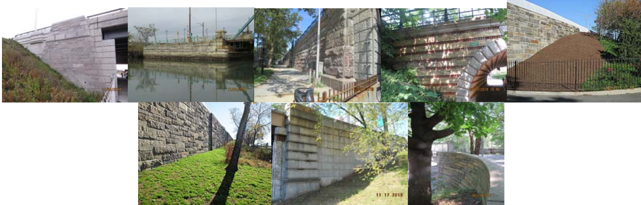
Belt Parkway over Rockaway Parkway, Grand Street, 145 th Street, and Center Drive (Playmates Arch) Wingwalls. (First Four Credit: NYSDOT) Belt Parkway Over Bay Ridge Avenue Bridge Northwest and Southeast Wingwalls in 2015. Brooklyn Bridge North Wingwall in 2016. (Brooklyn Bridge Credit: NYSDOT) Van Cortlandt Equestrian Bridge over Henry Hudson Parkway End Abutment Right Wingwall in 2018.
