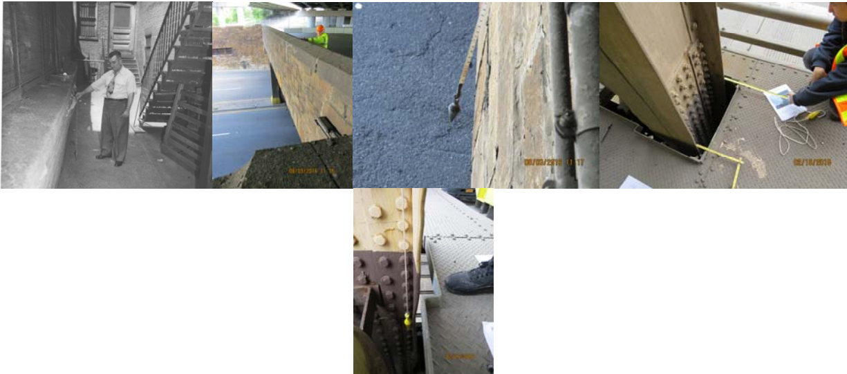
Plumb Bob Demonstrated by Department Engineer in 1951. In Use at Eliot Avenue Bridge over Queens Boulevard in 2016, and the Lower Level of the Ed Koch – Queensboro Bridge in 2018.
