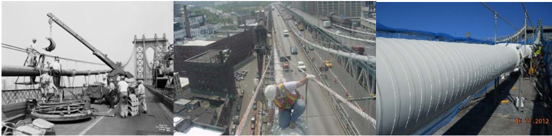
Replacing Cables on the Manhattan Bridge in 1955. (Credit: NYC Records) Inspector on Manhattan Bridge Cable. Cable B. (Credit: NYSDOT)
