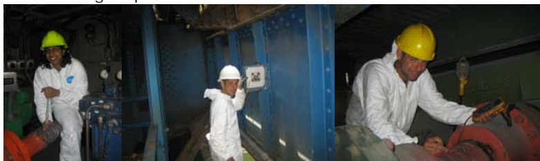
June 2012 - Metropolitan Avenue Bridge. Summer College Intern Nikita Gupta Unsealing the Wire for Strain Gauge Testing. July 2012 - Unionport Bridge. Summer College Intern Kevin Hillery Setting up Inclinometer Calibration. August 2012 - Hunters Point Avenue Bridge. Kevin Hillery Checking Strain Gauge Connections With a Millimeter. (Credit: Vera Ovetskaya)
