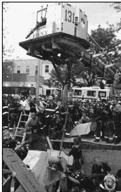
Ladder 131 operates at Brooklyn Box 1326, 145 11th Street, trench cave-in rescue, June 27, 2006. photo by FF Michael Gomez, Squad 288
