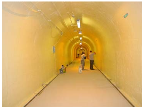
Applying the 2 nd Skid Resistant Coating to the Western Half of the Floor. – the Structure's Lighting Creates the Yellow Tint. (Credit: Thomas Leung)
