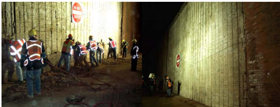
Masonry Crew Removing the Bottom of the Brick Façade. Completed Safety Repair. (Credit: Joseph Saverino)
