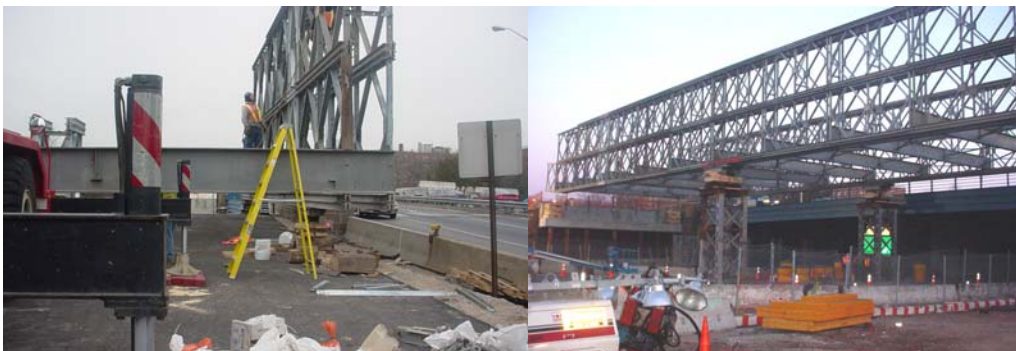
Assembling the Temporary Bridge. Nose of the Temporary Bridge Nearly at the West Abutment. (Credit: Valeriya Remezova)
