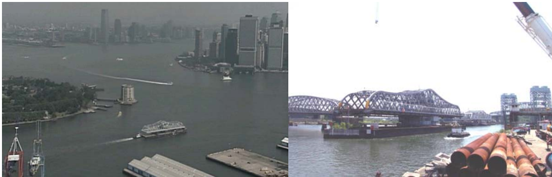
Swing Span Arrival in NYC. Barge Arrival at the Bridge Site. (Site Credit: Bojidar Yanev)
