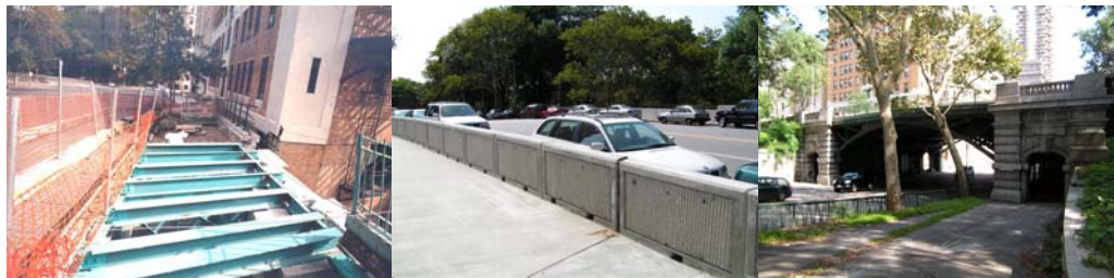
Newly Installed Structural Steel Floor Beams Along the East Sidewalk. Completed Pedestrian Concrete Barrier. Looking East from West 96 th Street at the Newly Rehabilitated Bridge.
