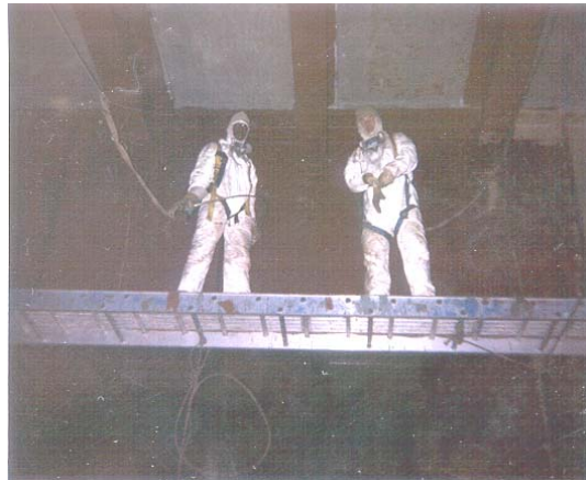
Bridge Painters Goncalo Lima & Milan Radovic at the 11 th Avenue Viaduct. (Credit: Eralene Powell)
