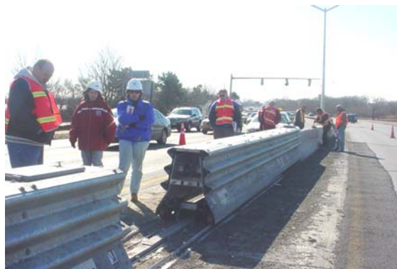
Director of Design-Build/Emergency Contracts Chris Sklavounakis and Beatriz Duran Observing the Demonstration Opening of the Movable Median Barrier. (Credit: Valeriya Remezova)
