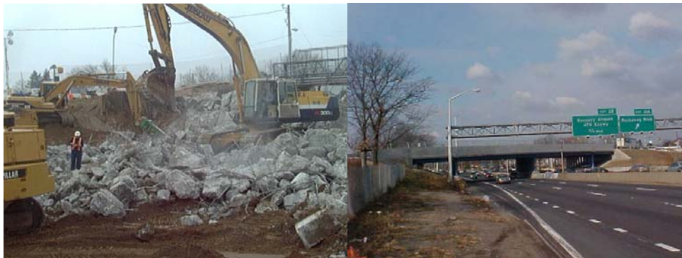
Demolishing the Old Guy Brewer Boulevard Bridge in March 2002 The New Bridge
