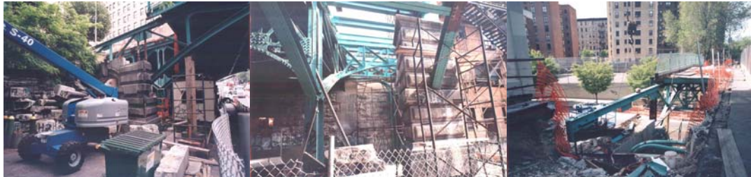
View of the Bridge Under Construction Showing the Marked Granite Stones to be Reinstalled. Newly Installed Structural Steel Members Along the East Sidewalk. View of the New Structural Steel Fascia Girder Being Installed.
