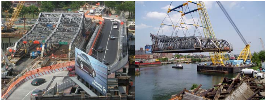
Old Third Avenue Swing Span on Left, New Temporary Bridge on Right. Removing the Manhattan Half of the Old Swing Span. (Credit: Daniel Hom)
