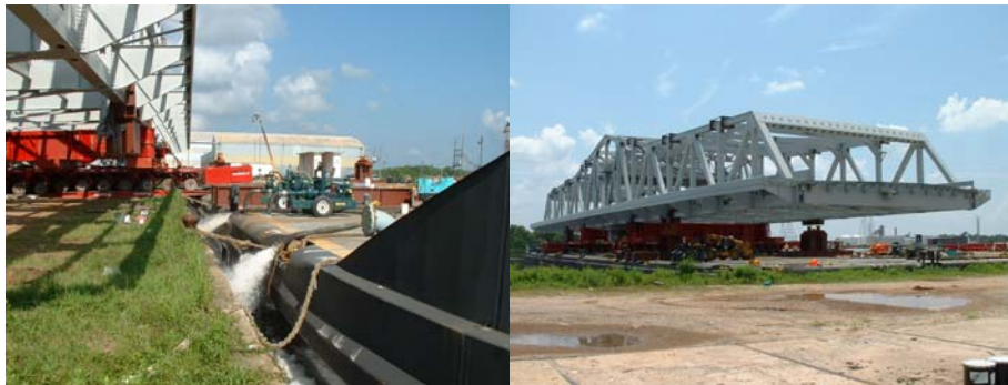
Transfer of New Third Avenue Swing Span From Land to Ocean Barge.
