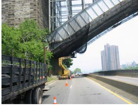
Installing Safety Netting During the Painting of the Washington Bridge. (Credit: Vadim Sokolovsky)
