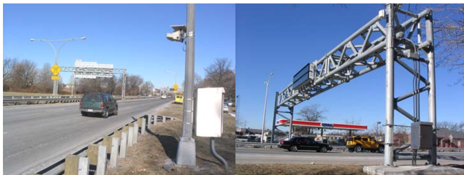
Overheight Sensor on the Northbound Hutchinson River Parkway. Gantry With an Exit Variable Message Sign on the Northbound Hutchinson River Parkway. (Credit: Roly Parroco)
