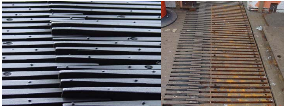
Worn Out Finger Joints on the Bridge. New Finger Joints. (Credit: Nasir Khanzada)
