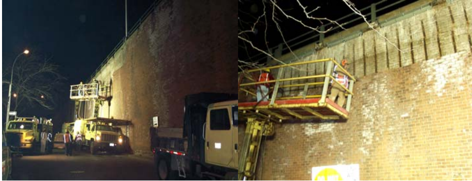
Bricklayers Ignazio Trapani & Savatore Romano on the Truck Platform Removing the Brick Façade. Cement Masons John Padovano & Thomas Valentino Removing Bricks. (Credit: Joseph Saverino)
