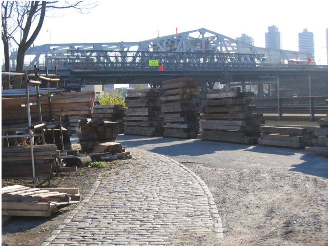
View From the Bronx of the Third Avenue Temporary Bridge and New Swing Span in November 2004. (Credit: Michele N. Vulcan)
