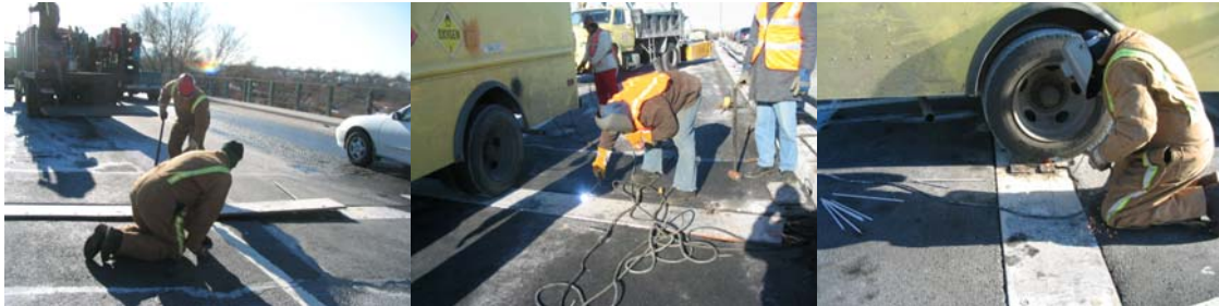
Division Ironworkers at the Belt Parkway Bridge over Paerdegat Basin. (Credit: Gholamali Mozaffari)
