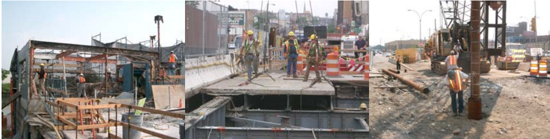
Looking East at the Demolition of the Bridge Operator House. Looking West at the Removal of the Northwest Grid Deck. Looking East at the Driving of a Test Pile.
