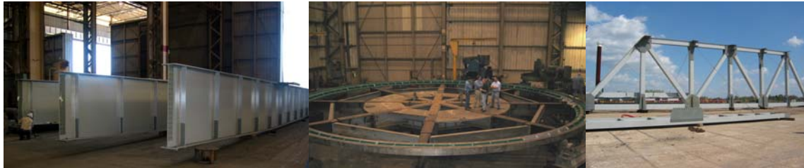
Touching up the Painting of the Intermediate Floorbeams. Track and Rack Assembly on Rotary Table Prior to Tooth Cutting. Northwest Truss Section for the New Third Avenue Bridge Swing Span (Credit: Rahul Shah)
