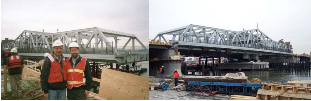
Engineer-in-Charge Daniel Hom and Deputy Chief Engineer Russell Holcomb at the Float-in. New Swing Span After the Float-in. (Span Credit: Keith Burrowes)
