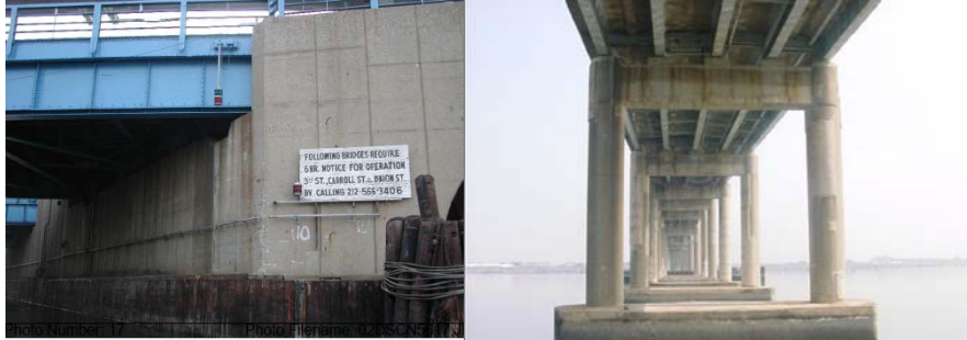
Left Side of Pier 1 of Hamilton Avenue Bridge. Pier 17 of Rikers Island Bridge. (Credit: NYSDOT)
