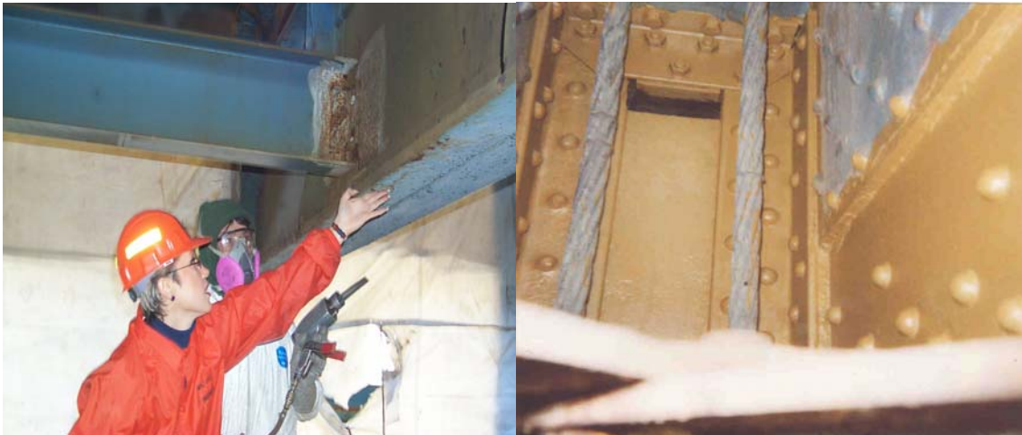
Spot Cleaning Before Painting on the Williamsburg Bridge. Primer Coating on the Williamsburg Bridge.
