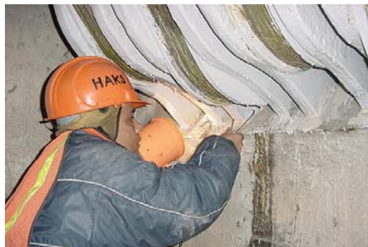
Inspecting the Eyebars in the Brooklyn Anchorage of the Manhattan Bridge. (Credit: NYSDOT)
