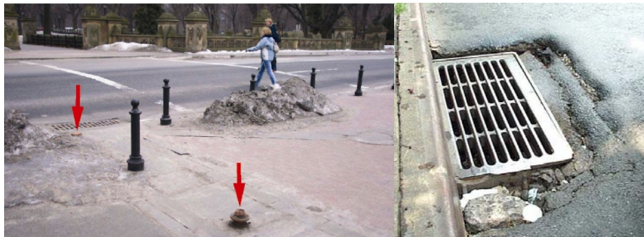
72 nd Street Cross drive Near Concert Grounds – The Posts Were Missing, Leaving the Bases Protruding Above the Sidewalk. This was a Tripping Hazard. Gun Hill Road over Bronx Boulevard – the Asphalt Surrounding the Catch Basin Had Settled, Causing the Grating to Deflect Under Heavy Traffic Loads. This was a Safety Hazard to Vehicles. (Description & Credit: NYSDOT)
