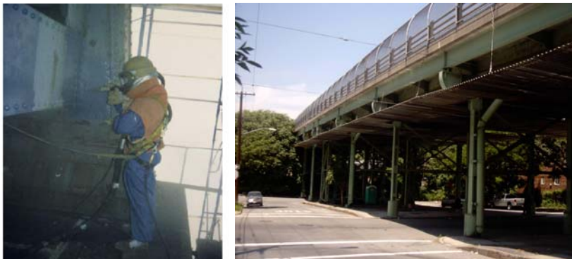
Abrasive Blasting. Platform Installed for Painting of the East 241 st Street Bridge.
