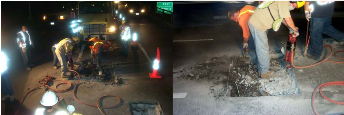
Masonry Crews and Highway Repairers Repairing Recurrent Potholes on the Eastbound Brooklyn-Queens Expressway, Just Past the Middagh Street Underpass. Break-Out and Removal of the Old Asphalt Roadway and Concrete Deck. (Credit: Anthony Napolitano)
