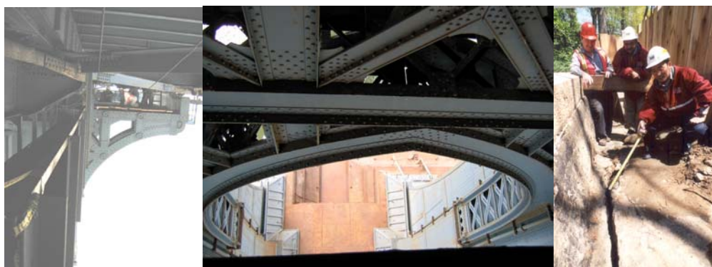
Flag Engineers Inspecting a Red Flag (Floor Beam Web) on the Tower Structure of the Manhattan Bridge. Closeup of the Location. (Credit: Bojidar Yanev) Flag Engineers Inspecting a Red Flag on the Central Drive Bridge over Transverse Road #1-- the West Fascia Had a Long Crack Running From the South Abutment Wall to the North Abutment Wall. (Credit: Peter Basich)
