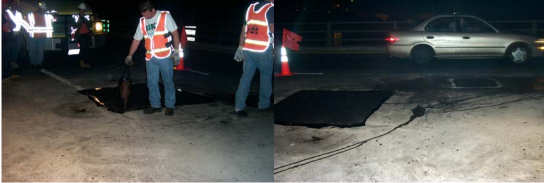
Sealing the Edges of the Cutout With Asphalt Cement to Prevent Water From Seeping In. Closeup of Part of the Completed Concrete Deck Repair on the Eastbound BQE. (Credit: Anthony Napolitano)
