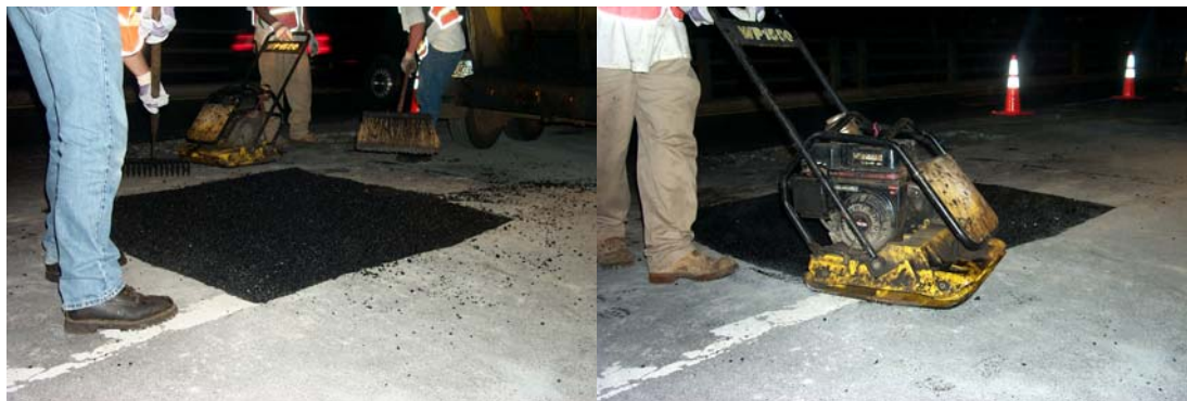
Rolling and Tamping the Asphalt on the Eastbound BQE. (Credit: Anthony Napolitano)
