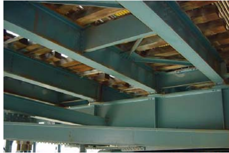
South Transit Floorbeams, Stringers, and Bracing Members on the Manhattan Bridge. (Credit: NYSDOT)
