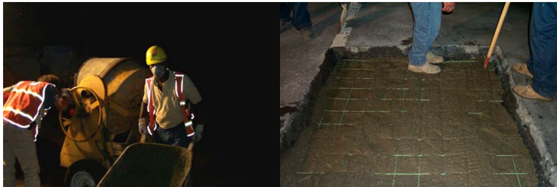
Installing New Concrete With Rebar in the Cutout on the Eastbound BQE. (Credit: Anthony Napolitano)
