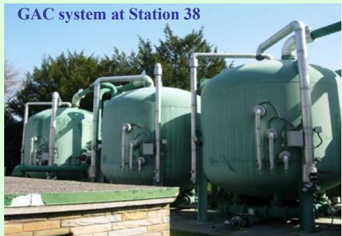
GAC system at Station 38
