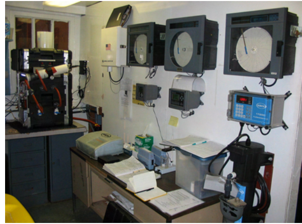
Figure 2.1 Continuous monitoring instrumentation at Kensico Reservoir (Catskill Lower Effluent Chamber).
