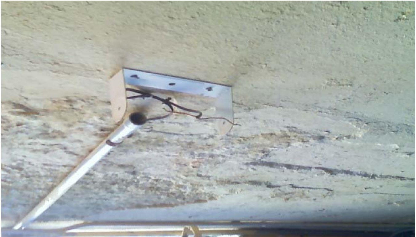
Lasker Rink – Picture # 1: Inoperable Ceiling Fixture and Peeling Paint
