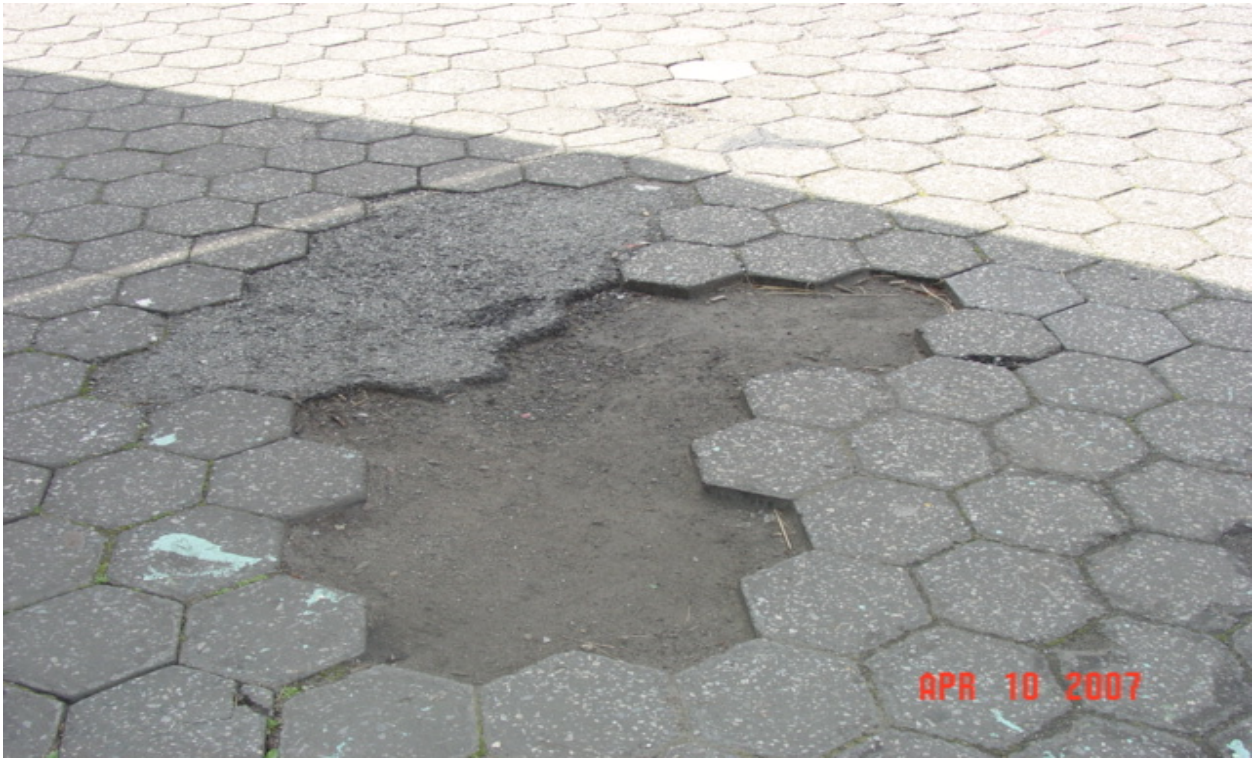
Lasker Rink – Picture # 3: Missing Flooring Tiles on the Upper Deck
