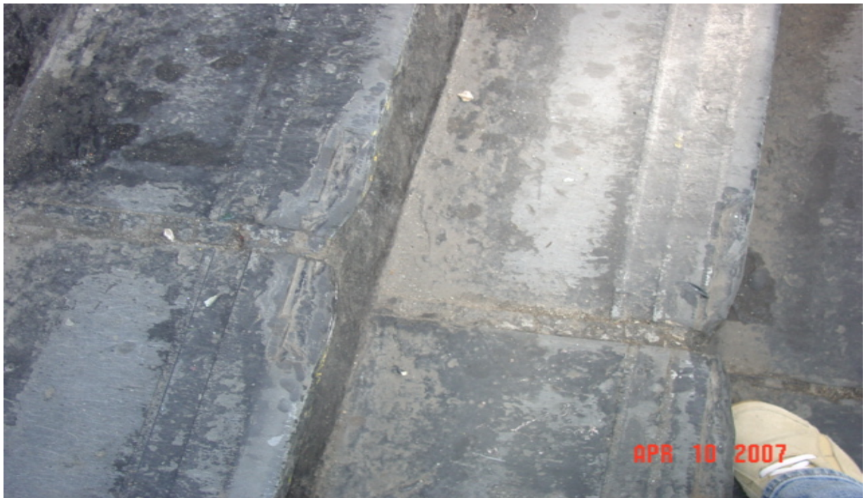
Lasker Rink – Picture # 6: Damaged Treads on Staircase
