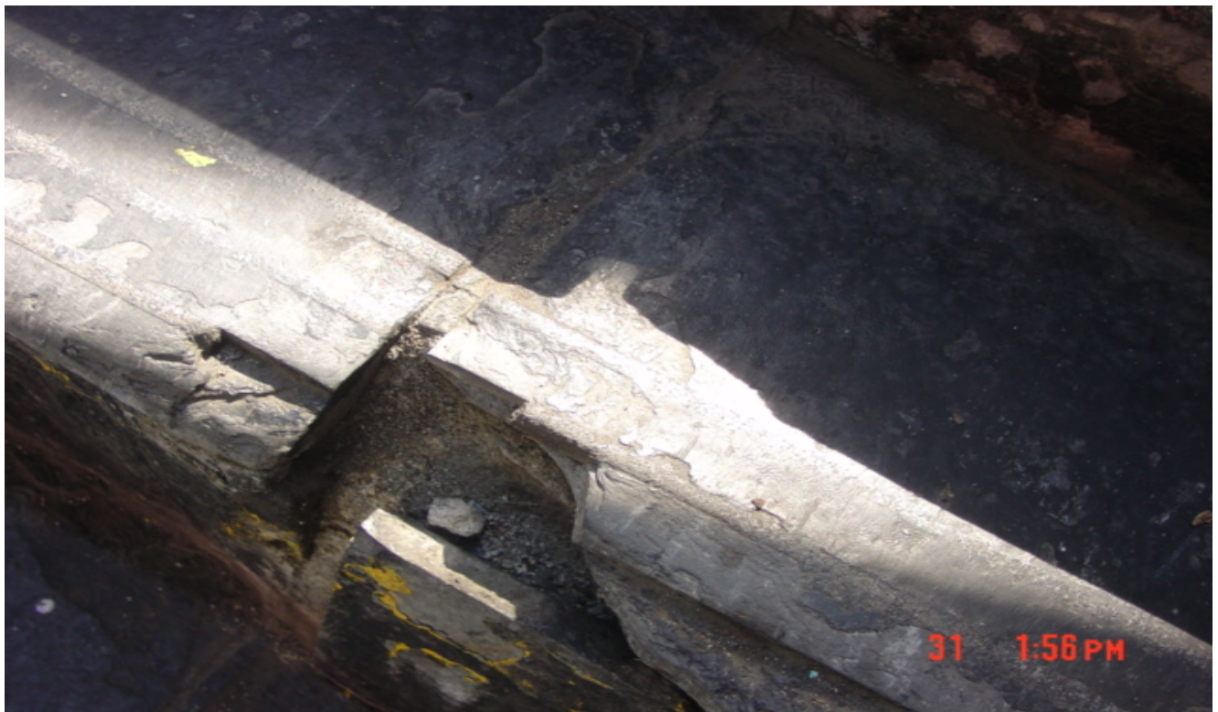
Lasker Rink. Picture # 2: Deteriorated stairs at entry gate pavilion.
