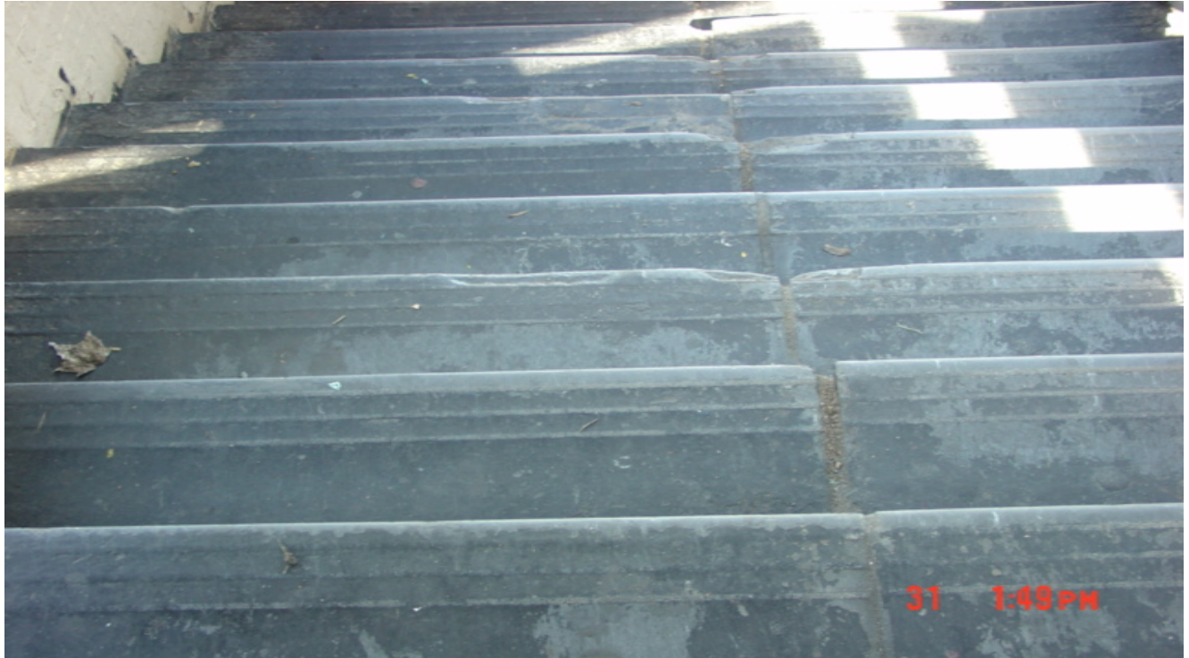
Lasker Rink. Picture # 1: Deteriorated stairs at entry gate pavilion.
