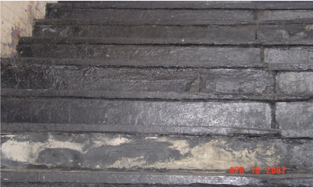
Lasker Rink – Picture # 8: Damaged Treads and Risers on Stair Case
