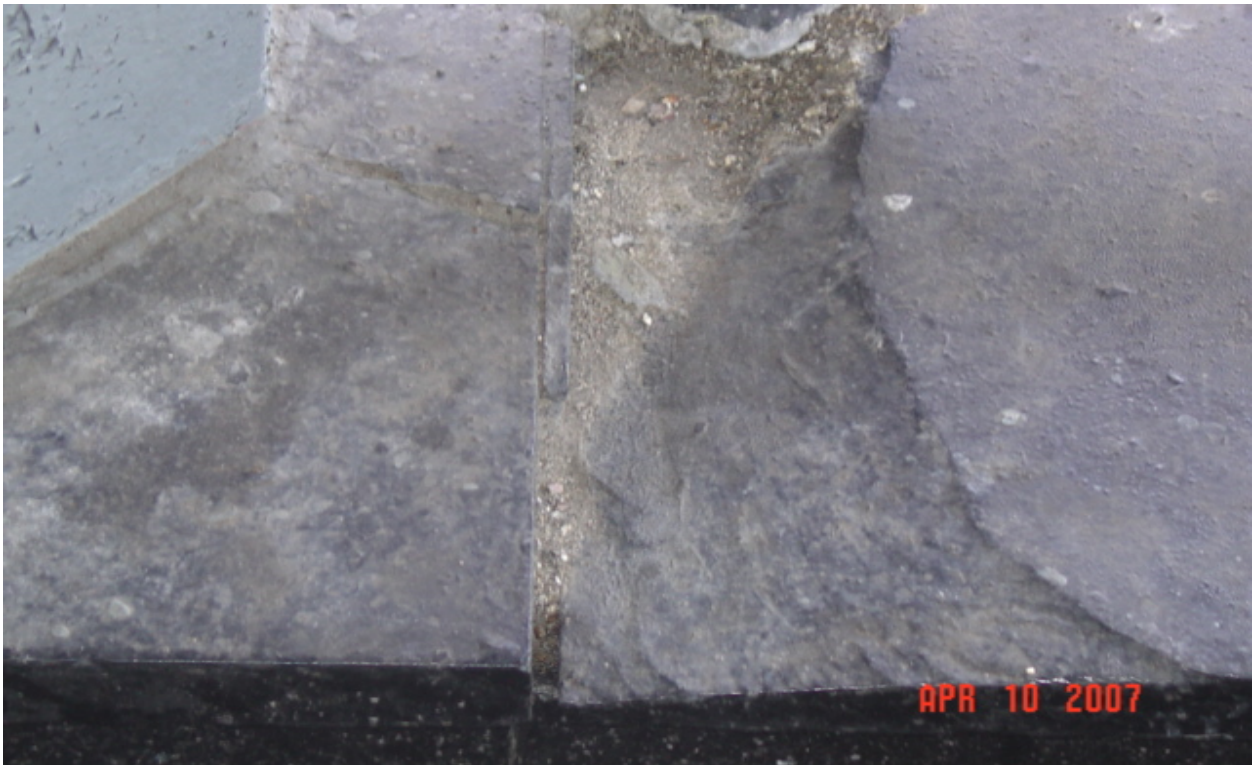
Lasker Rink – Picture # 4: Deteriorated Floor on the Upper Deck
