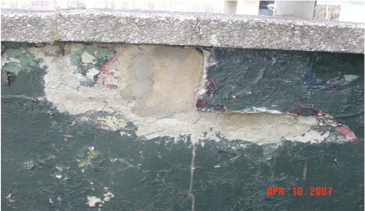
Lasker Rink – Picture # 1: Damaged Parapet Wall
