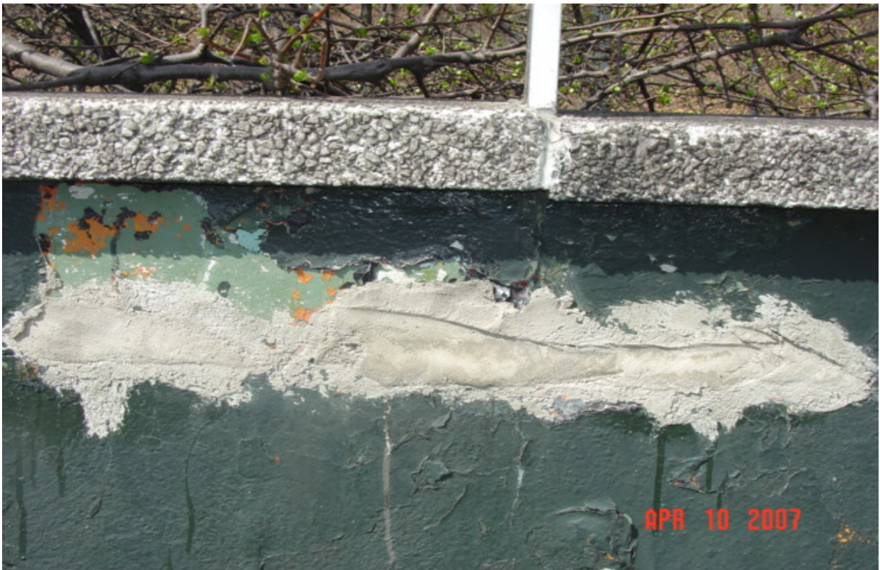
Lasker Rink – Picture # 2: Damaged Parapet Wall
