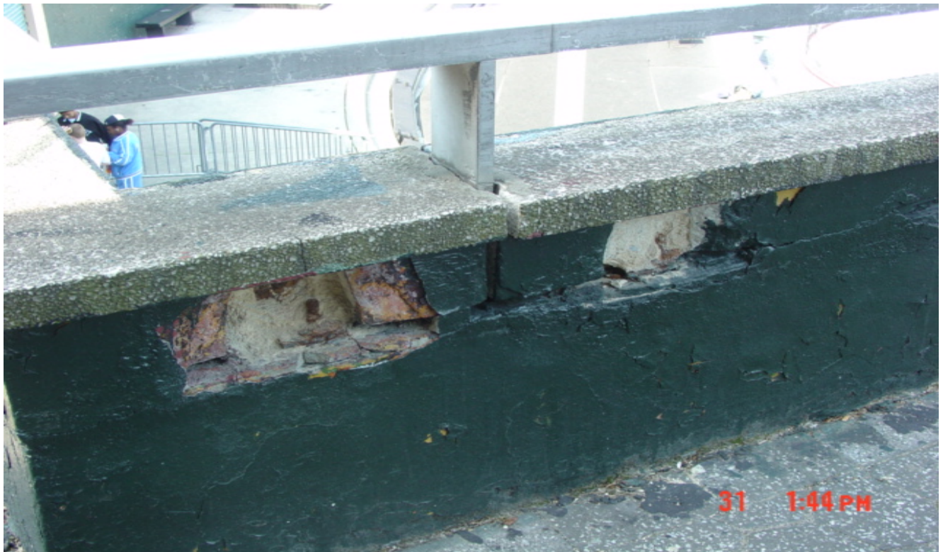
Lasker Rink. Picture # 4: Damaged parapet wall.
