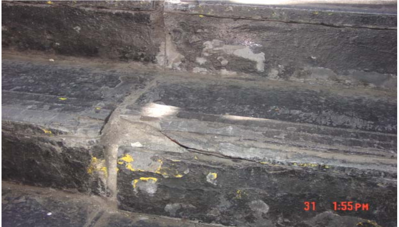
Lasker Rink. Picture # 3: Deteriorated stairs at entry gate pavilion.
