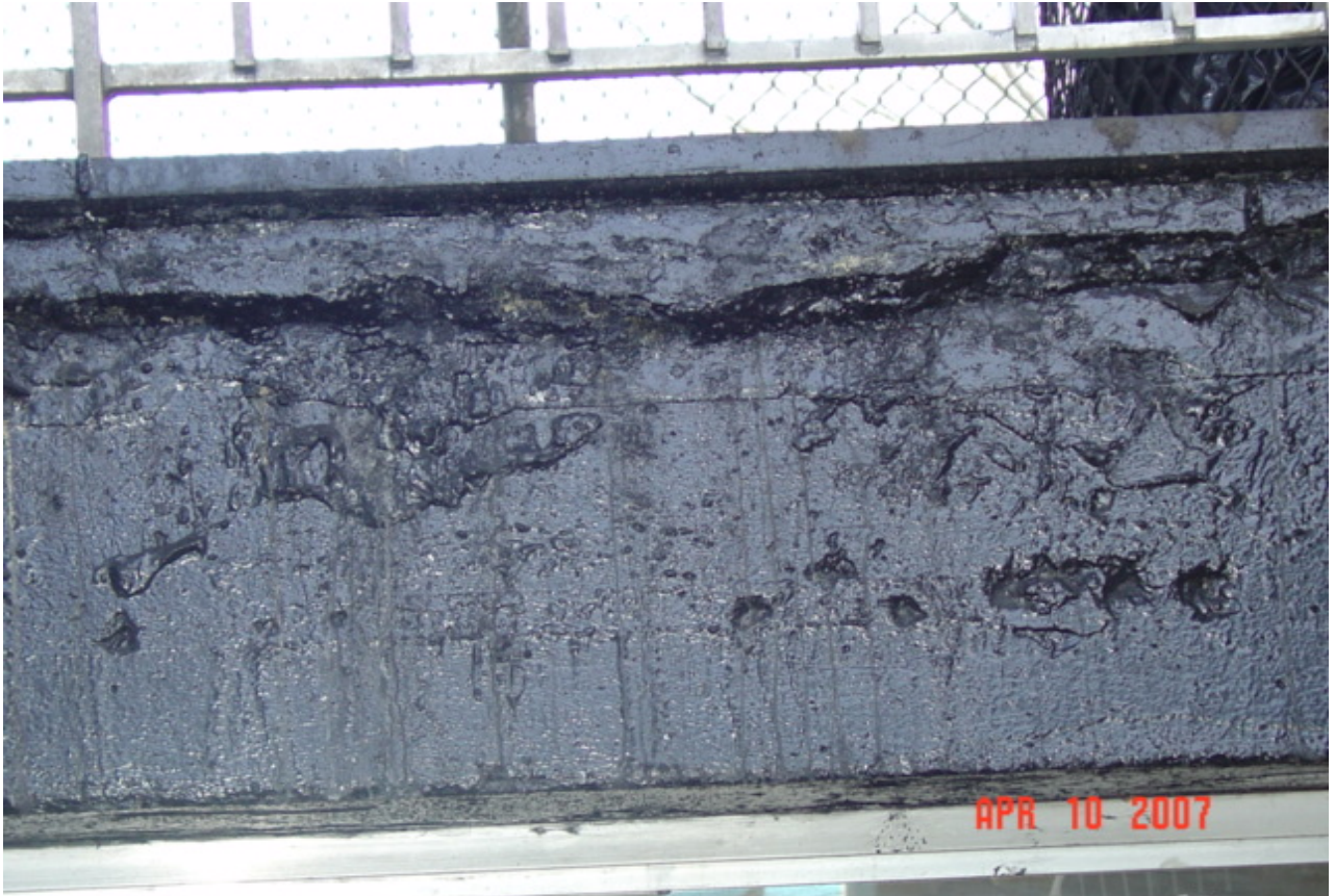
Lasker Rink – Picture # 5: Chipping/Separation of the Concrete Surface on the Upper Deck
