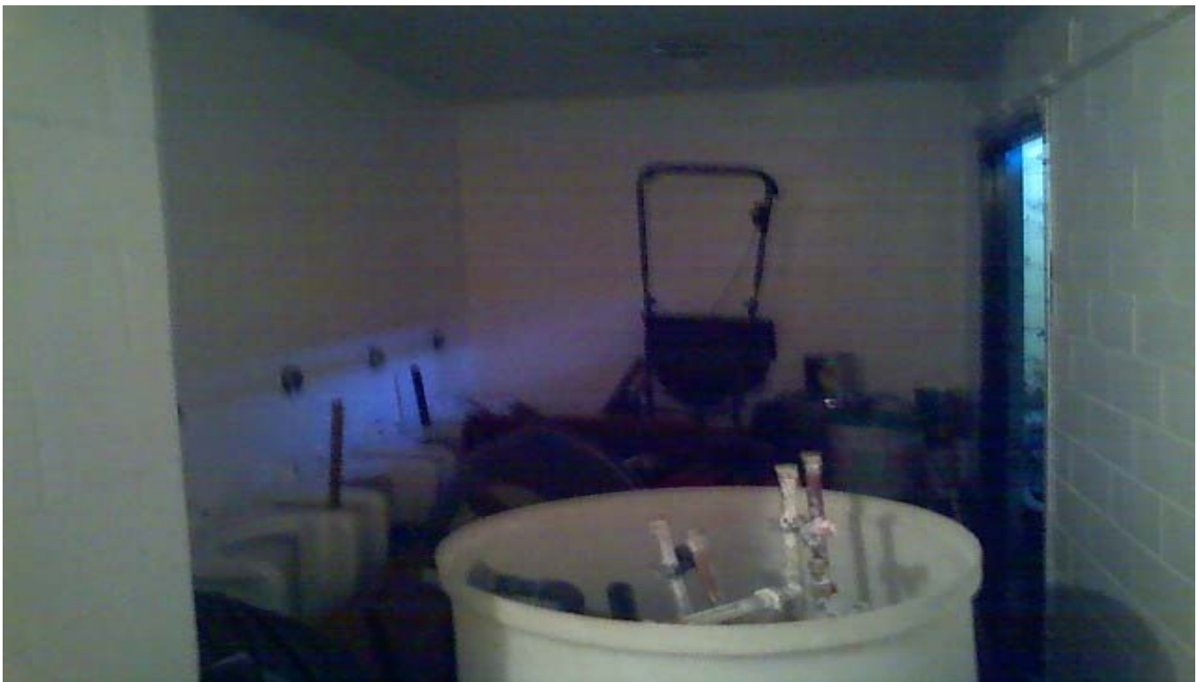
Lasker Rink – Picture # 4: Inoperable Restroom Facilities
