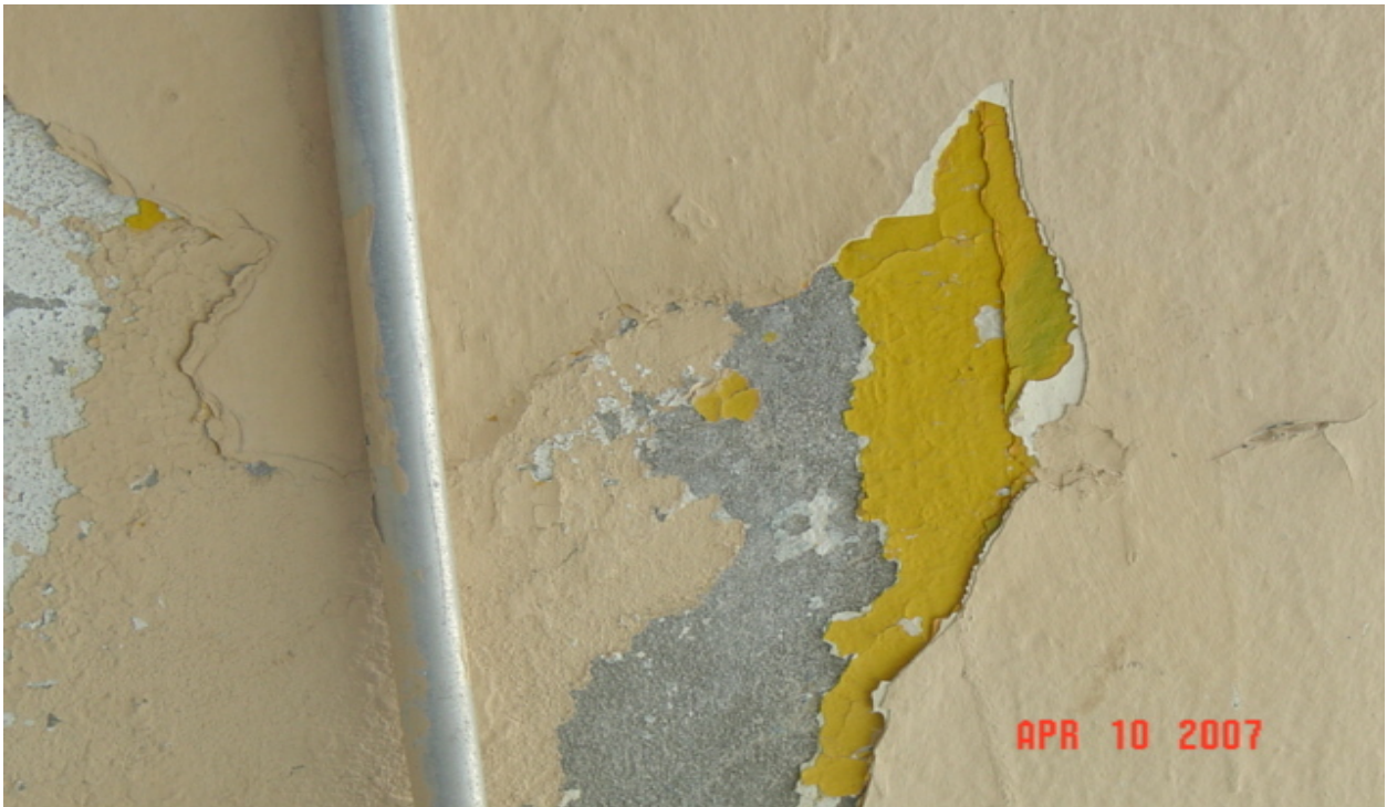
Lasker Rink – Picture # 10: Peeling Paint on the Interior Wall
