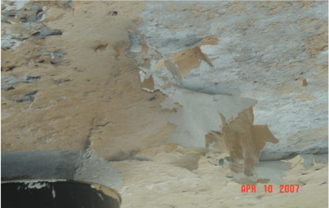
Lasker Rink – Picture # 9: Peeling Paint on the Ceiling Below Upper Deck
