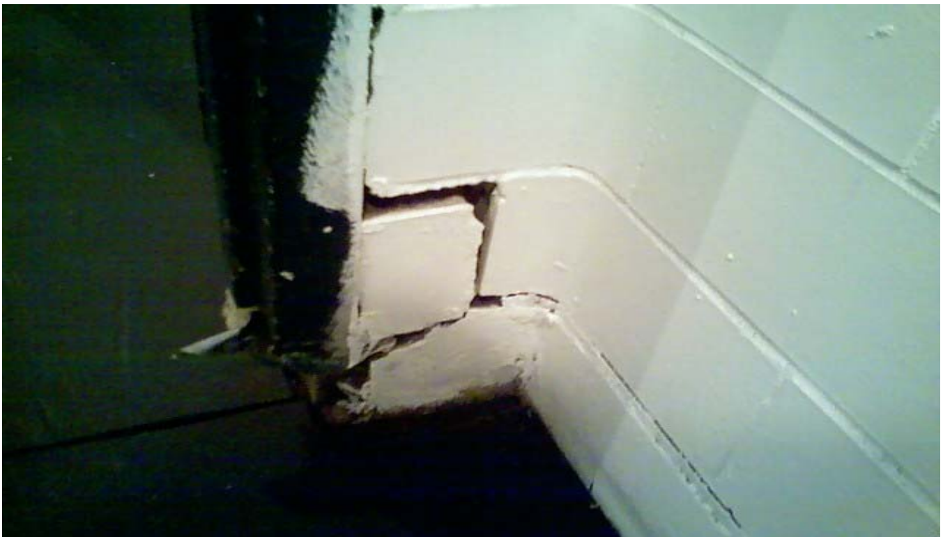
Lasker Rink – Picture # 2: Cracked Restroom Wall
