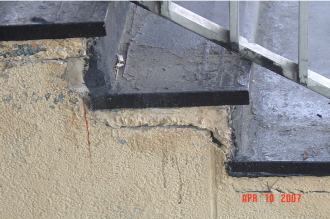
Lasker Rink – Picture # 7: Concrete Separation Below Stair Case Treads
