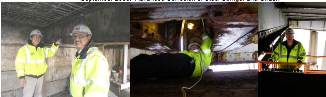
Assistant Civil Engineer Andrew Hoang and Civil Engineer Rajendra Pandya Measuring the Section Loss of the Bottom Flange of A Floor Beam, Utilizing a Digital Caliper. Executive Director of Bridge Preventive Maintenance and Repair Thomas Whitehouse Inspecting a Red Flag on a Girder Floor Beam at the Belt Parkway Bridge over Gerritsen Inlet. Mr. Whitehouse Operating a Zoomboom. (Gerritsen Credit: Steve Havemann)
