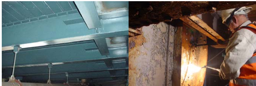
Stringers on the Manhattan Bridge. (Credit: NYSDOT) Bridge Repairer & Riveter Joseph Antony Repairing a Red-Flagged Stringer on the Bridge. (Credit: Hany Soliman)
