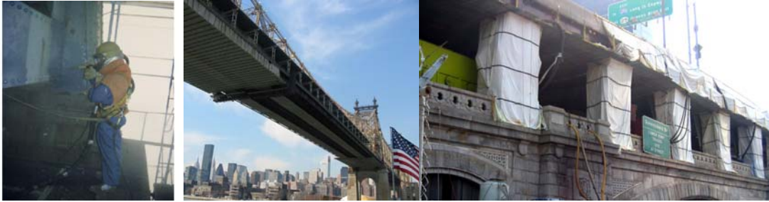
Abrasive Blasting. Platform Installed for Painting of the Queensboro Bridge (Credit: Vadim Sokolovsky) Containment on Queensboro Bridge Manhattan Ramp. (Credit: Peter Basich)
