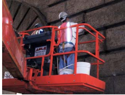
Pointing Joints on the East Face of the Brooklyn Anchorage of the Manhattan Bridge.
