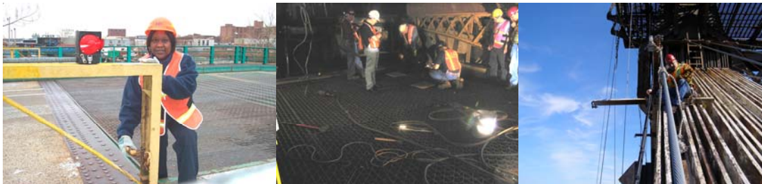
Bridge Operator Mary Harrigan at the Union Street Bridge. (Credit: Adal Maldonado) Bridge Repairer/Riveters Repairing the Willis Avenue Bridge Grating. (Credit: Reza Taheri) Supervisor Electrician Ben Cipriano Repairing a Damaged Electrical Cable on The Queensboro Bridge in March 2007. (Credit: Bala Nair)
