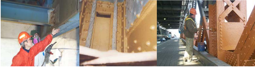
Spot Cleaning Before Painting on the Williamsburg Bridge. Primer Coating on the Williamsburg Bridge. Salt Splash Painting on the Williamsburg Bridge. (Salt Splash Credit: Fouad Althaibani)
