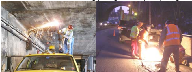
PIA Flag (Truck Wedged Under the FDR Drive at Span 41): Removing the Debris. (Credit: Victor Sandoval) PIA Flag Repair (Through Hole) on Harlem River Drive Ramp. (Credit: Bojidar Yanev)
