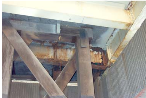
Timber Shoring Supporting a Failing Steel Beam – a Potential Winter Hazard. (Credit: Bojidar Yanev)
