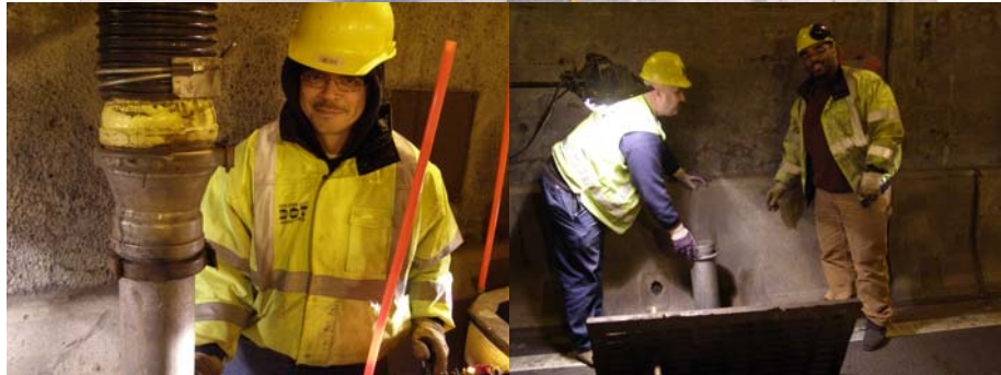
Cleaning Catch Basins on the Manhattan Bridge. Drain Crew: Highway Repairer Anthony Irizarry, Supervisor Highway repairer Michael Parise, and Assistant City Highway Repairer Giovanni Caballero. (Crew Credit: James Campbell)
