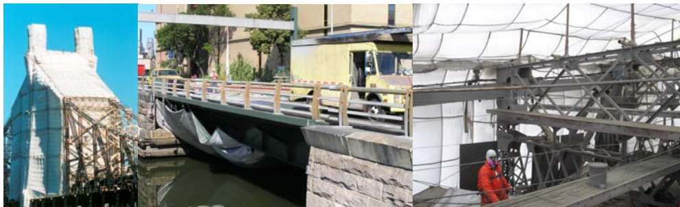
2005: Queensboro Bridge Containment. (Credit: Peter Basich) 2005: Preventing Paint From Falling Into the Dutch Kills under the Hunters Point Avenue Bridge. (Credit: Sergiy Parayev) Working Inside the Queensboro Bridge Containment.
