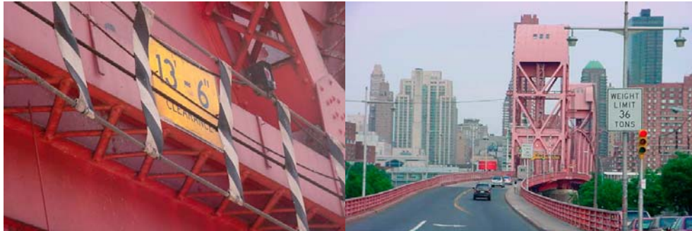
Roosevelt Island Bridge Vertical Clearance Restriction and Posted Weight Signs (Credit: NYSDOT)
