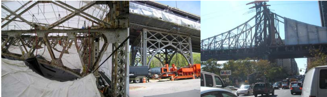
Inside the Queensboro Bridge Containment. 2005: Roadway Containment. (Roadway Credit: Michele N. Vulcan) 2006: Containment Above the Upper Roadway.
