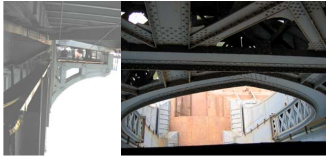
Flag Engineers Inspecting a Red Flag (Floor Beam Web) on the Tower Structure of the Manhattan Bridge. Closeup of the Location. (Credit: Bojidar Yanev)
