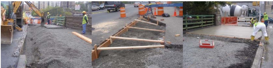
Sidewalk Repairs at East 174 th Street Over The Ramp to The Cross Island Parkway. (Credit: Reza Taheri)
