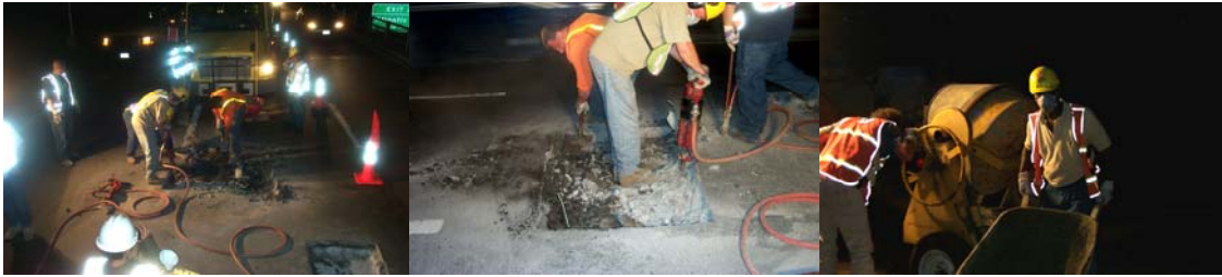
2005: Masonry Crews and Highway Repairers Repairing Recurrent Potholes on the Eastbound Brooklyn-Queens Expressway, Just Past the Middagh Street Underpass. Break-Out and Removal of the Old Asphalt Roadway and Concrete Deck. Installing New Concrete With Rebar in the Cutout on the Eastbound BQE. (Credit: Anthony Napolitano)
