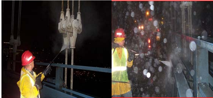
Power Washing the Corrosive Deicing Solvents Within the Range of the Roadway Splash Zone on The Manhattan Bridge in October 2007. Particular Attention is Directed to Cleaning the Gusset Plate. (Credit: Albert Hong)
